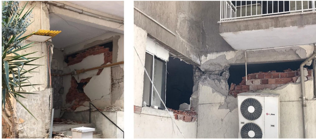
Figure 36. Heavy damage in a RC frame building with URM infills (Credit: Ozgur Ozcelik).
