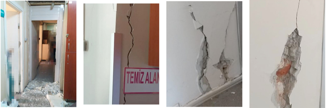
Figure 22. Fallen debris and damage observed in the interior walls of the Buca Seyfi Demirsoy hospital in Izmir (Haberek, 2020; Oda TV, 2020).
