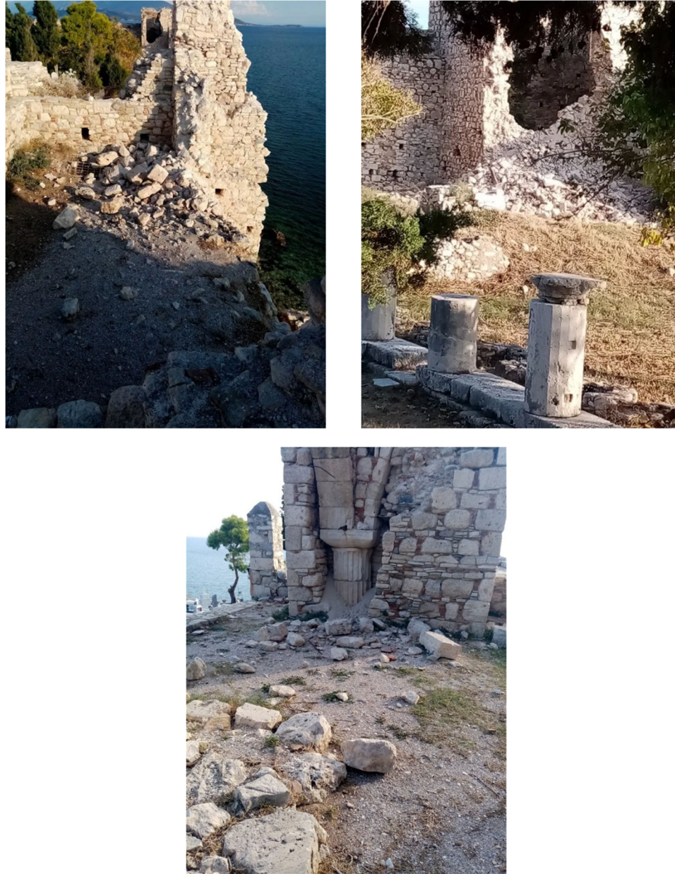
Figure 28. Damage to the wall of the Castle of Lykourgos Logothetis in Pythagorion (Dikastiko, 2020; Protothema, 2020b).
