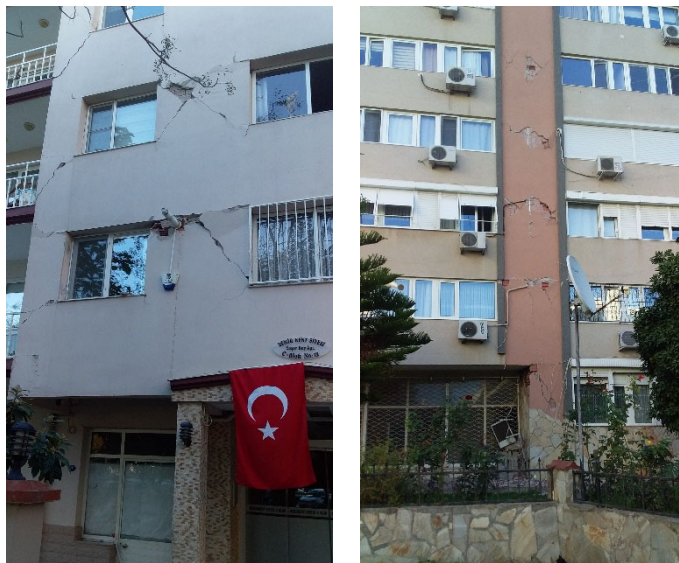
Figure 37. Diagonal cracks in exterior infill walls (Credit: Mauricio Morales-Beltran).
