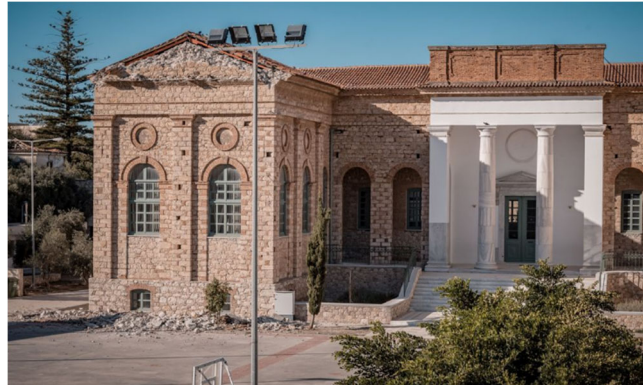
Figure 29. Damage to the Porphyriada school in Karlovasi (Documentonews, 2020).
