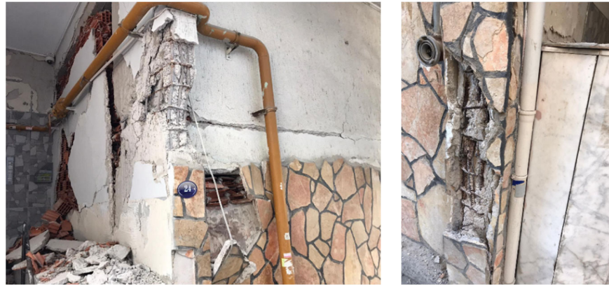
Figure 39. Large transverse reinforcement spacing (left) and corrosion of reinforcing bars (right) (Credit: Ozgur Ozcelik).
