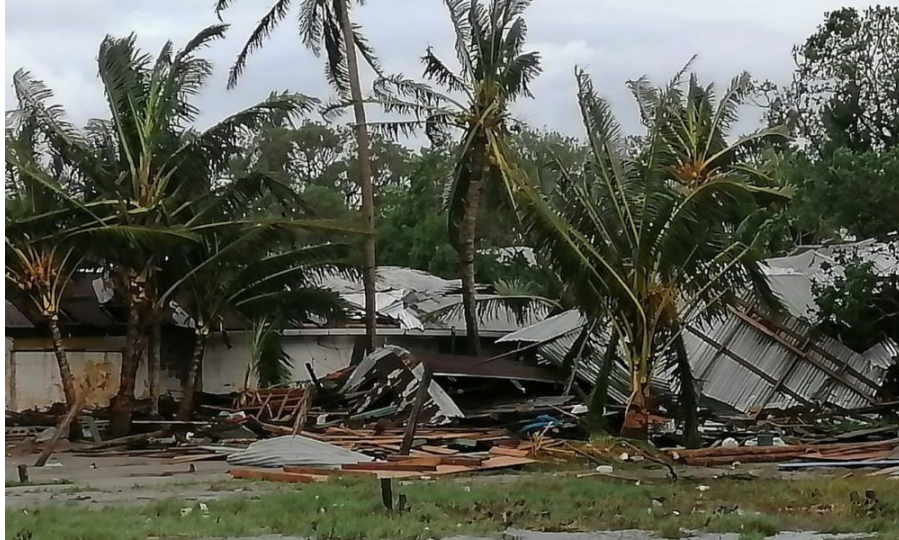
Figure 3.3. Structural collapse of residential building in Managua (Davila, 2020)
