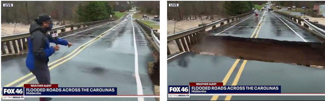
Figure 3.6. Just before and after the collapse of a portion of a bridge on Cheatham Ford Rd in Alexander County, NC (GPS: 35.896155, -81.054812) due to loss of freeboard from rising floodwaters (screen clips from Fox46 Twitter account).
