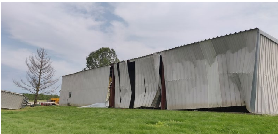
Figure 23. Damaged metal building envelope.
