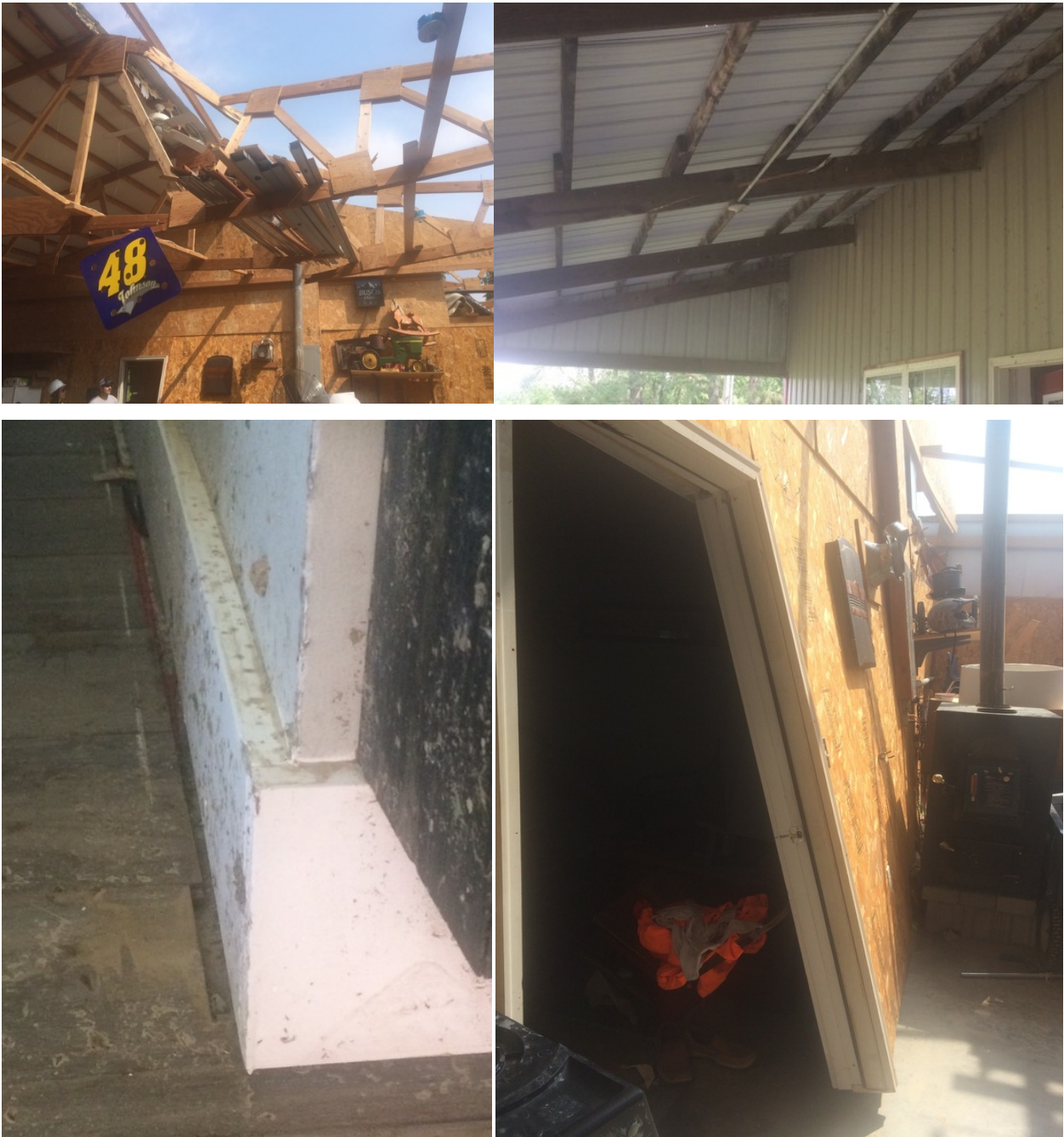
Figure 26. Residential auxiliary structure with severe roof loss (top left), split roof rafters (top right), shifted interior walls (bottom left), and uplifted and released interior walls (bottom right).
