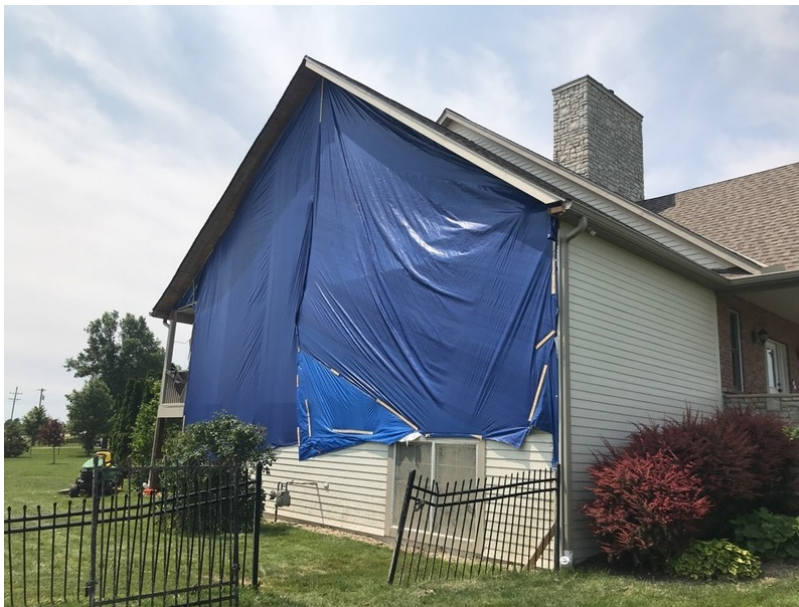
Figure 14. Single-Family house missing east side of the wall.
