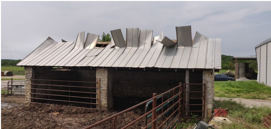
Figure 22. Metal roof exhibiting uplift damage.
