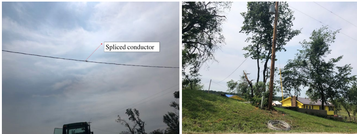
Figure 33. Recovered local power distribution structures: repaired conductor lines (according to the resident) (left); and a reinstalled power pole (right).
