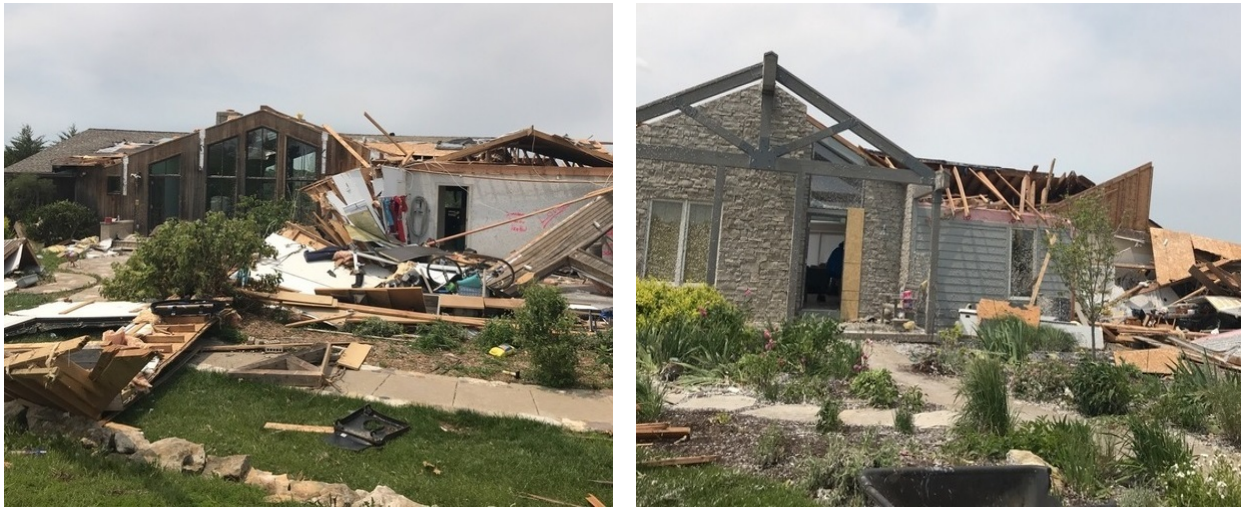
Figure 15. Views of two destroyed single-family wood-frame structures in the Bear Lake neighborhood west of Bonner Springs, Kansas.
