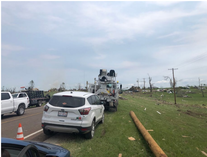
Figure 34. An electric wood pole in-place ready for reinstallation. Also captured in this photo is the linear array of poles, which were all destroyed during the tornado and reinstalled rapidly by Kansas City Power and Lights (based on information from crew member).
