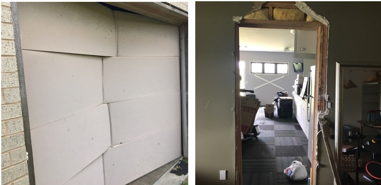
Figure 16. Damage to garage door (left) and interior house door (right).
