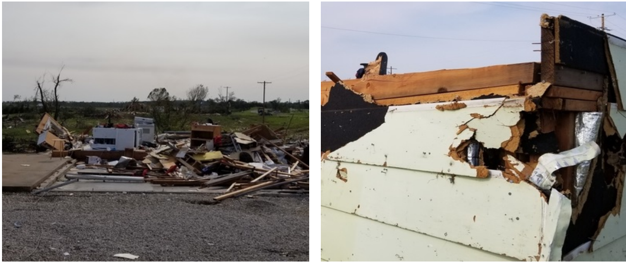
Figure 17. Catastrophically damaged single-family structure in Linwood, Kansas. Photos of the front of the home (left) and the joint where the first-floor walls (missing) rested on the basement walls (right).
