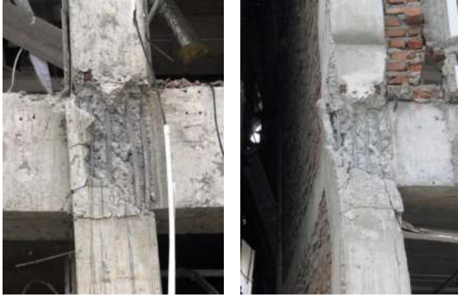
Figure 57: Lack of confinement reinforcement in the beam-column joints may have contributed to the collapse of the Mercure Hotel.
