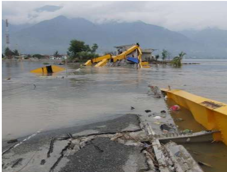
Palu Bridge IV which collapsed during the earthquake (Source: Ian Robertson)
