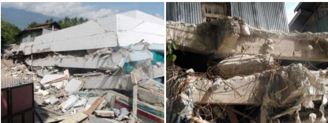
Figure 54: Column failures resulting in complete collapse of the three-story Dunia Baru Restaurant
