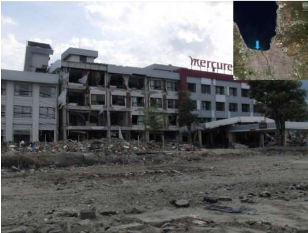
Figure 55: The five story Mercure Hotel experienced a complete collapse of the ground floor.
