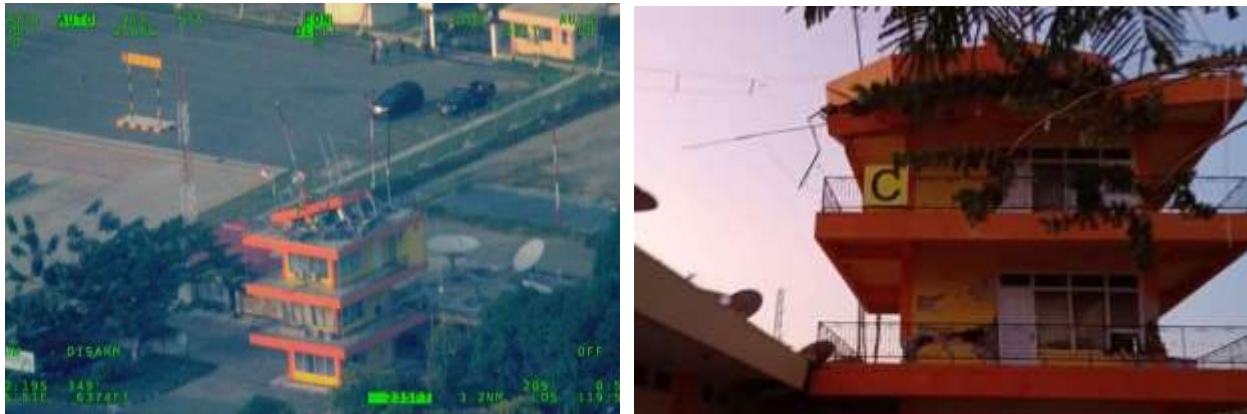
Figure 60: Collapse of the roof of the air traffic control tower at Palu Airport. Structural damage is also evident in walls and columns at the second level of the tower (right).
