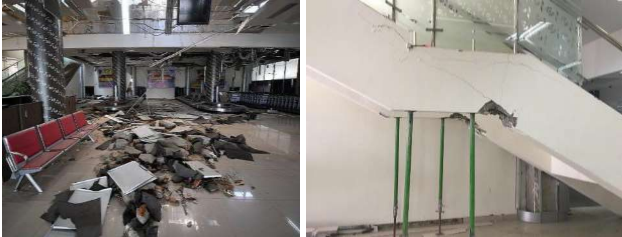
Figure 62: Earthquake damage at Palu airport terminal building: non-structural elements (left) and escalator connecting ground and second floors (right).
