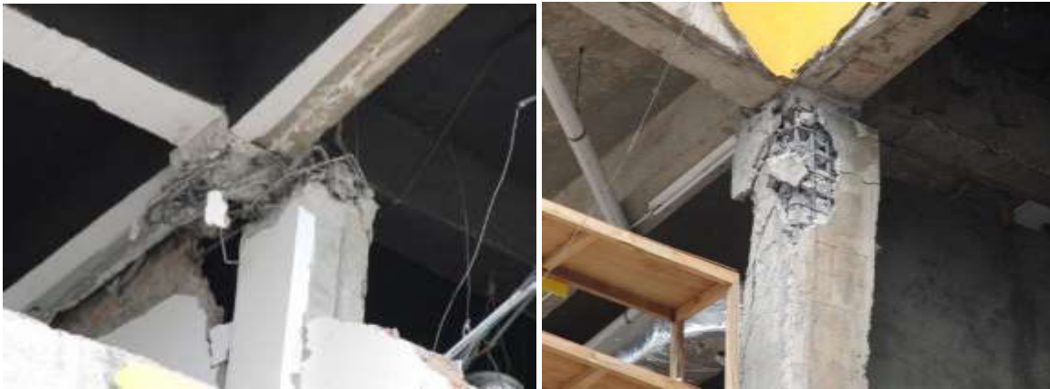
Figure 51: Partial collapse of two interior columns due to shear or flexural failure in the hinging region. Note the lack of damage in the beams framing into these columns.
