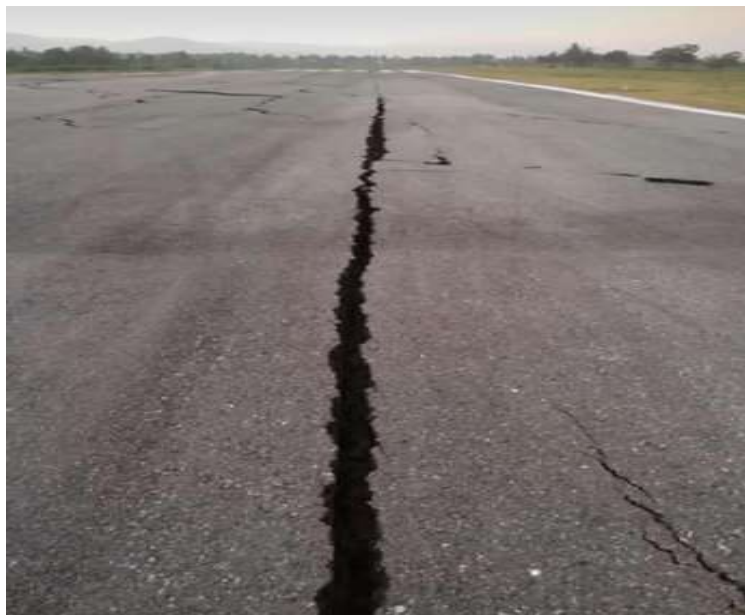
Figure 61: Earthquake damage to Palu airport runway.
