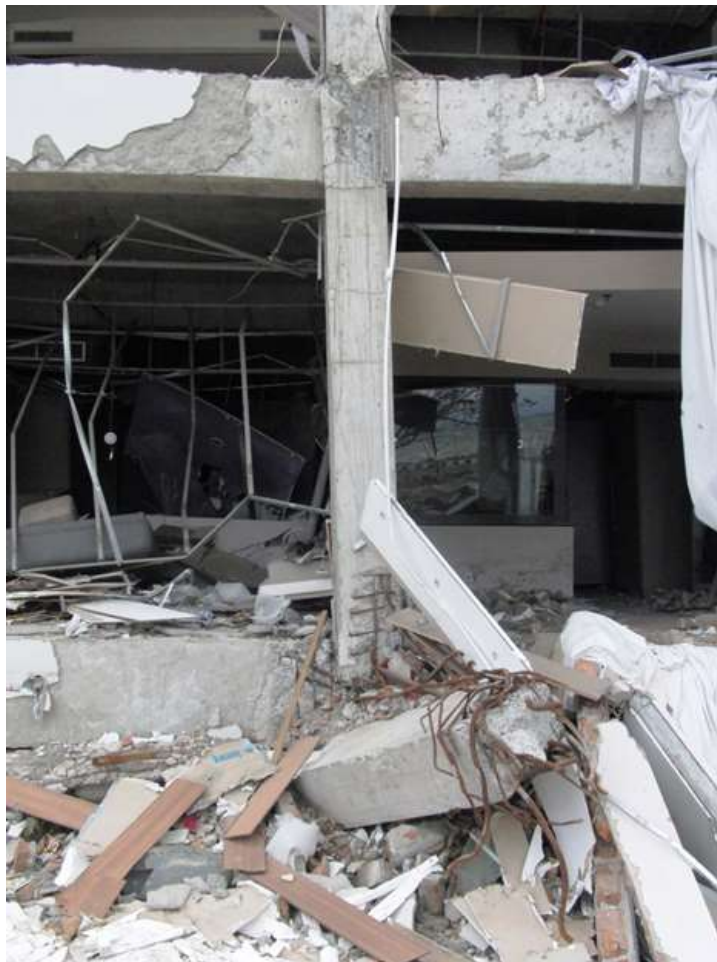
Figure 58: Failed first floor column and damaged joints at second and third floors of Mercure Hotel.
