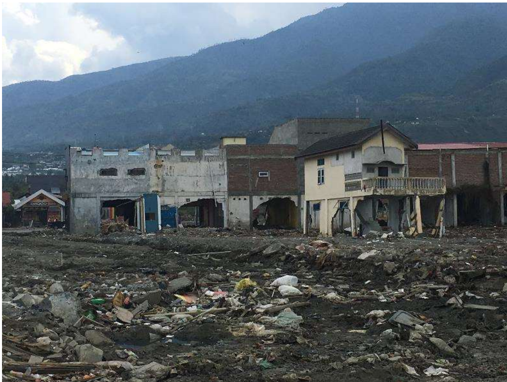
Figure 34: Low-rise reinforced concrete frame structures with unreinforced masonry infill wall panels damaged by tsunami loads (Credit: Ian Robertson).
