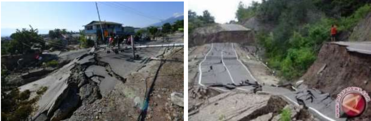
Figure 65: Road failures due to the earthquake.
