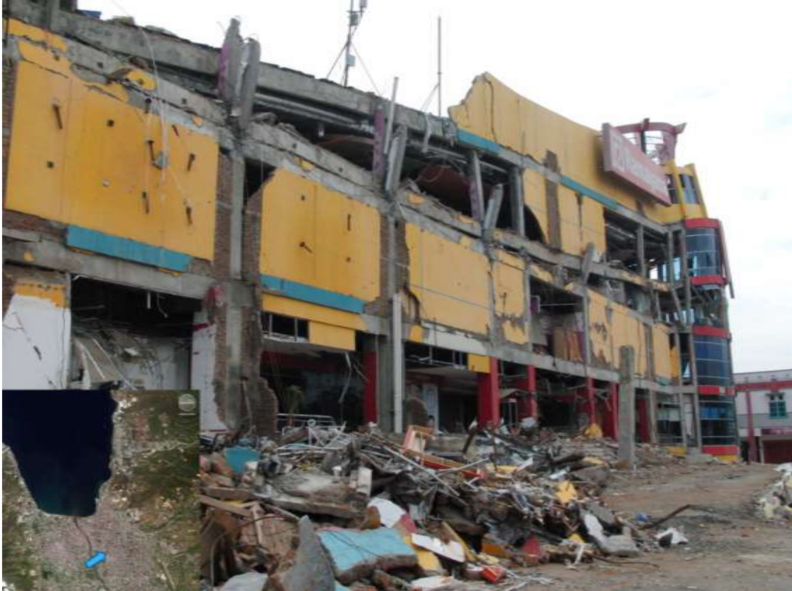
Figure 48: West elevation of Tatura Shopping Mall showing column and joint failures resulting in collapse of the third level and roof.
