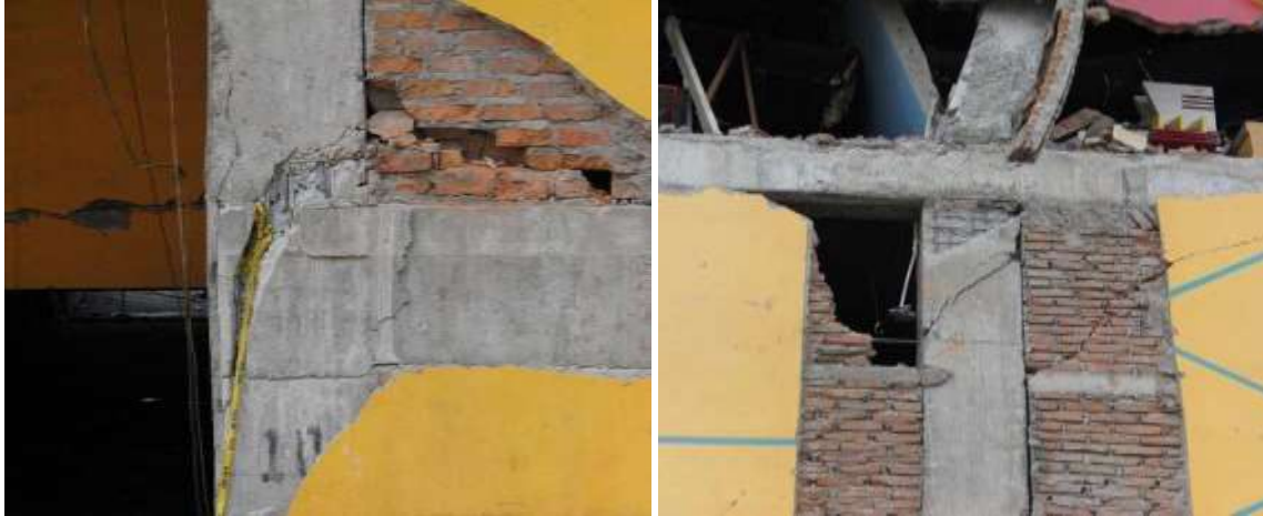
Figure 50: Column shear cracking, possibly exacerbated by presence of masonry infills
