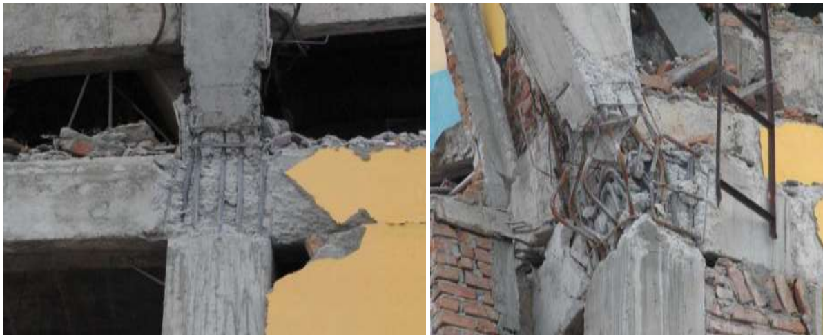
Figure 49: Lack of ties in the beam-column joints probably resulted in buckling of column vertical reinforcement and failure of the unconfined concrete in the joints.
