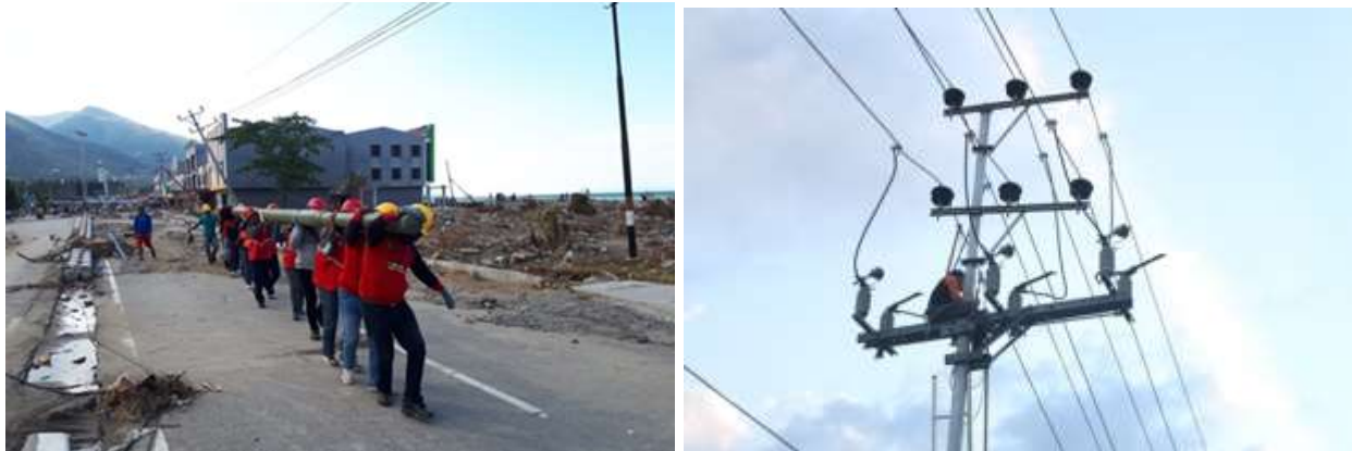
Figure 81: Restoration of the power distribution system within days of the earthquake and tsunami.
