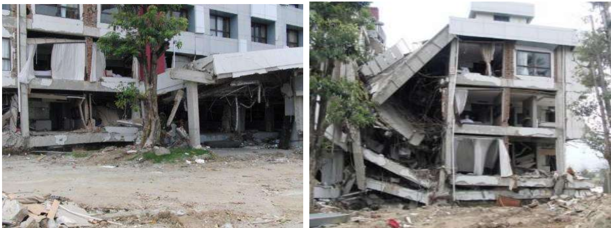
Figure 56: Ground floor collapse (left) and collapse of all floors for one bay (right) of the Mercure Hotel.
