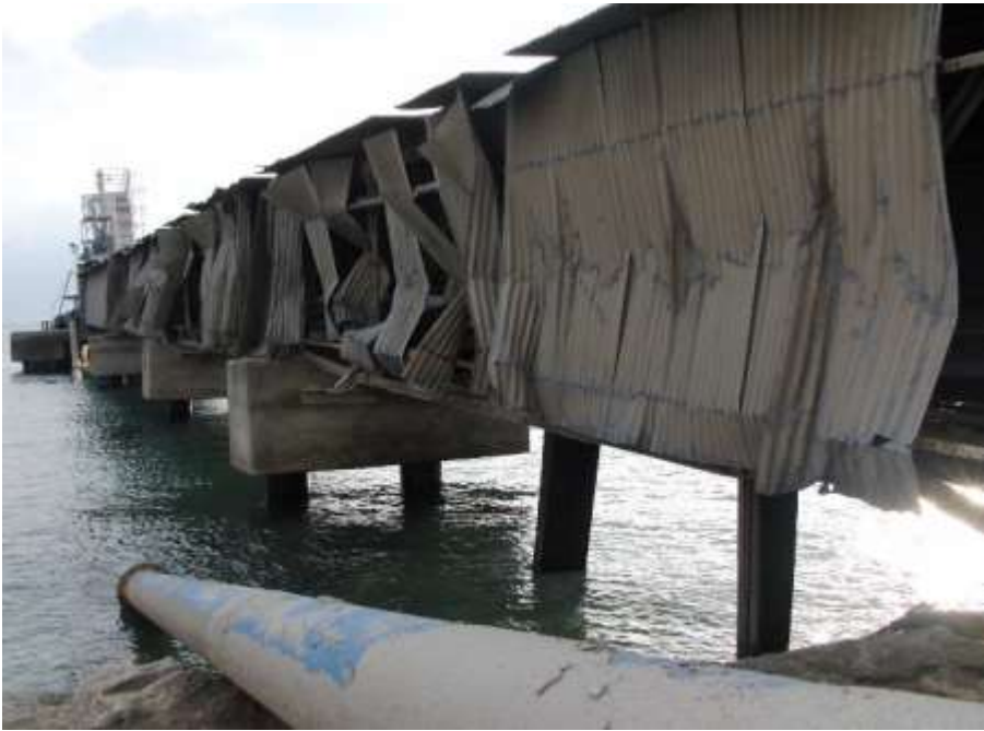
Figure 80: Hydrodynamic damage to sheet metal cladding on the pier supporting a conveyor belt for cement transport from ships to the silos.
