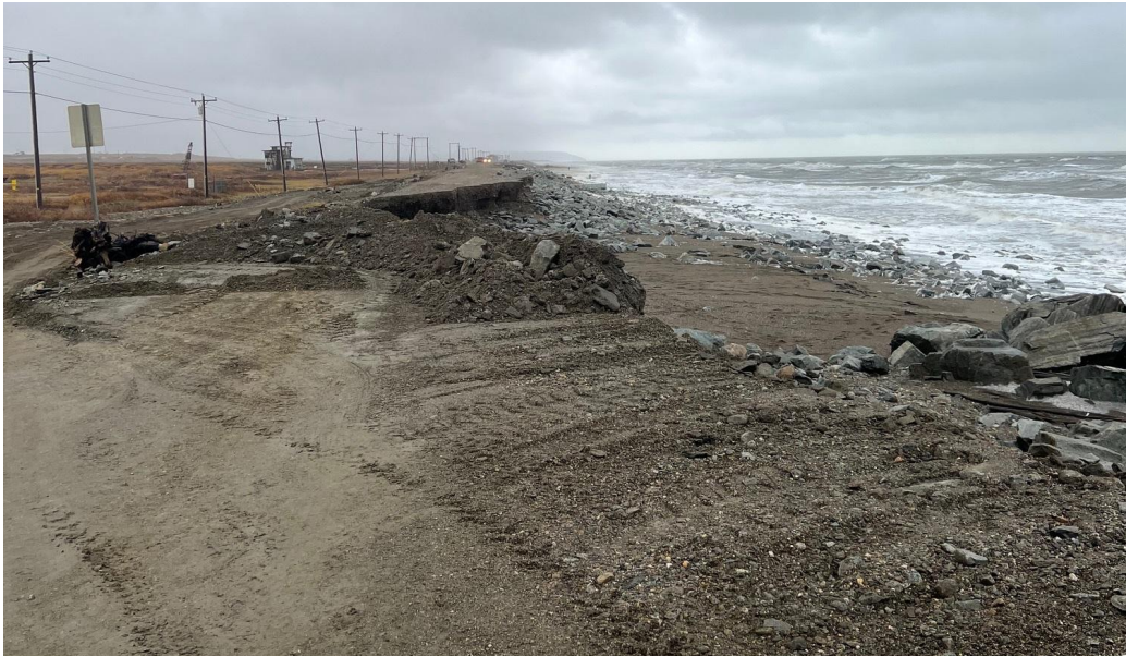
Figure 6.2: Coastal erosion along Nome-Council Highway (source: Bering Strait School District, Alaska DHS & EM 2022b )
