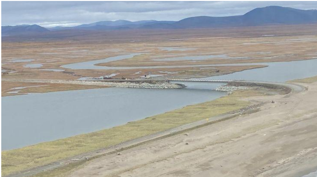
Figure 6.3: Bridge on Nome-Council Highway with some apparent abutment damage (source: Alaska DOT&PF 2022 )
