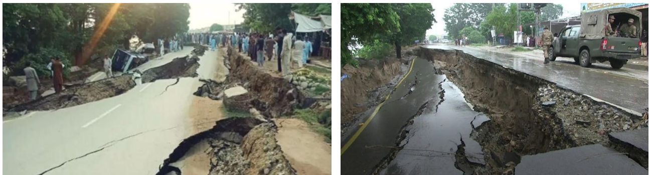
Figure 4. Damage to roads in Kashmir earthquake
