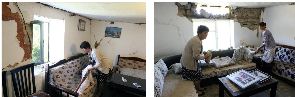
Figure 5. Severely damaged houses in a village near Tirana, Albania quake (AP News, 2019)
