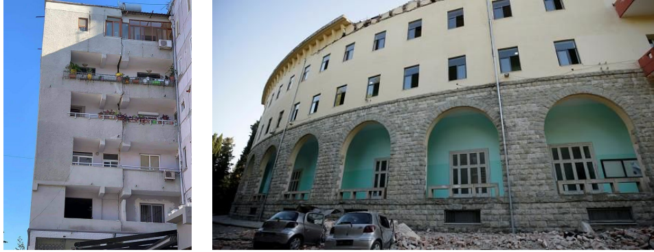
Figure 6. Heavily damaged building with a big crack running all along the height (left); Cars crushed by debris fallen from the collapsed roof a building; Albania quake (Euro News, 2019)
