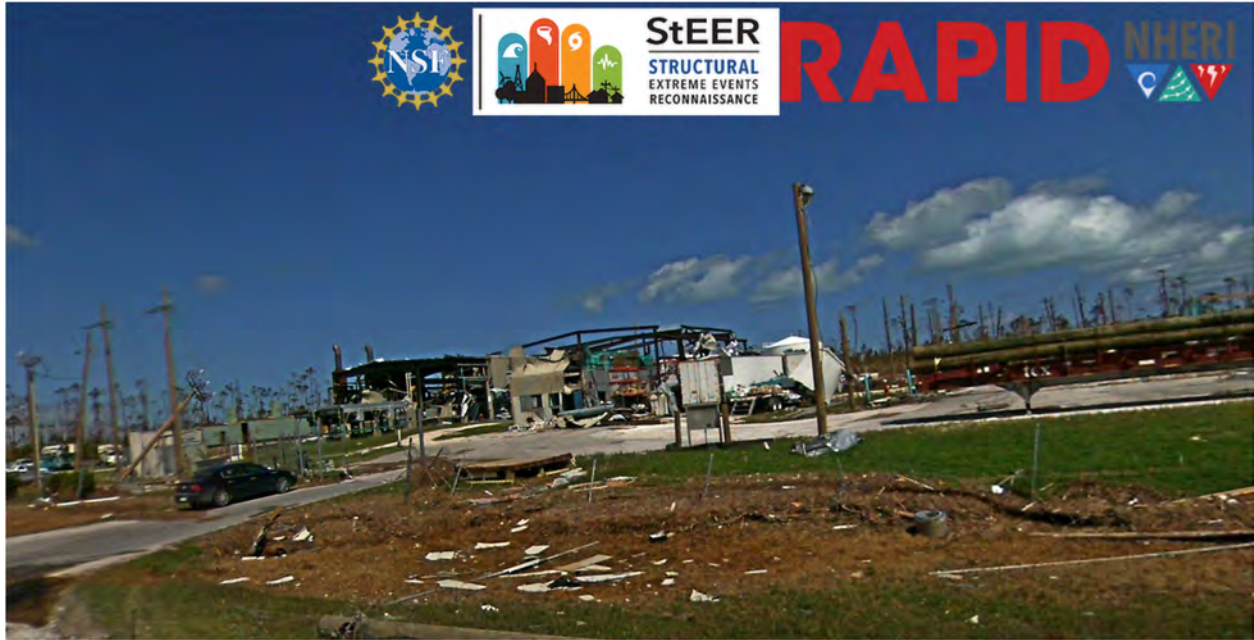
Figure 7.2. Applied StreetView image of damaged Marsh Harbour power plant facility [26.53466, -77.09566].
