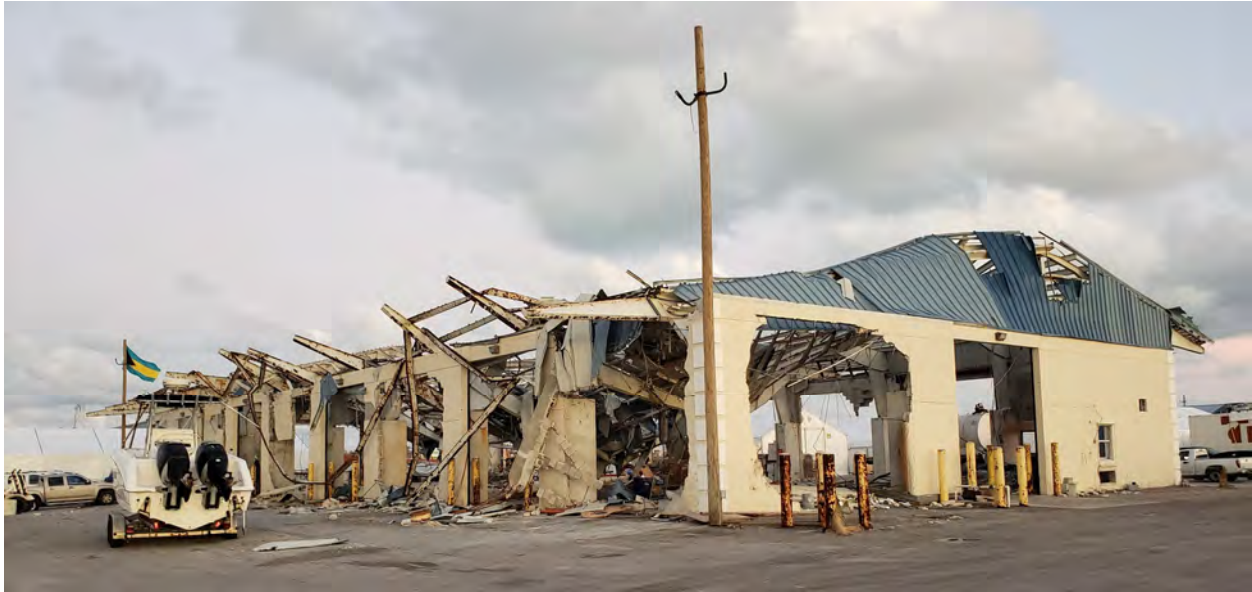
Figure 7.6. Image of damage to warehouse building at Marsh Harbour Government Port [26.54332, -77.06435].
