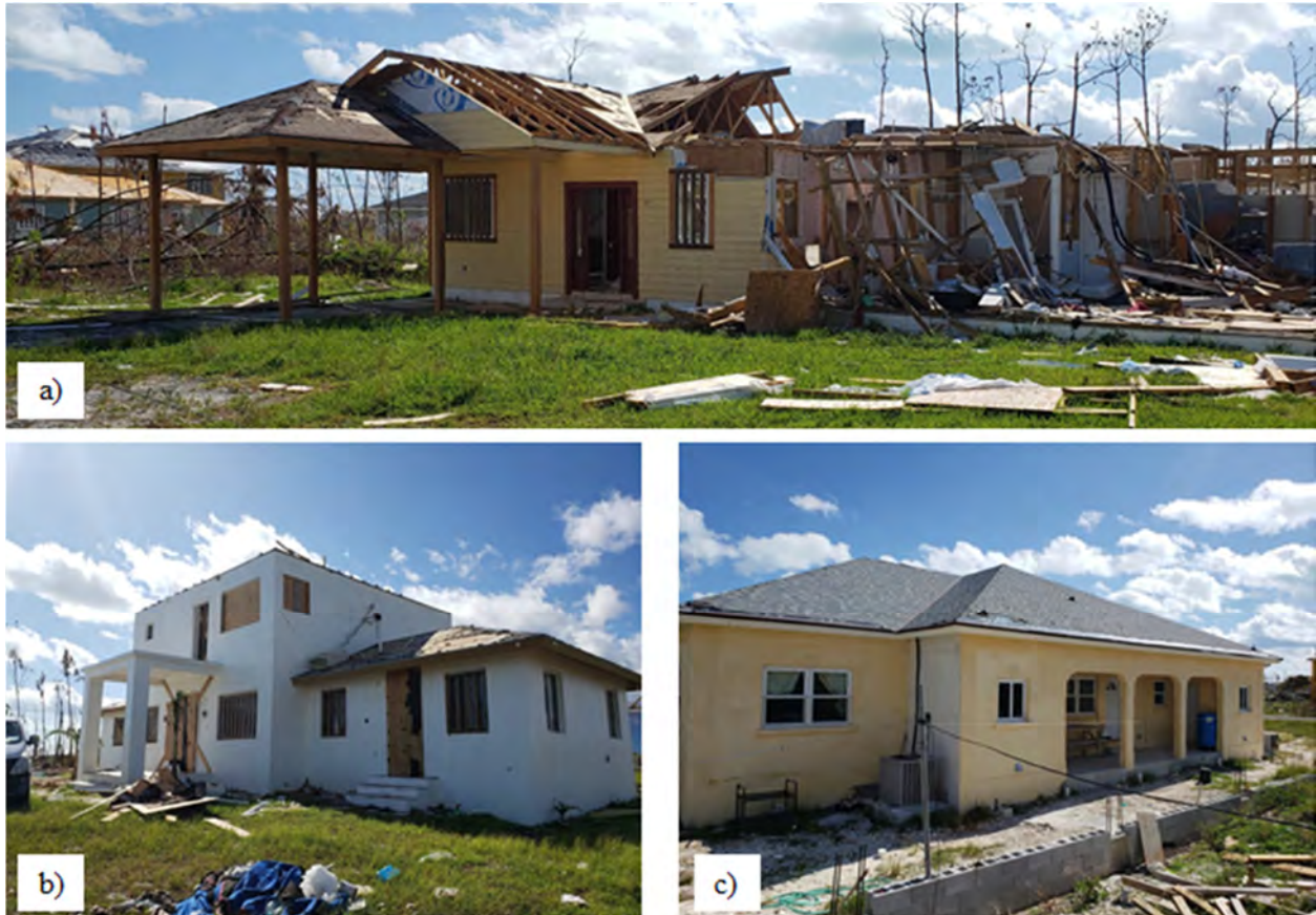
Figure 6.11. (a) Example of “Destroyed” wood-frame residence in Central Pines [26.53908, -77.08815]; (b) Example of “Severe” damage in Central Pines [26.53713,-77.08815]; (c) Example of “Minor” damage in Central Pines [26.63991, -77.08816].
