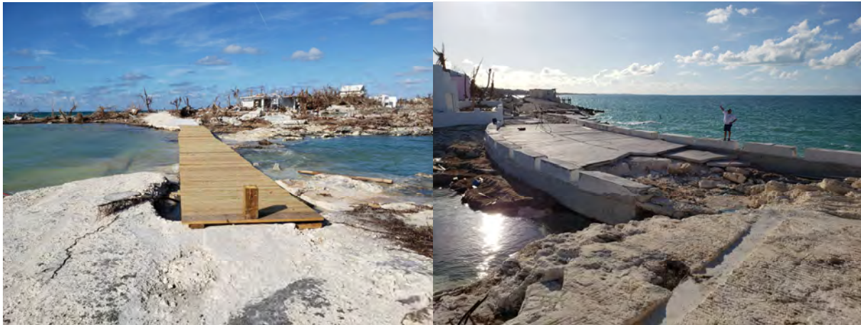
Figure 7.4. Examples of roadway surge damage: (a) Complete roadway washout of Eastern Shores road which has been temporarily replaced with a pedestrian bridge [26.55190, -77.03761]; (b) Roadway erosion of concrete pavement and guardrail on Eastern Shores Road [26.55313,-77.03569].
