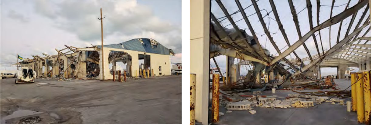
Figure 6.5. Metal building at the International Port Area destroyed by high winds, waves and storm surge.
