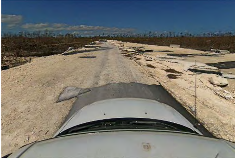
Figure 7.5. StreetView image of damage to a recently reconstructed roadway on the road from Marsh Harbour to Treasure Cay [26.58216, -77.16946].
