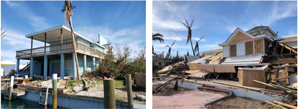
Figure 6.6. Severe damage to residential buildings, including loss of roof over top story (left) and collapse of bottom story in wood-frame building (right).
