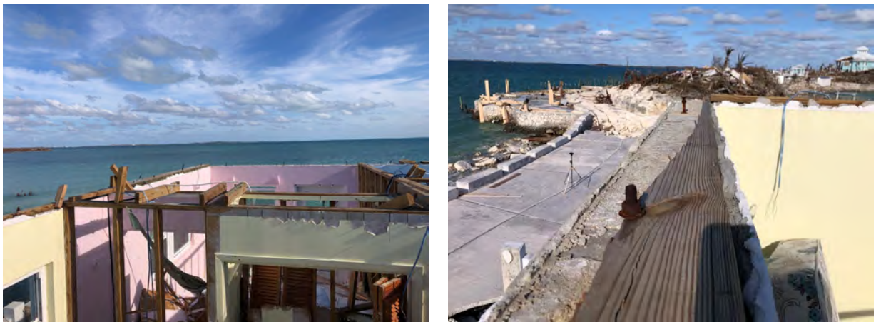
Figure 6.7. Typical connections of elevated wood-frame construction atop reinforced masonry ground floor construction. Anchor bolts were commonly observed anchoring the sill plates (shown above) but in failed buildings, straps were not utilized to provide a strong positive connection between the studs and the sill plate.
