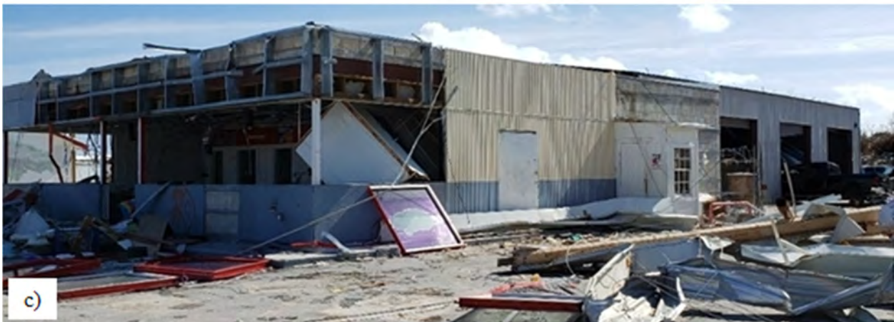
Figure 6.9. Variation of damage to commercial buildings in Marsh Harbour: (a) Minor damage to Maxwell’s grocery store [26.53773, -77.05638]; (b) Moderate damage to Ace Hardware (metal building) which also showed significant water ingress damage [26.536398, -77.06132]; (c) Destroyed gas station with evidence of significant flooding due to the refrigerator that has been lifted and moved [26.53677, -77.06014]
