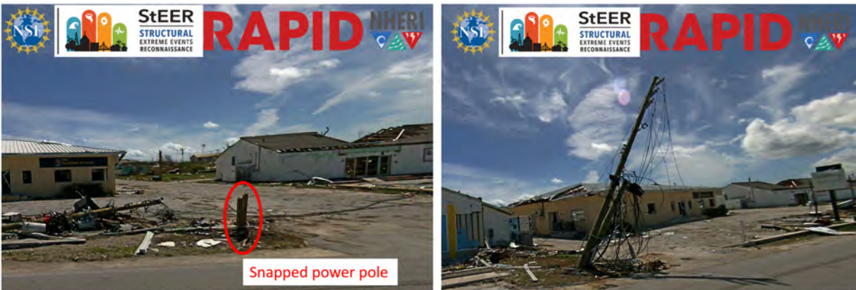
Figure 7.1. Snapped and leaning power poles in the business district of Marsh Harbour captured by the NHERI RAPID EF Applied StreetView camera.
