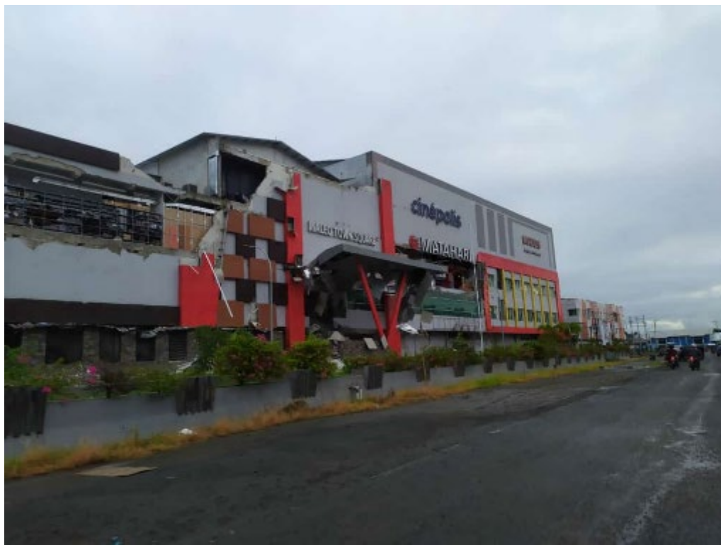
Figure 3.11 Photographs of the Matahari Shopping Center in Mamuju taken from Google Street view (top) and a video frame taken after the earthquake (bottom) (2.6694S, 118.8918E) (Source: https://twitter.com/fad__id/status/1349863151873925120?s=09 )
