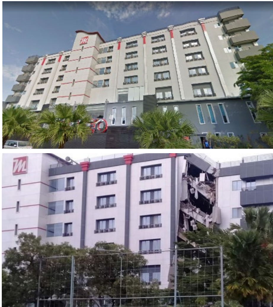
Figure 3.10 Google Street view image (top) and partial collapse (bottom) of the d'Maleo Hotel in Mamuju. (2.6728S, 118.8867E) (Source: Arman/a Majene resident, https://kumparan.com/paluposo/foto-bangunan-rusak-dampak-gempa-majene-sulawesi-barat-1uysWeg3YSB )
