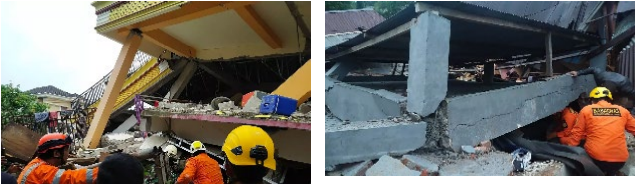
Figure 3.1 Photos of collapsed buildings suggesting the initiation of collapse from failed beam-column joints (Indiatimes, 2021).
