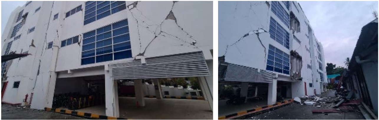
Figure 3.8 Local Power Utility Office built in 2017 with significant facade damage. (2.6771S, 118.895E) (Source: PLN/State Electricity Company Documentation, via detikNews, 2021)
