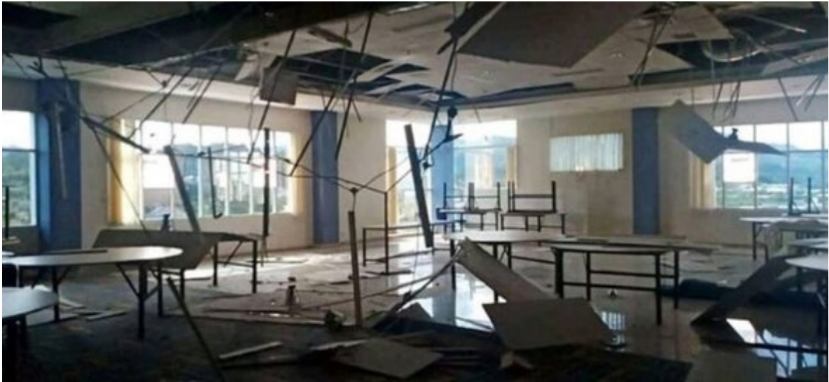
Figure 3.12 Non-structural suspended ceiling damage observed in a building (Reuters, 2021).
