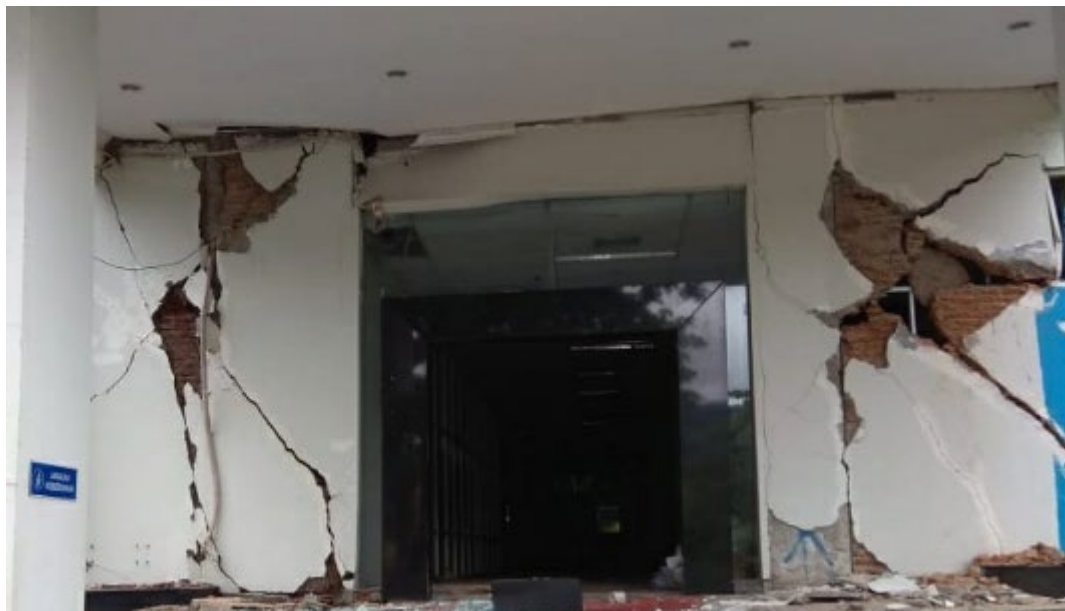
Figure 3.9 Damage experienced by the frame members and infill walls of the Mamuju Tax Office (Twitter, 2021a).
