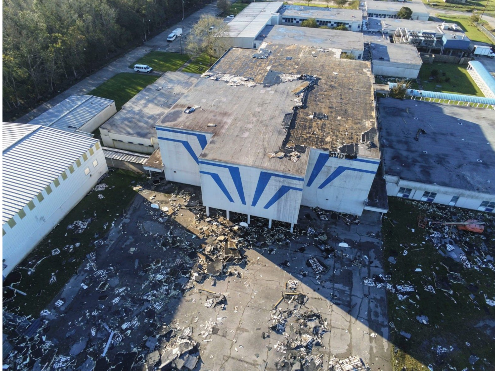
Figure 3.1.2. Drone imagery of damage to commercial roofing system and roof deck at St. Bernard Middle School in St. Bernard, LA (Source: Sandy Huffaker, Getty Images via NWF Daily News )
