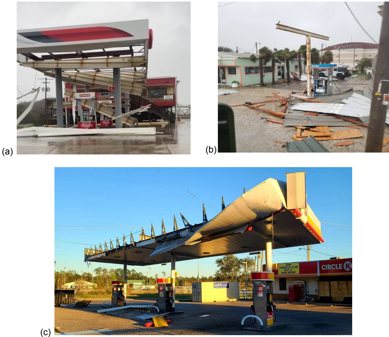
Figure 3.2.3. Damage to gas station canopies: (a-b) in Grand Isle, LA (Source: Facebook 1-2 ) and (c) Waveland, MS. (Source: Twitter )
