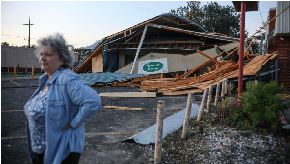
Figure 3.1.4. Collapsed restaurant in Chalmette, LA (Source: Sandy Huffaker, Getty Images via NWF Daily News )
