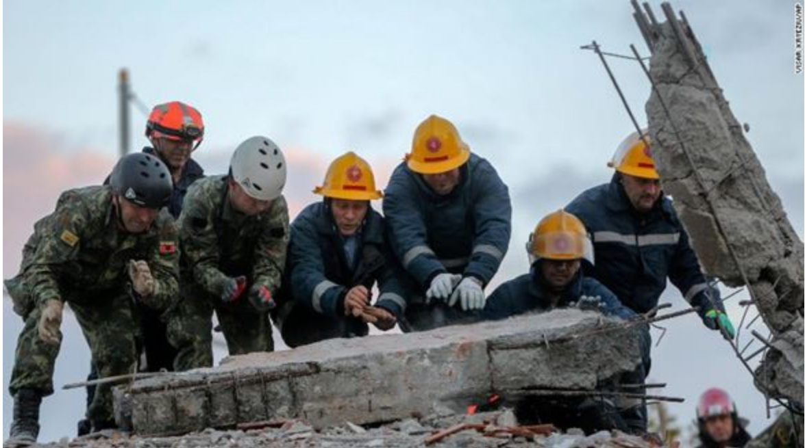
Figure 6. Lack of transverse reinforcement and failure in a diagonal plane associated with shear damage of the vertical element and lack of adequately anchored confining reinforcement in the horizontal element (CNN, 2019)
