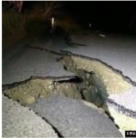
Figure 9. Significant road damage in Tirana (CSEM, 2019)
