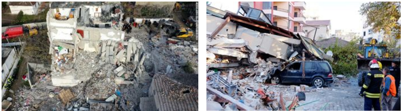
Figure 3. Collapsed reinforced concrete buildings (CNN, 2019)
