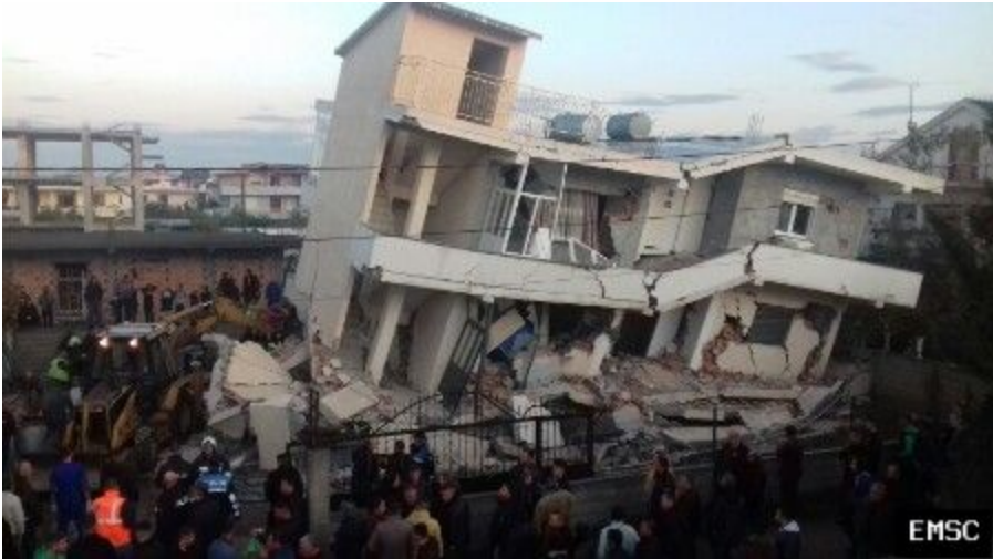
Figure 7. A soft/weak story collapse observed in Durres (CSEM, 2019)
