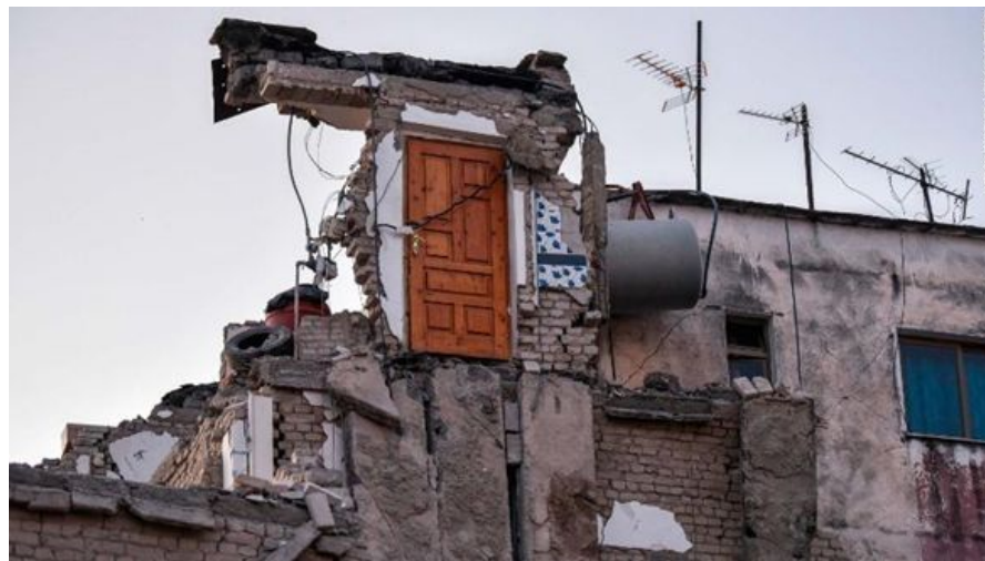
Figure 4. Collapsed masonry building in Thumane with the doorframe standing (CNN, 2019)
