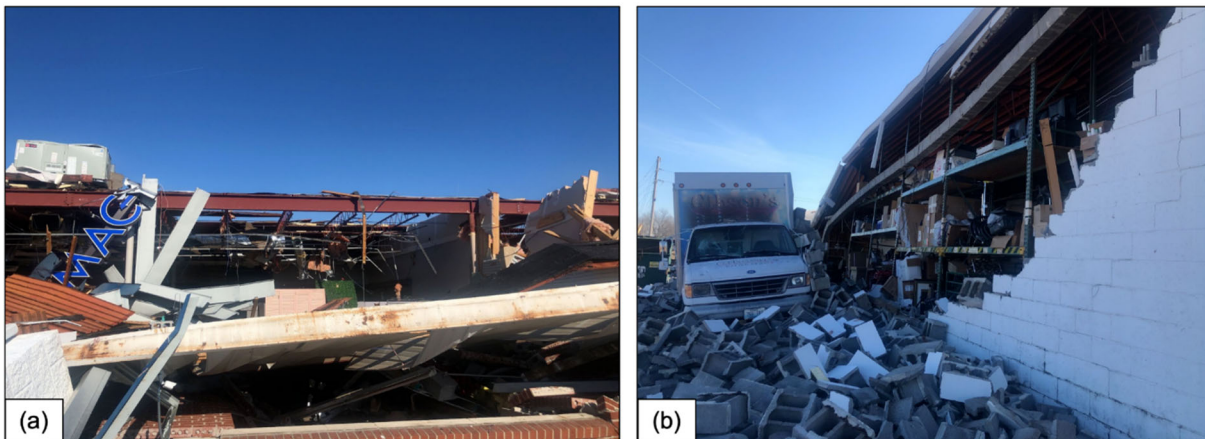
Figure 6.3.5. Examples of failure modes in commercial structures located at 715 E Broadway (Lat: 36.7442, Long:-88.6278) in Mayfield (All images acquired by the FAST).
