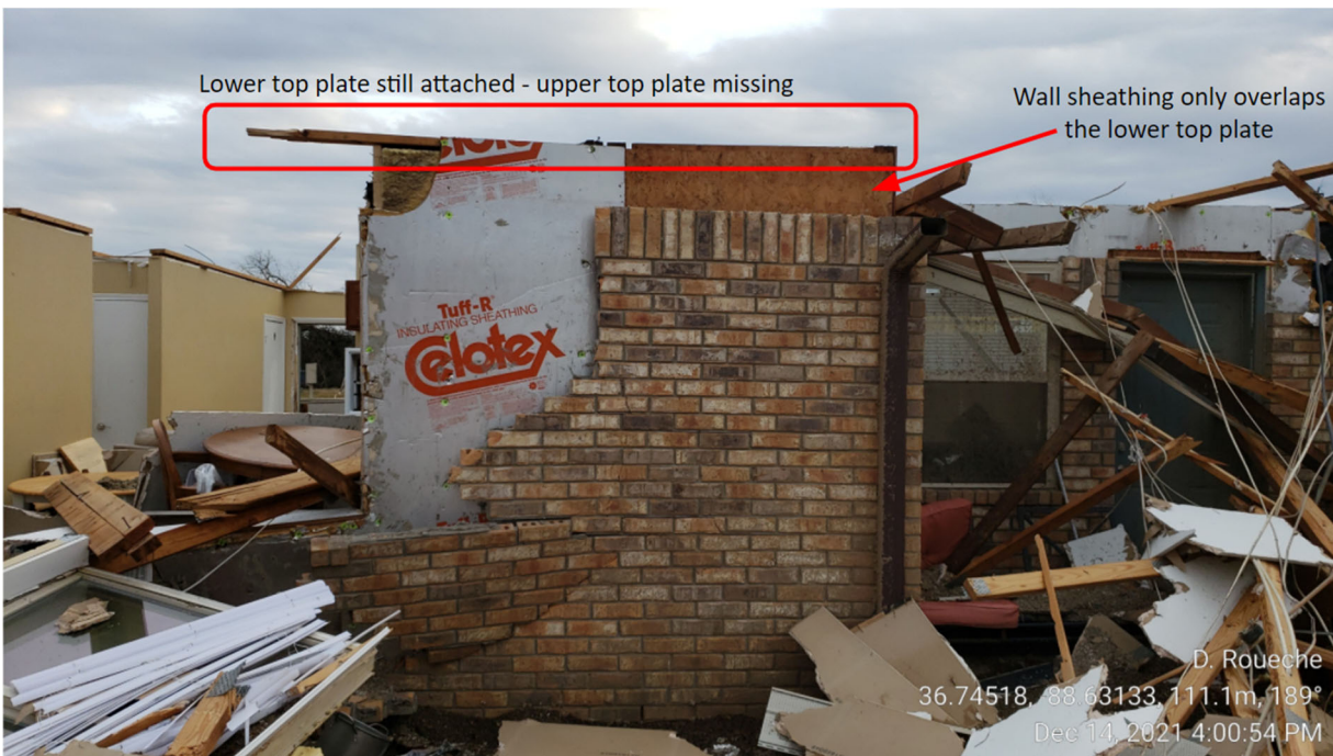
Figure 6.2.5. Roof-to-wall failure occurring via separation of the upper and lower top plates of the stud wall of a unit at the Windhaven Apartment complex (Lat: 36.7452, Long: -88.6313). Removal of the upper of the two top plates was observed around the perimeter of the structure (Image acquired by the FAST).
