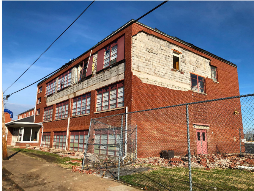
Figure 6.3.4 St. Joseph Catholic School at 702 W Broadway (Lat: 36.7411, Long: -88.6442), Mayfield with failure (or lack) of brick veneer ties to the backup CMU (Photo taken by the FAST).
