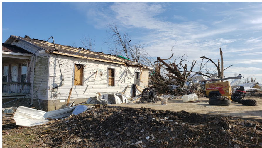
Figure 6.1.6. Single-family residence with building envelope damage 200 ft down-path of the collapsed water tower in Mayfield. The home had been constructed with hurricane straps that wrapped over the top of the wood trusses and connected them to the wood-frame walls. (Images acquired by the FAST).
