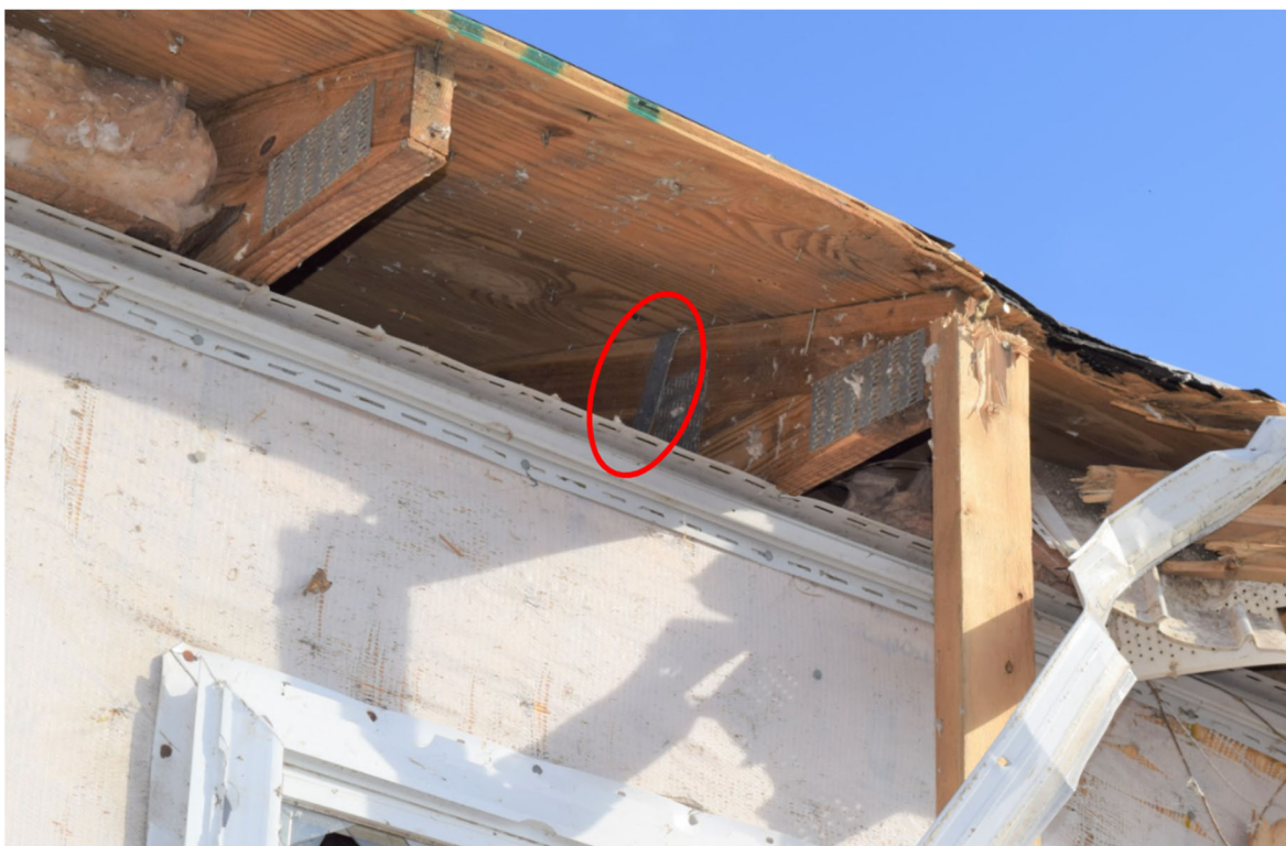
Figure 6.1.7. Steel strap wrapping around a truss to secure it to the wood-frame wall in a home adjacent to the collapsed water tower in Mayfield, KY. (Photo taken by the FAST).
