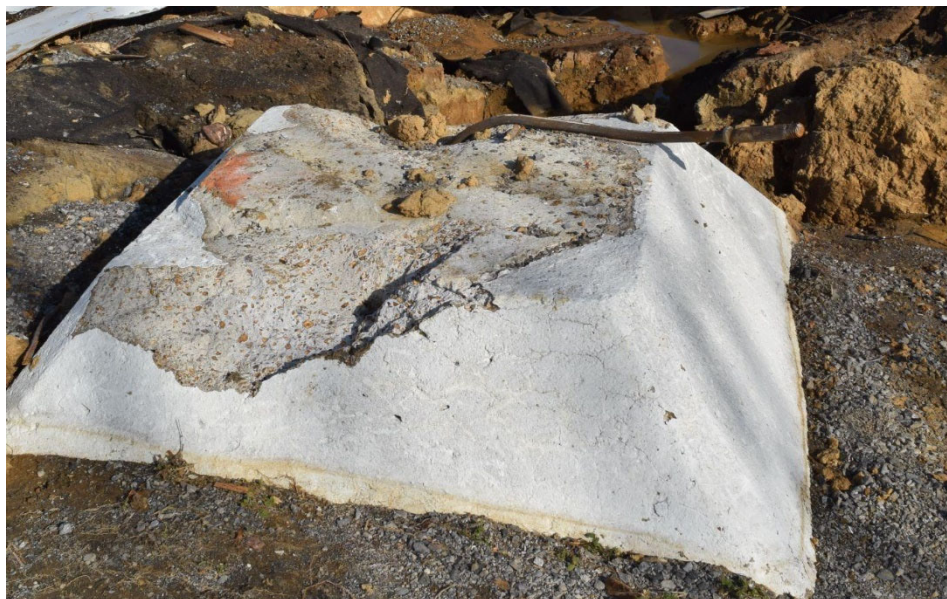
Figure 7.2.2. Shearing of one anchoring rod and pullout of another at one of the eight support footings for the Mayfield water tower (Image acquired by the FAST).
