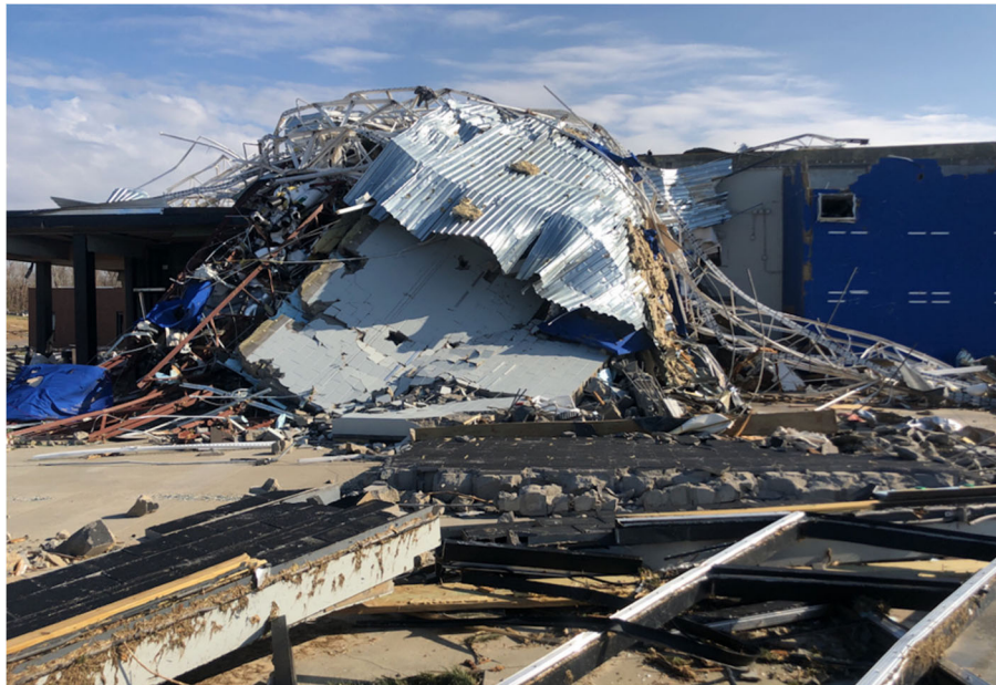
Figure 6.3.10. Collapse of light metal industrial roof trusses of UK Research and Education Center in Princeton, new building (Image acquired by the FAST).
