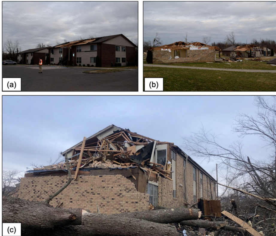
Figure 6.2.2. Examples of damage to multi-family residential structures in Mayfield: (a) Windhaven Apartments (two-story units) (Lat: 36.7447, Long: -88.6297), (b) Windhaven Apartments (one-story units), (c) Tree impact on the Mayfield Garden Apartments (Lat: 36.7350, -88.6436). (All images acquired by the FAST).
