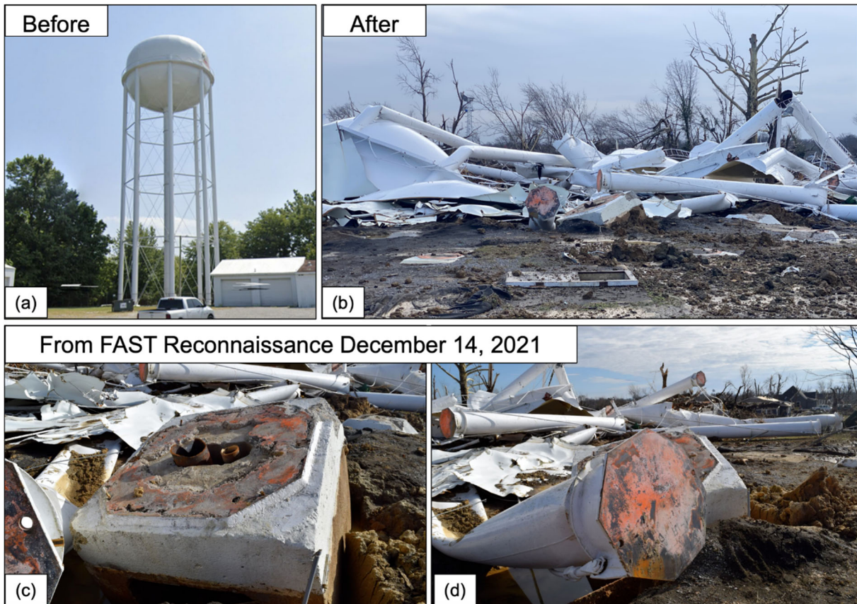
Figure 7.2.1. (a) Water tower in Mayfield (Lat: 36.7389, Long:-88.6425): (a) before and (b) after 10 December tornado (source: Chris Jackson on Twitter ) with a closer evaluation of footings during the FAST assessment (c & d).
