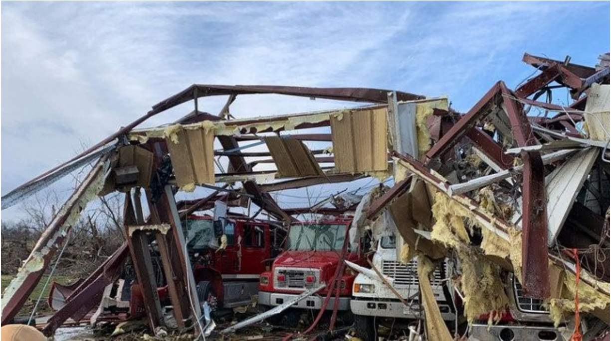
Figure 6.4.2. Damage to Cayce Volunteer Fire Department building (Lat: 36.5551, Long: -89.0326) in Fulton County, rendering emergency equipment inoperable (source: FirefighterCloseCalls.com ).
