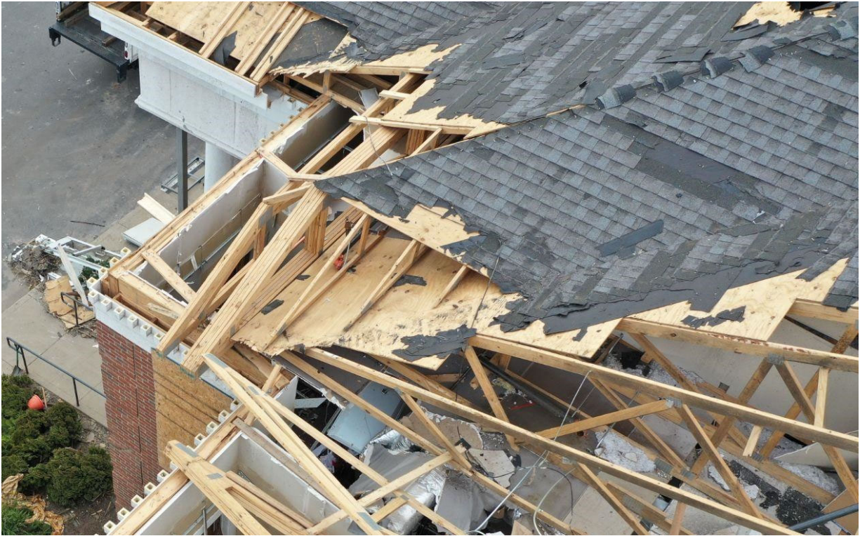
Figure 6.3.6. Roof-to-wall connection failures at the FNB bank (Lat: 36.7419, Long: -88.6350) in downtown Mayfield (Photo taken via UAV by the FAST).
