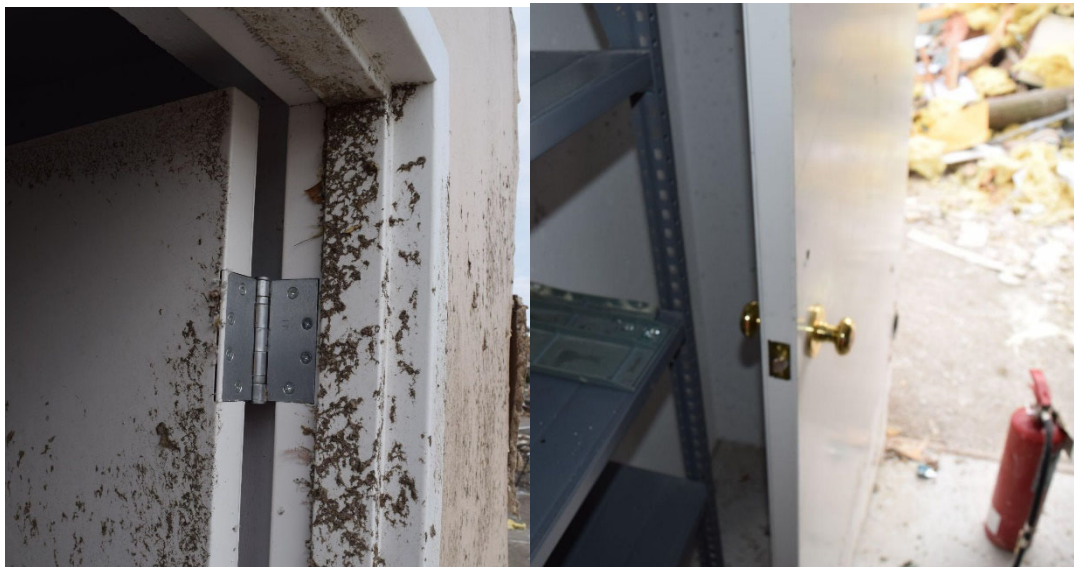
Figure 6.6.3. Door hardware for safe room in attorney’s office building shown in Figure 6.6.1(b) (Photos acquired by the FAST).
