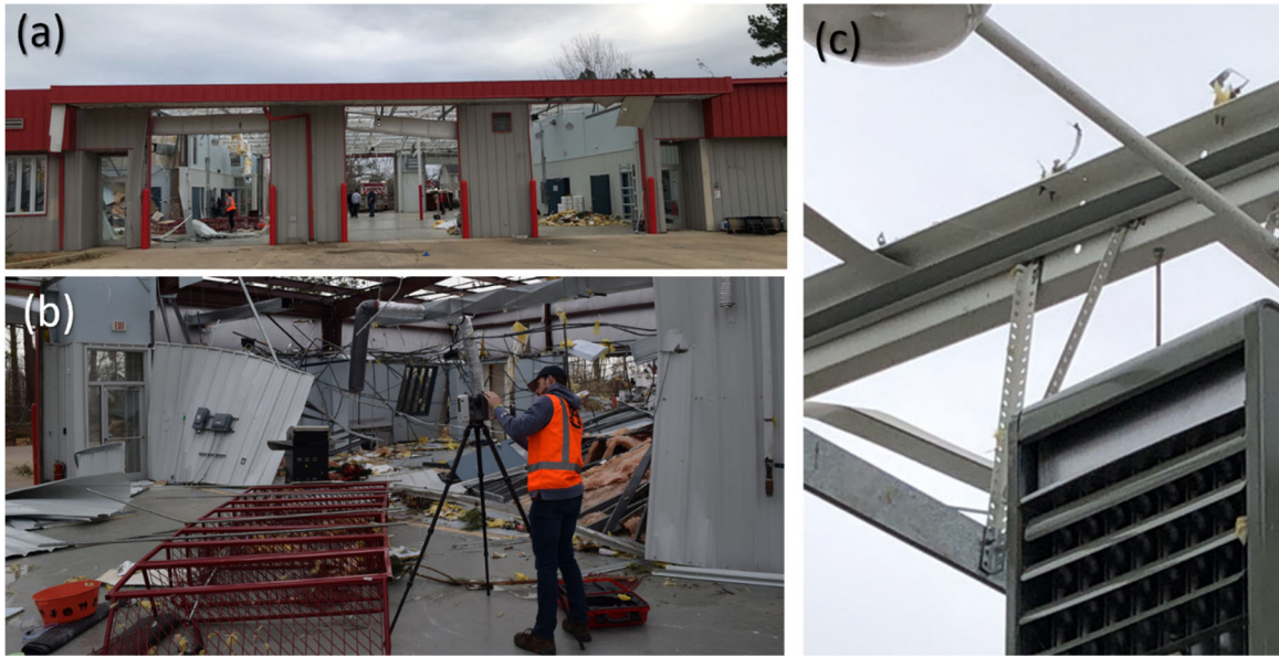
Figure 6.4.4. East Marshall District Station 1 (Lat: 36.9232, Long: -88.2476). (a) Exterior doors were blown in and all roof cladding uplifted; (b) LiDAR scans were collected inside and outside the building; (c) roof panels were attached to the roof structure through flexible ties that were fastened to the top flange of the z-purlins. Failure occurred at the connection between the flexible tie and the roof panel. All images acquired by the FAST.
