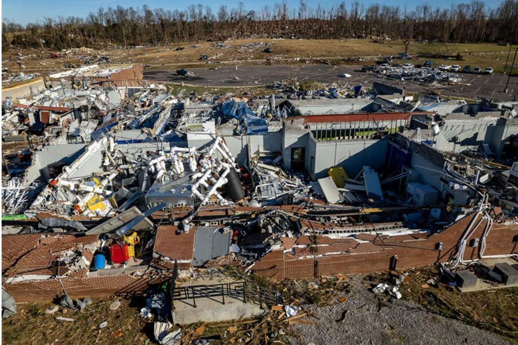
Figure 6.3.9. A closer view of destruction in the Grain and Forage Center of Excellence at the University of Kentucky Research and Education Center (Source: KATIE PRATT, The Paducah Sun ).
