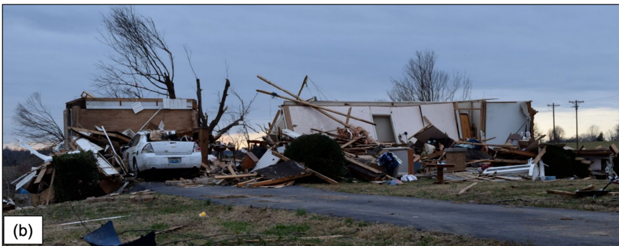
Figure 6.1.4. Representative damage to single-family homes in Princeton, KY along (a) Dogwood Ln (Lat: 37.0808, Long: -87.8984), and (b) Country Club Ln (Lat: 37.0781, Long: -87.9052), showing wood-frame structures with roof structure failures and subsequent wall collapses. (Images acquired by the FAST).
