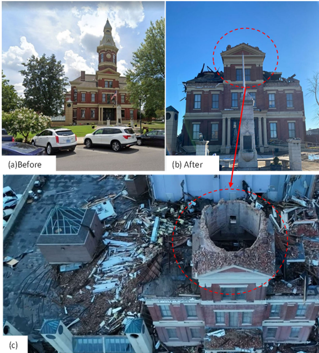
Figure 6.3.3. Damage to the 133-year-old Graves County Courthouse (Lat: 36.7413, Long: -88.6352) building (a) before, (b) after damage, and (c) aerial view of destroyed tower (source: CNN and NY Times ).
