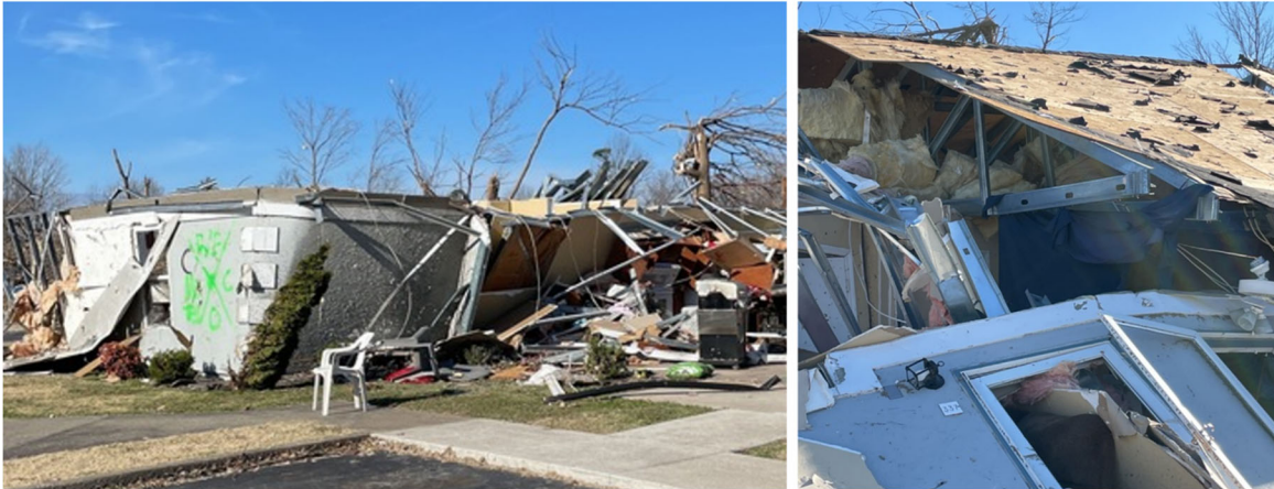
Figure 6.2.6. Collapse of a cold-formed steel framed unit at the Mayfield Manor Apartments in Mayfield, KY (All images acquired by the FAST).
