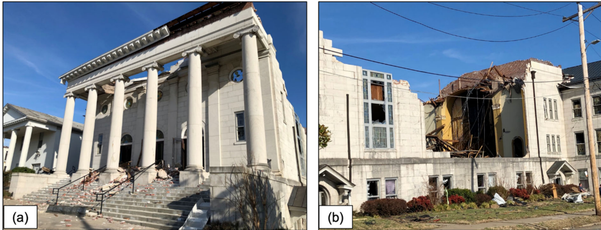
Figure 6.5.2. Damage to First United Methodist Church (Lat: 36.7399, Long: -88.6366) in Mayfield, KY. Images acquired by the FAST.
