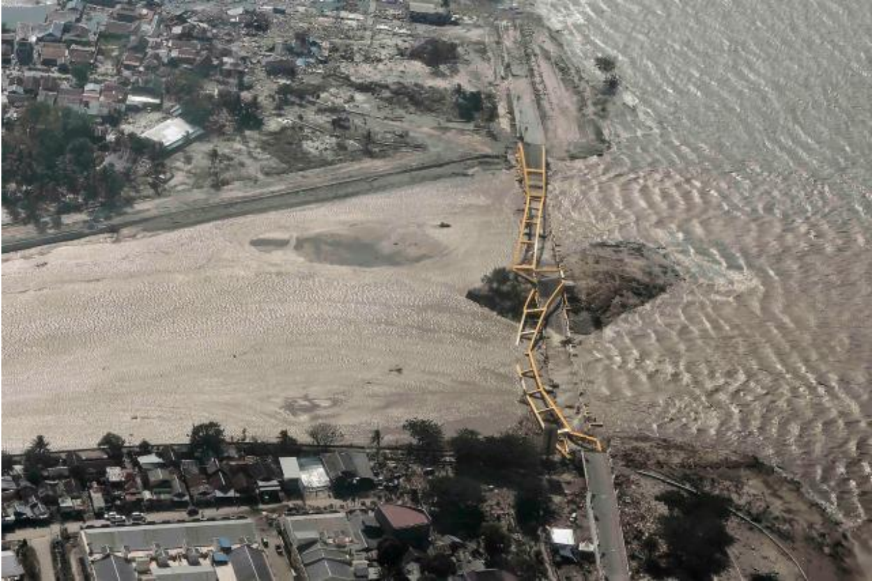
Figure 25: Palu Bridge IV after earthquake and tsunami
