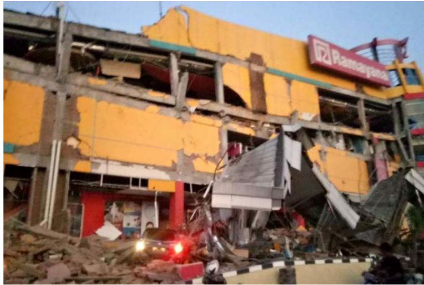
Figure 15: A reinforced concrete Shopping Center in Palu experienced partial collapse during the earthquake (Photo: AFP/BNPB)
