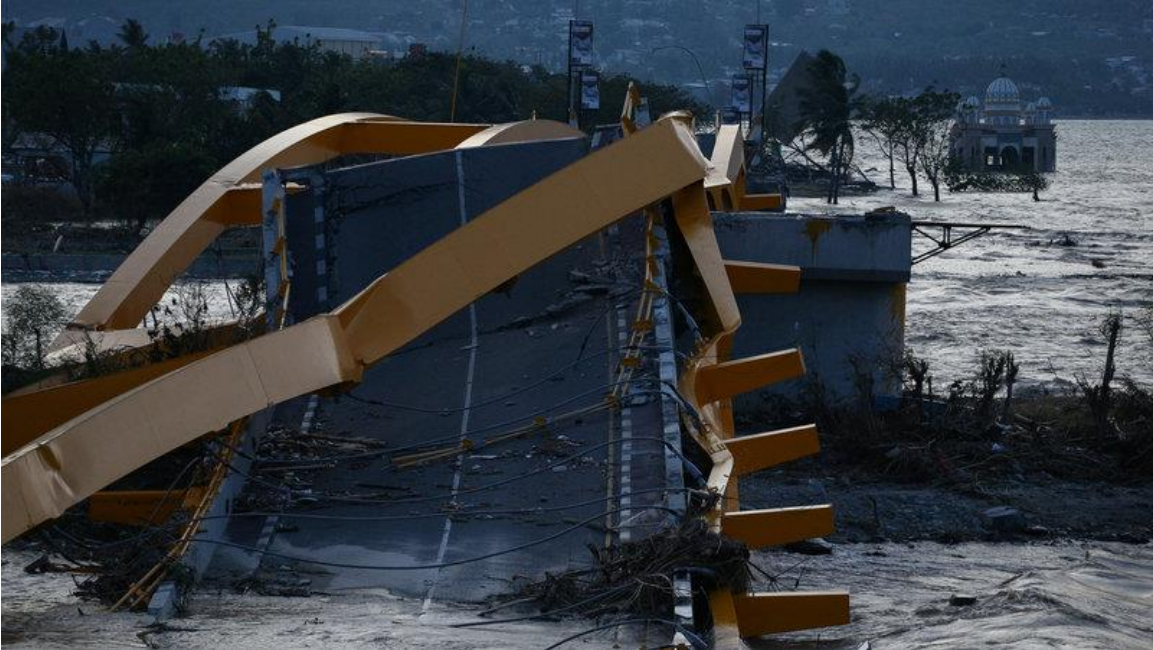
Figure 26: Palu Bridge IV after earthquake and tsunami (Photo: Athit Perawogmetha/Reuters)
