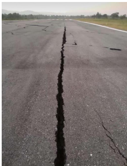
Figure 32: Damage to Palu's Mutiara Sis Al Jufri Airport runway due to ground movement.
