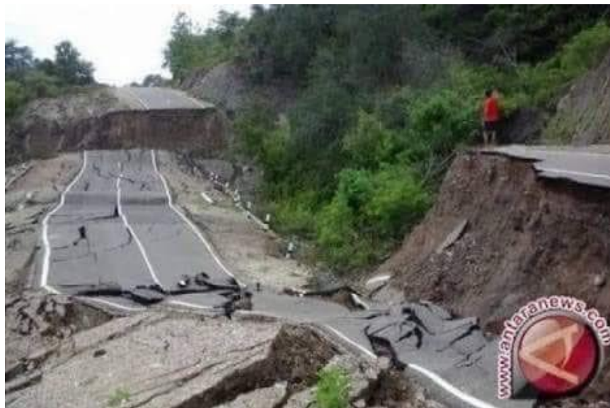
Figure 30: Failure of roadway due to landslide induced by the earthquake.
