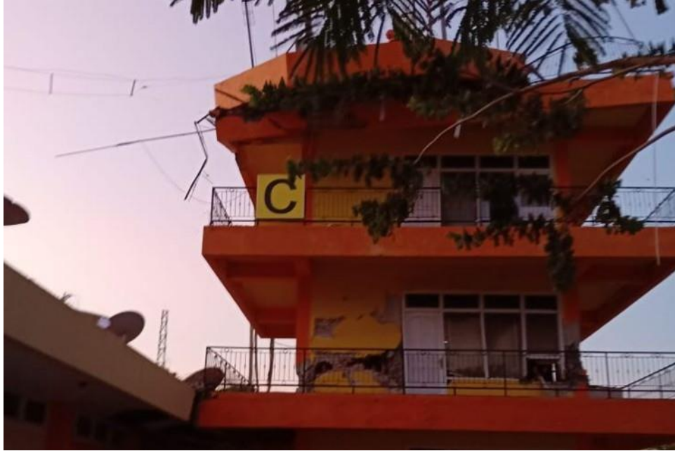
Figure 21: Earthquake damage to airport control tower.
