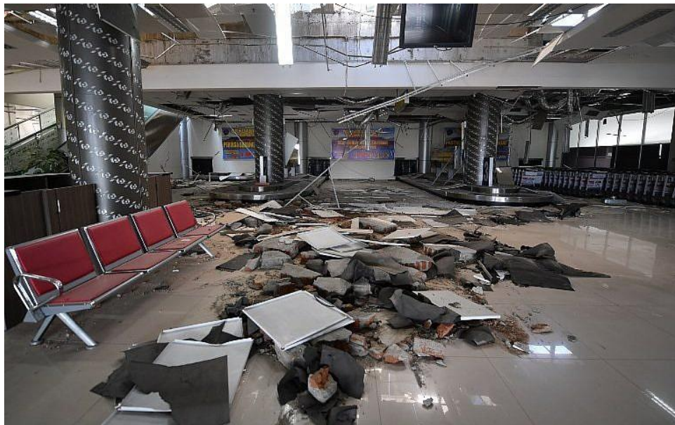
Figure 22: Damage inside airport terminal building (AFP Photo/Adek Berry)
