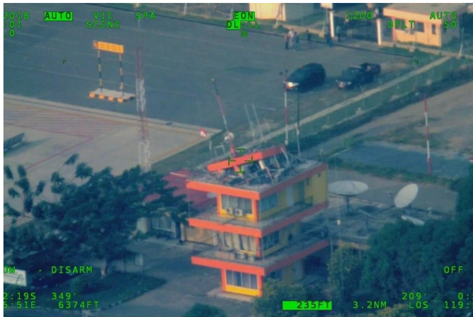
Figure 20: Airport Control Tower after earthquake with top level collapse (0.91670 S, 119.90654 E)
