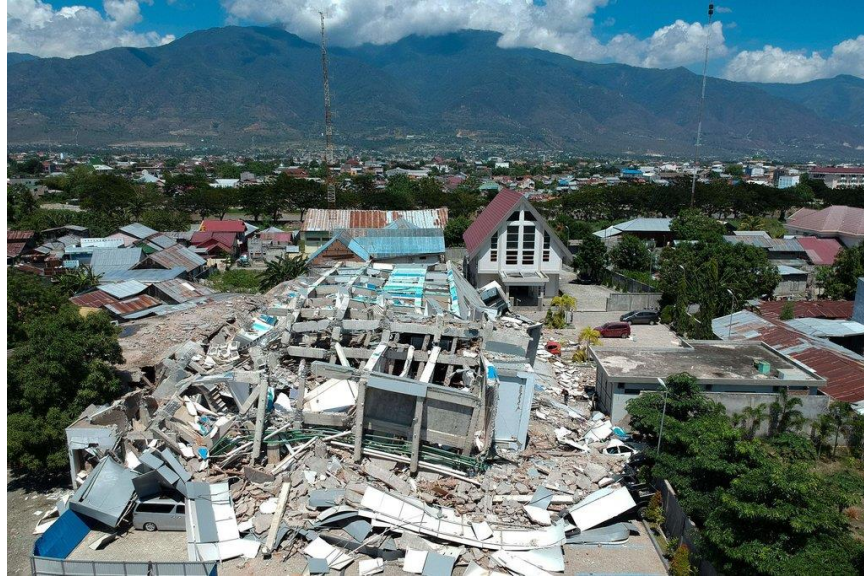
Figure 13: Collapsed Roa-Roa Hotel after earthquake
