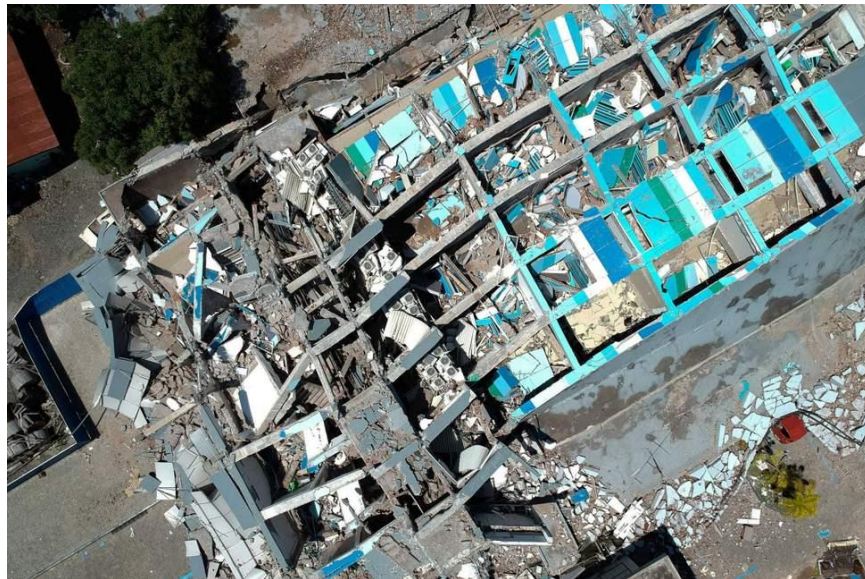
Figure 12: Collapsed Roa-Roa Hotel after earthquake
