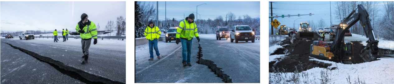
(b) A crack occurred in the road at the International Airport Road off-ramp on southbound Minnesota Blvd. 28
