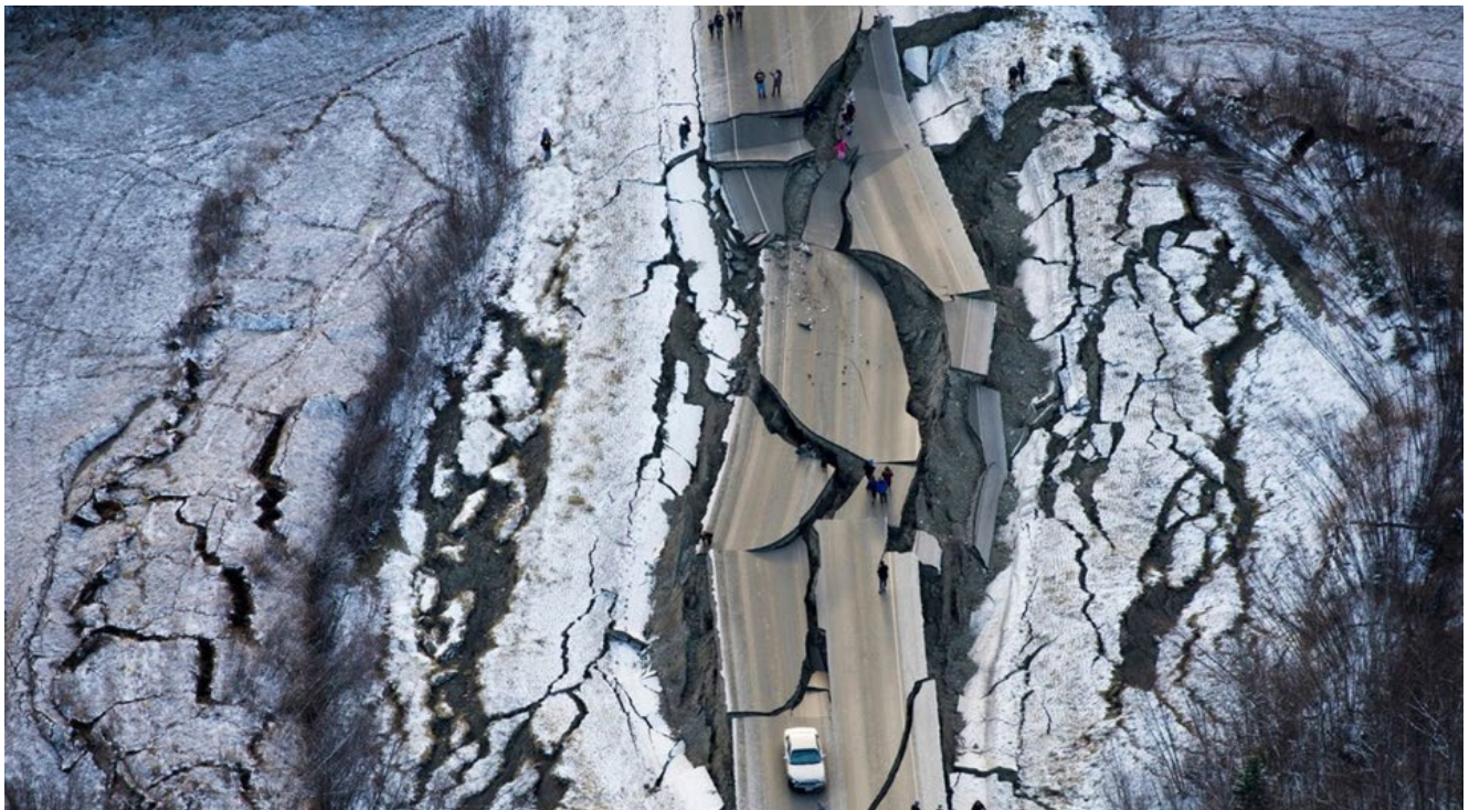
Figure 30: Aerial photo of damage on Vine Road, south of Wasilla 35
