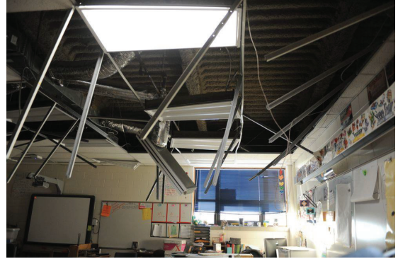
( Anchorage Daily News ) Failure of ceilings in some classrooms at Hanshew Middle School
