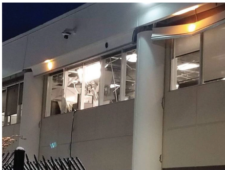
Office building damage, Anchorage
