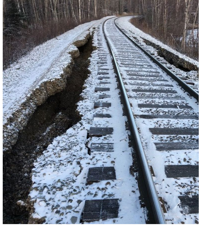
Figure 28: Cracks along parts of Alaska Railroad system 31
