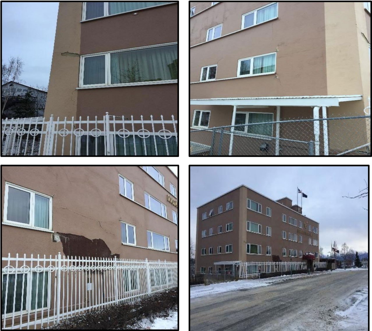
Figure 13: Major cracks observed in Anchorage Grand Hotel, Downtown Anchorage, Alaska 11
