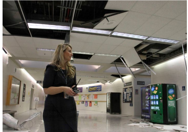
(b) Ceiling tiles came down at Chugiak High School in Chugiak 20
