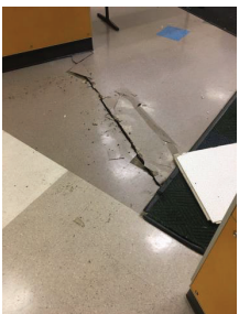
( Twitter ) Damage to school floor - school name not yet identified
