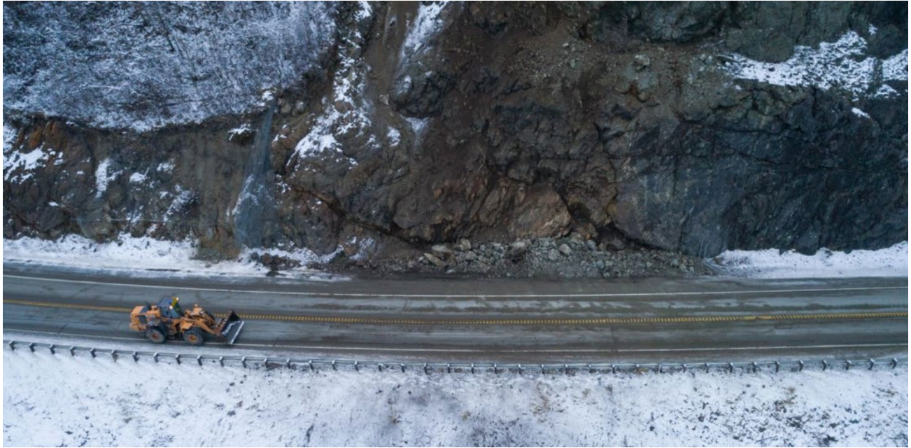
Figure 33: The Seward Highway near McHugh Creek was temporarily closed due to a rockslide 38
