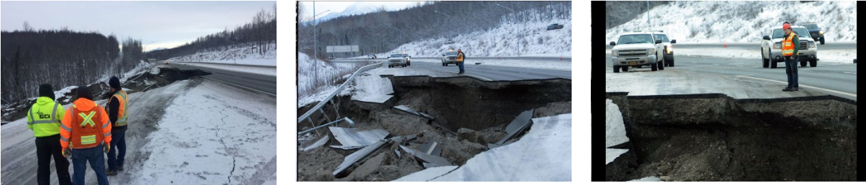
(a) Damage to Glenn Highway southbound lanes between Eklutna and Mirror Lake 27
