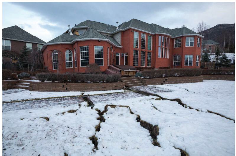
Residential Building in Eagle River damaged due to earthquake https://www.adn.com/alaska-news/2018/12/01/anchorage-fire-chief-how-to-look-for-serious-structural-damage-at-home/
