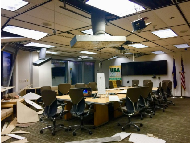
(a) Ceiling tiles that had fallen down in one of the rooms on The University of Alaska Anchorage 19
