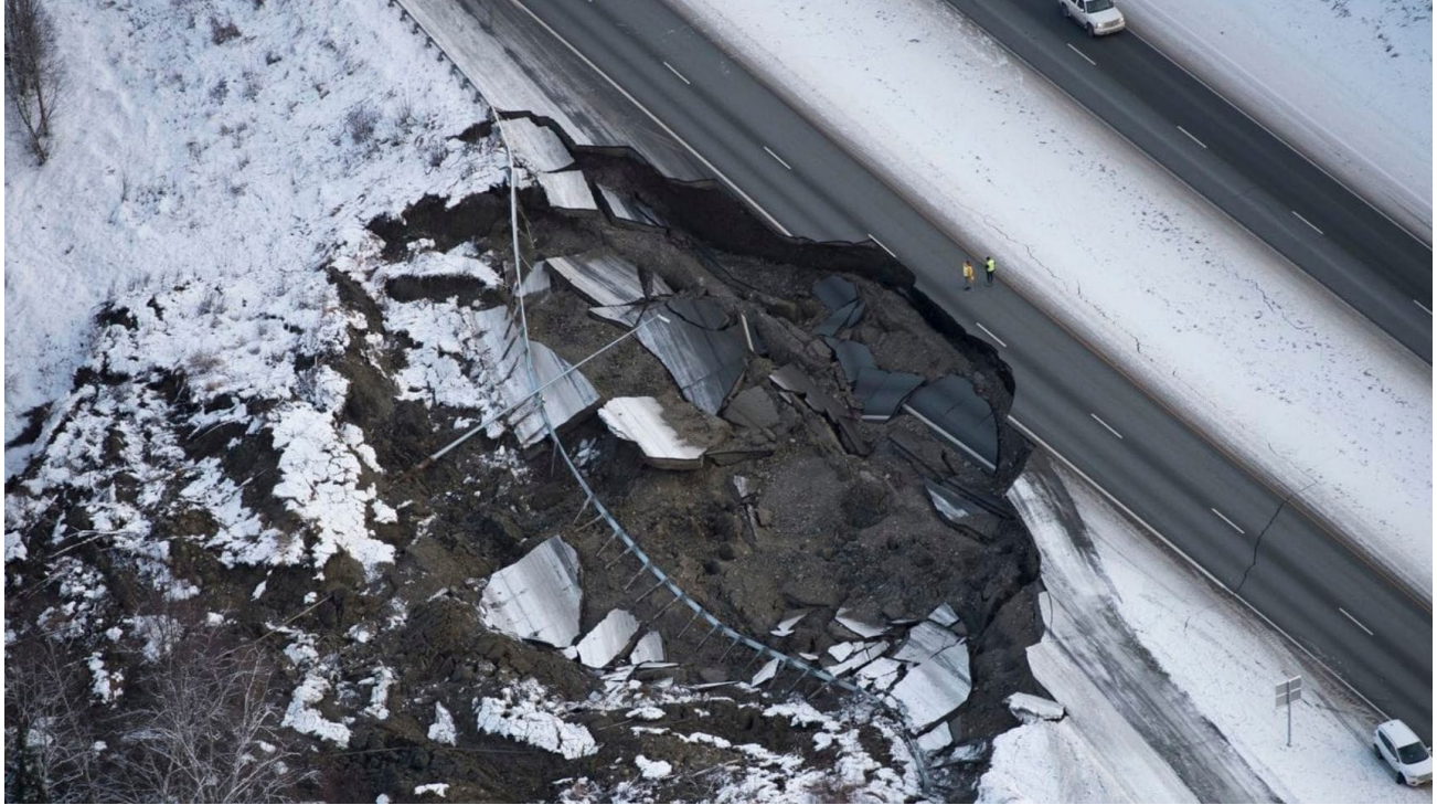
Figure 31: Aerial photo of the damage on the Glenn Highway near Mirror Lake in Anchorage, approximate location: 61.42° N, 149.42° W 36
