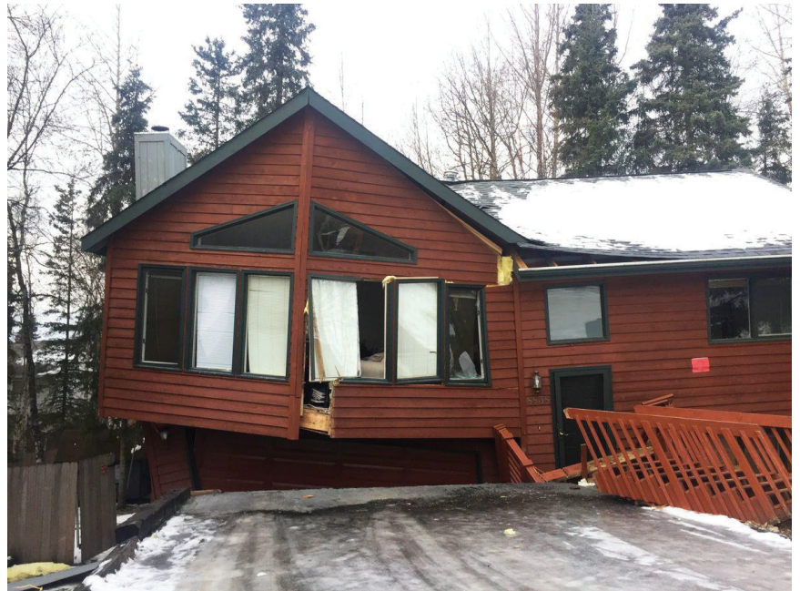
Partially collapsed two story home on Dome Circle in Eagle River
