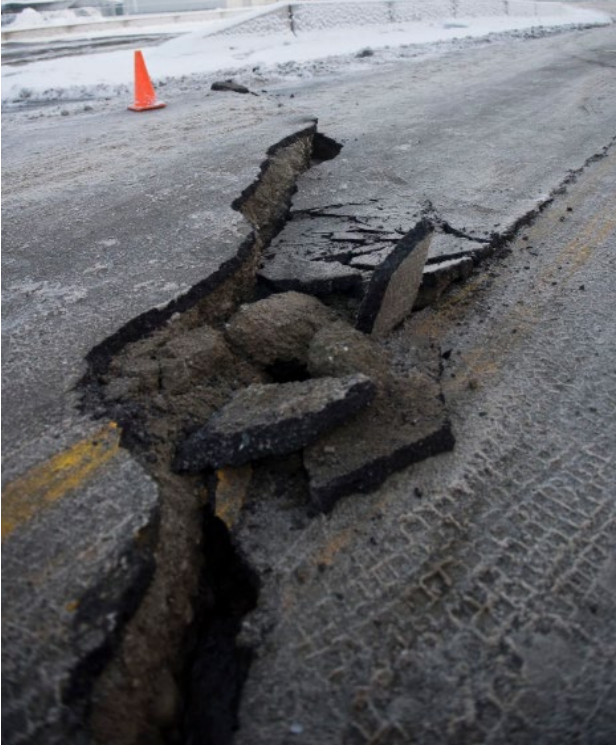
Figure 27: Cracks in Aircraft Drive near Lake Hood 30
