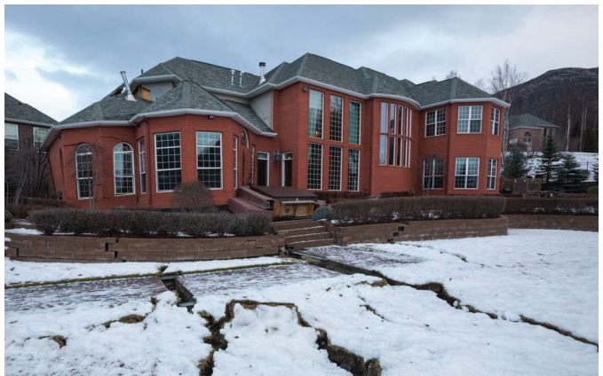
Severe structural damage
