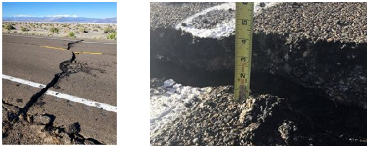
Figure 3. Pavement damage on U.S. Highway 95 between Las Vegas & Reno (Ritter, 2020)
