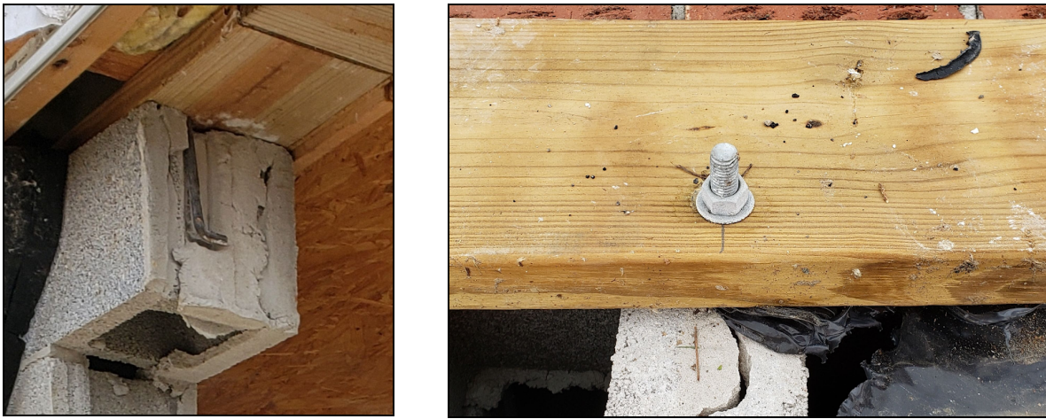
Figure 6.1.8. Bottom and top views of the typical sill plate to masonry stem wall connection. Here the sill plate is fastened to the stem wall with a j-bolt embedded in the head joint between adjacent empty CMU blocks.
