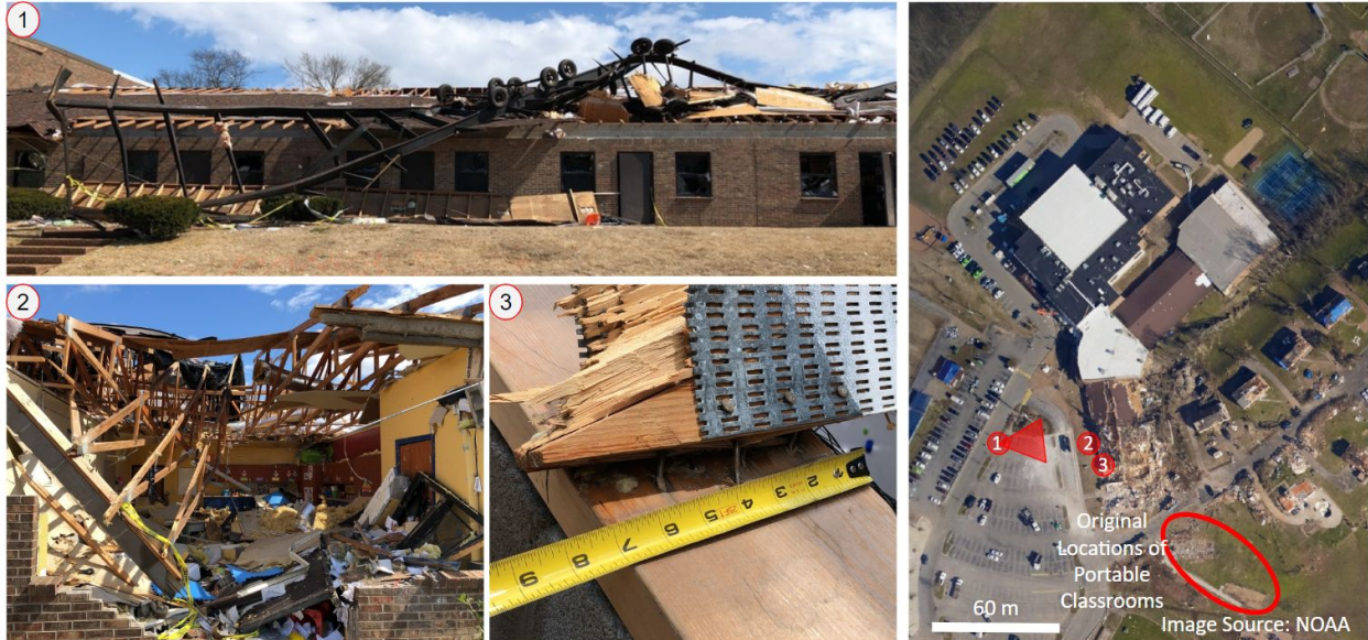
Figure 6.5.3. Representative images showing damage to the Donelson Christian Academy. (1) shows the frame of a portable classroom atop the south wing of the academy; (2) shows roof trusses still attached to the CMU bond beam with portions of the wall below collapsed. (3) shows a toe-nail connection between roof trusses and the 2x8 sill plate.
