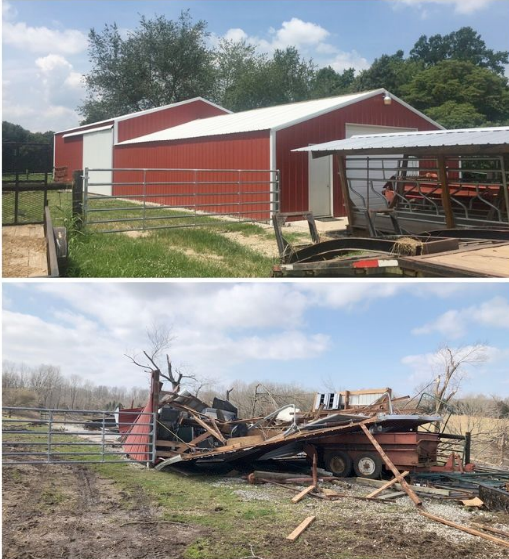
Figure 6.9.2. Before (top) and after (bottom) total collapse of metal barn (36.852421, -86.302735). Wood posts were set in the ground with no positive connection to the 4" thick concrete slab. Wind resistance would have been minimal. A few felled trees nearby.
