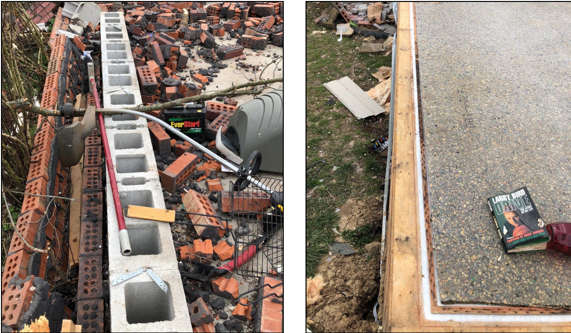
Figure 6.1.6. Common failures in Triple Crown subdivision with (left) foundation anchor straps installed into primarily ungrouted CMU block stem wall and (right) nailed sill plate attachment to floor system (two nails at 16-inches on-center).
