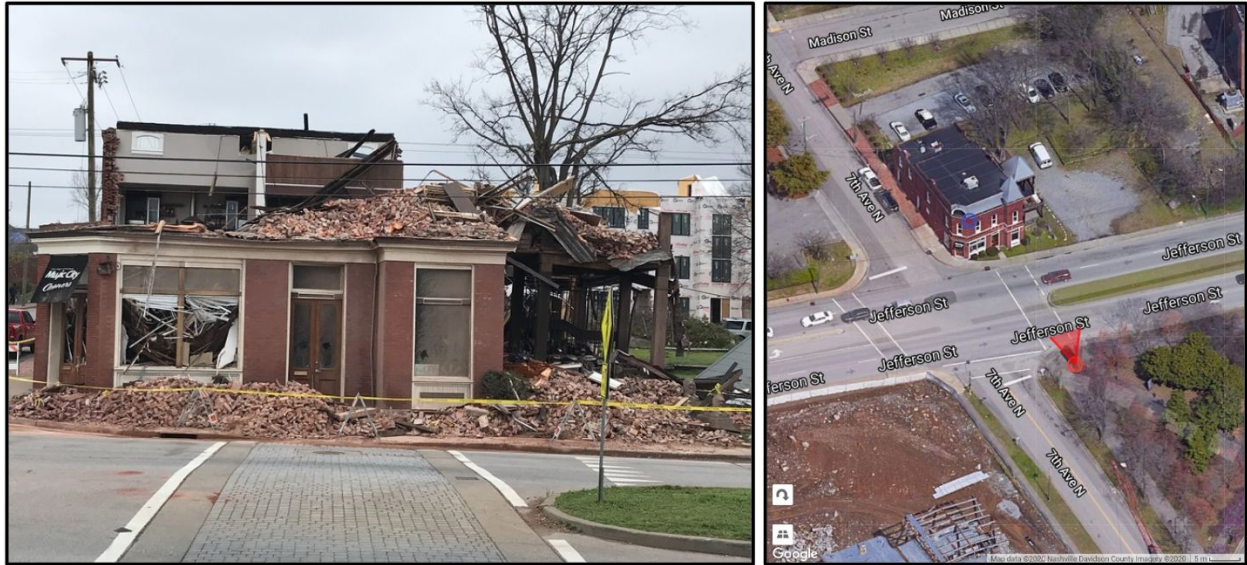
Figure 6.4.3. Destroyed office space in Germantown. Structure was built in 1910 and consisted of solid brick wythe walls (4 units thick) and heavy timber roof members.
