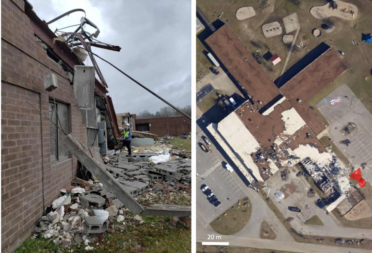
Figure 6.5.2. Collapsed CMU wall and roof beams at the south wing of Stoner Creek Elementary School. Steel I-beams and evidence of grouted and reinforced masonry were observed.
