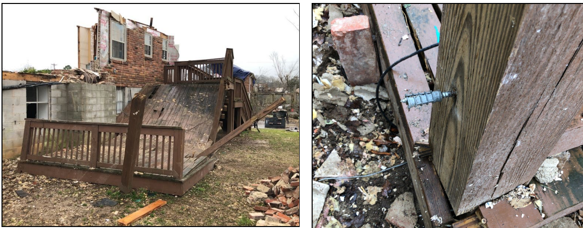
Figure 6.1.3. Several decks in Donelson that collapsed were fastened only to the brick veneer at the 2nd floor level.
