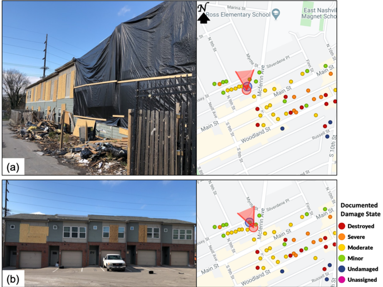
Figure 6.2.2. Cluster of townhome structures where (a) eastern exterior structure sustained moderate damage and (b) northern interior structure sustained minor damage. Photos taken March 10, 2020. Photo with map available on Fulcrum App.
