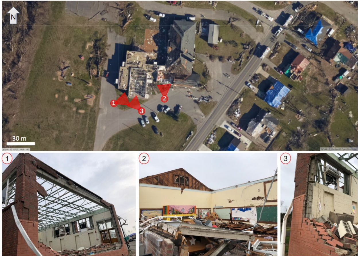
Figure 6.5.4. Observed damage sustained by the Donelson Chapel United Methodist Daycare Center, including (1) collapse of the end wall of the gymnasium with evidence of torsional racking of the building; (2) collapsed walls and complete roof removal in a classroom on the south side of the building; (3) clean failure of the CMU blocks near the corner of the gymnasium with no evidence of reinforcement or fully grouted cells in the wall below the bond beam. FAST noted very little fenestration damage on the east and north walls of the building.
