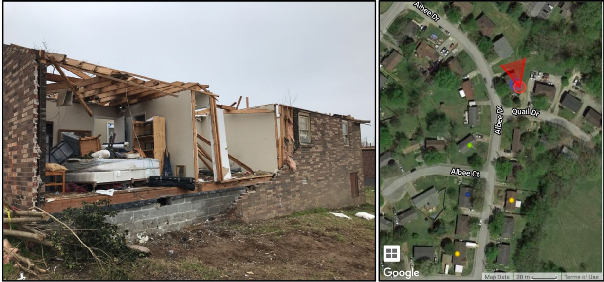
Figure 6.1.4. Single-story gable-roofed structure destroyed in Hermitage. Single-wythe brick facade on wood stud wall with Celotex wall sheathing. Home built in 1980. Photo taken March 12.
