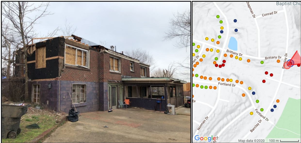
Figure 6.1.5. Typical 1980's construction in Barclay subdivision, with wood rafters, non-structural wall sheathing, and unreinforced masonry stem wall foundations with walk-out basements. Damage may have been enhanced by topographic features, with heaviest damage colocated with a valley that ran East-West through the area.
