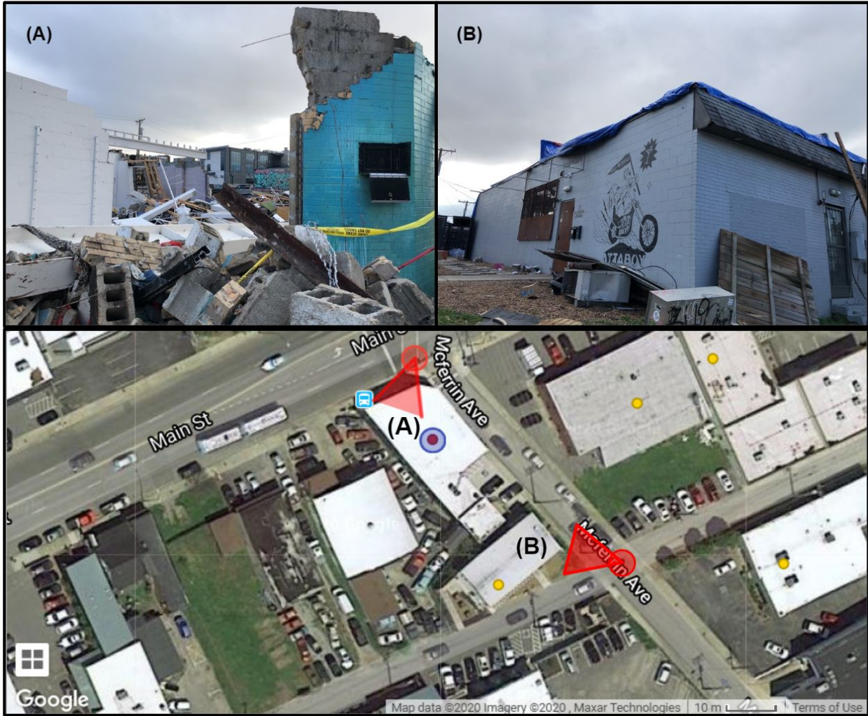
Figure 6.4.1. Damage to two adjoining buildings in the Five Points area of Nashville demonstrating the typical variability in performance observed in retail and office buildings. (a) a destroyed brick and concrete masonry block building with some steel framing members (built in 1950). Minimal reinforcement visible in the rubble, primarily existing in the bond beam; (b) a brick and concrete masonry block building with moderate damage to the roof cover (built in 1970).
