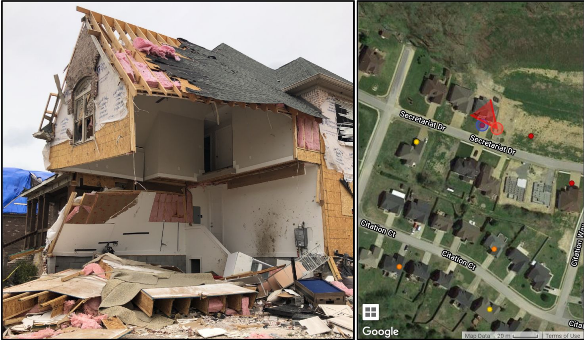
Figure 6.1.10. Garage wall failures were commonly observed, typically due to failure of garage doors, positive internal pressurization of the garage, and separation of walls at story joints, where discontinuities in the vertical load path exist.
