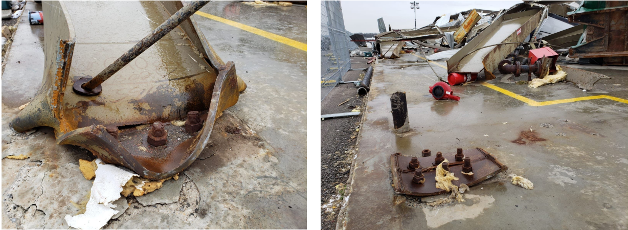
Figure 7.2.1. Baseplate damage and steel tension rupture in a collapsed hangar at the John C. Tune Airport.
