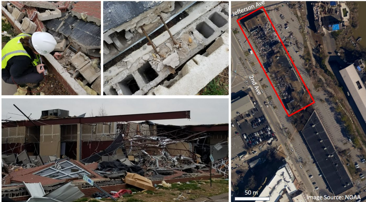
Figure 6.6.1. Total collapse of a government building in Germantown (GPS: 36.1740, -86.7822). The steel frame structure had infill CMU walls and brick veneers. Bent and snapped rebars were observed at the anchorage points.
