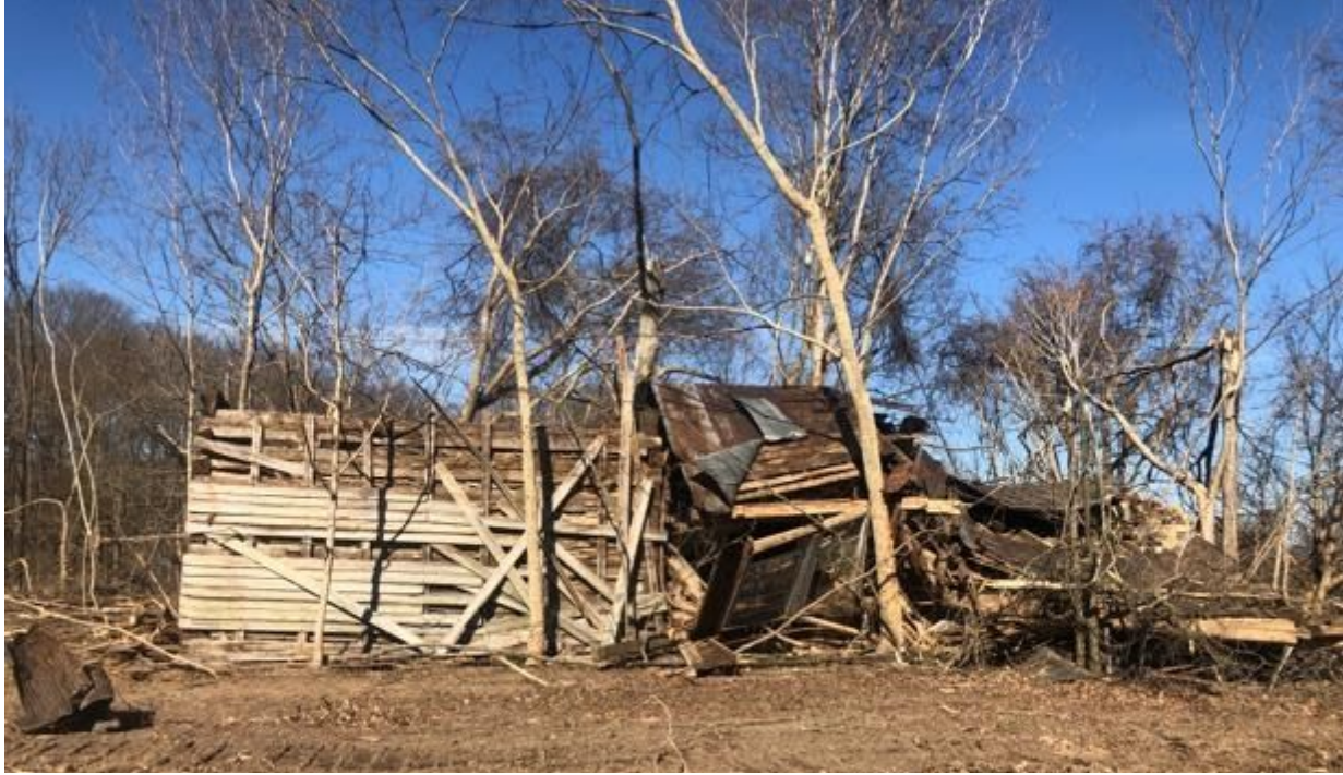
Figure 6.9.1. Destroyed wood-framed farm structure (36.854049, -86.295355) with a few fallen trees, but most still standing.
