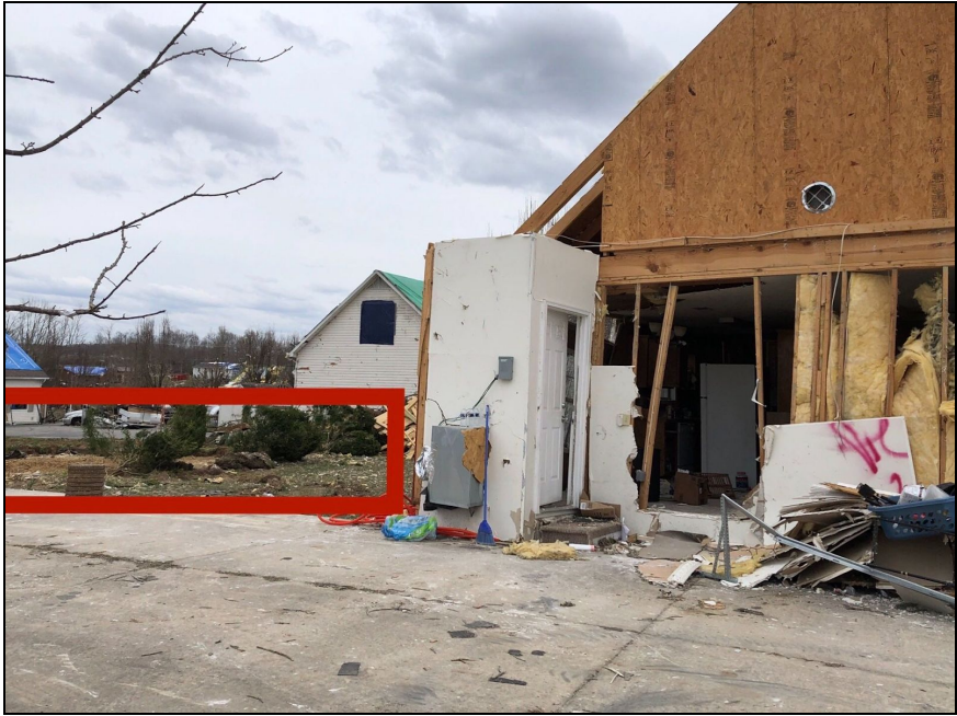
Figure 6.1.11. Anchorage failures were widespread, even when the majority of the home remained intact. This home slid approximately 50 ft off its foundation, and lofted over bushes. Red box indicates the original location of the home. The anchorage system present was the same as described previously - unreinforced masonry stem wall.
