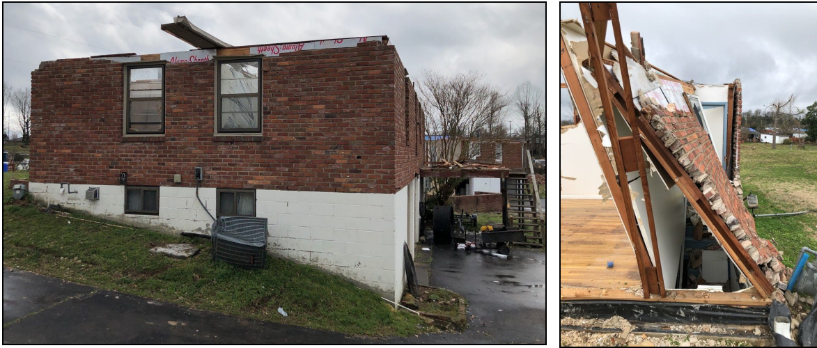
Figure 6.1.2. Typical construction and common failures in Donelson, with (left) a roof entirely removed, and (right) partial collapse of a wood-frame wall.
