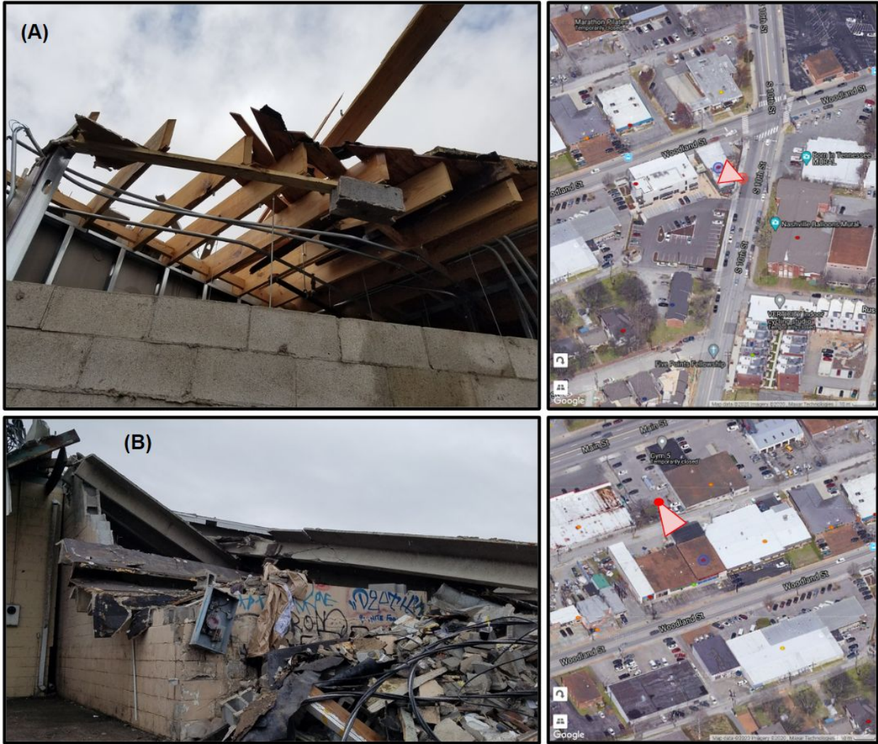
Figure 6.4.2. Additional failures noted in the Five Points area of Nashville: (a) Remnants of the bond beam and the wood top plate at a restaurant building originally constructed in 1935 with masonry block exterior walls, wood rafters, and cold-form steel interior walls; (b) Failure of prestressed concrete beams used in a small warehouse building constructed in 1962.
