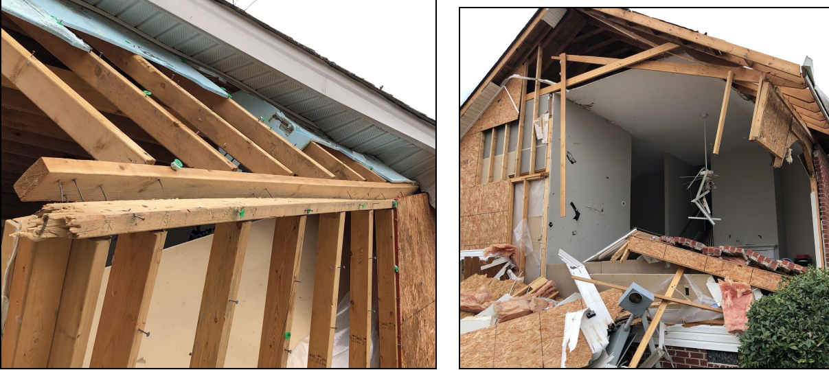
Figure 6.1.7. Gable end (left) and tall wall (right) failures occurring at the intersection of upper gable frame bottom plate and lower wall frame top plate, where sheathing is not overlapped and no lateral support is present.
