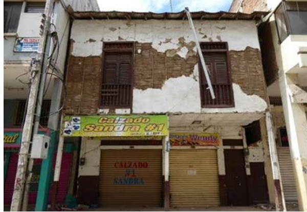
Figure 3.3. Non-engineered Bahareque House with substrate exposed by crumbled stucco ( Kaminsky 2023 ).
