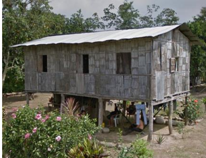
Figure 3.5. Non-engineered elevated wood house in Pasaje showing typical use of mixed lightweight materials as cladding elements and corrugated galvanized iron roof ( Google Earth Pasaje 2023 ).
