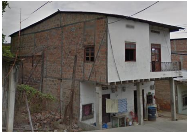
Figure 3.4. Two-story clay brick and timber building in Manabí. Note the timber framing on the unfinished face creates tall infill panels of irregular width ( Google Earth Manabí 2023 ).
