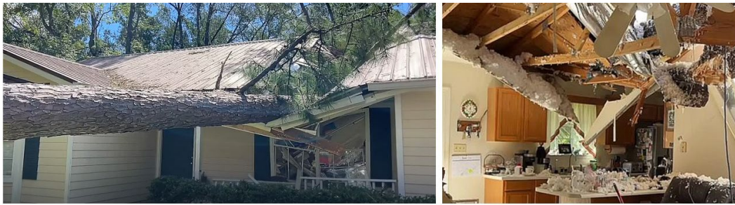
(a) Fallen tree on wooden roof structure
