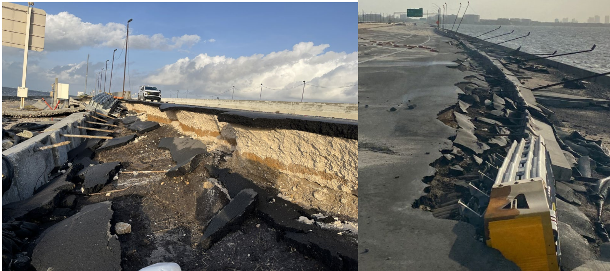
Figure 6.1. Asphalt pavement and soil subgrade washed away by Hurricane Helene storm surge (Source: FDOT West Central - Tampa Area ).
