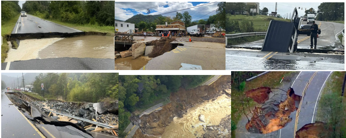
Figure 6.4. Geotechnical failures of roadways in North Carolina: (a) East Moore Street, (b) Hot Springs, (c) N.C. 211, (d) Hwy 105, (e) Rutherford County, (f) sinkhole (Source: CBS17 , RBP , Foxweather , 11Alive ).
