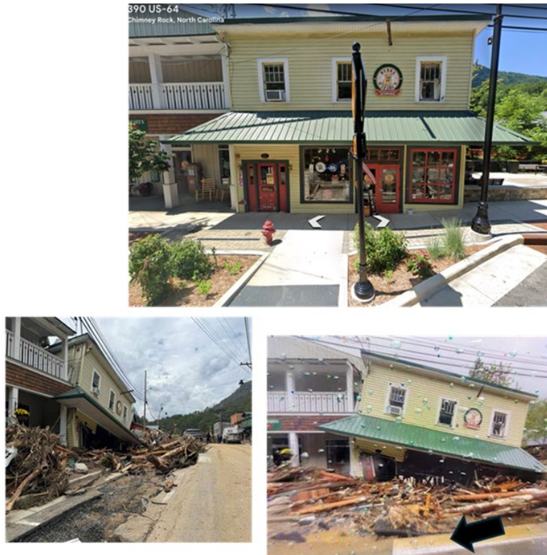
Figure 4.3.5. Two-story timber structure in downtown Chimney Rock collapsed due to fast-moving flood waters. The flow of the water along the graded road in front of the damaged building is also indicated with a black arrow (Source: Google Street View (top), bottom right from James Spann via Threads , bottom left WSOC-TV ).
