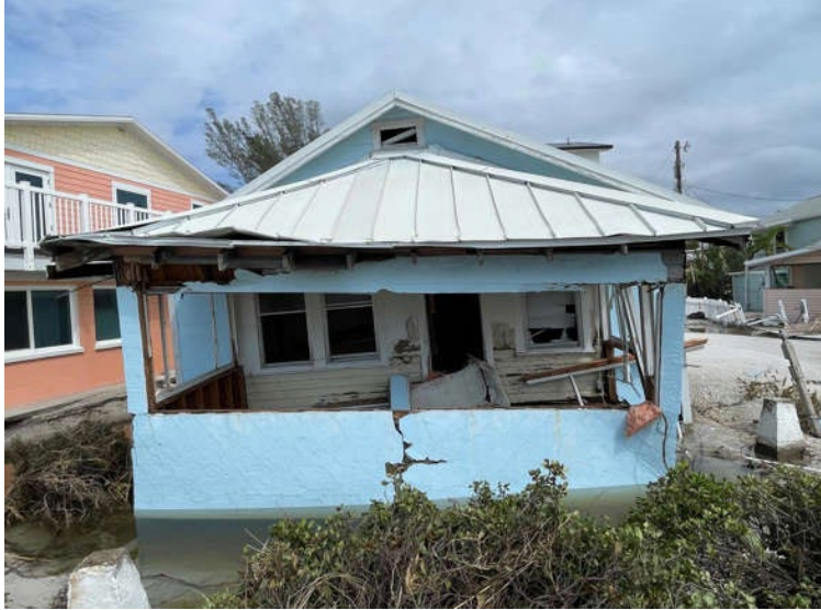
Figure 4.1.7. Dislocated non-elevated structure in Bradenton Beach on Anna Maria Island, FL (Source: Thomas Bender ).
