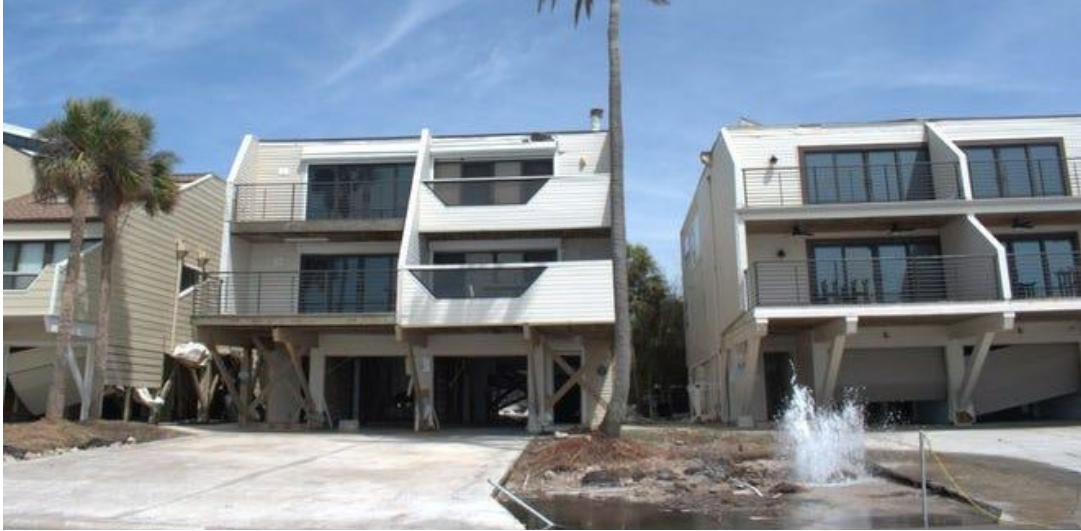
Figure 4.1.3. Damage to non-structural elements at ground floor of elevated buildings in Siesta Keys, FL (Source: Christian Casale ).
