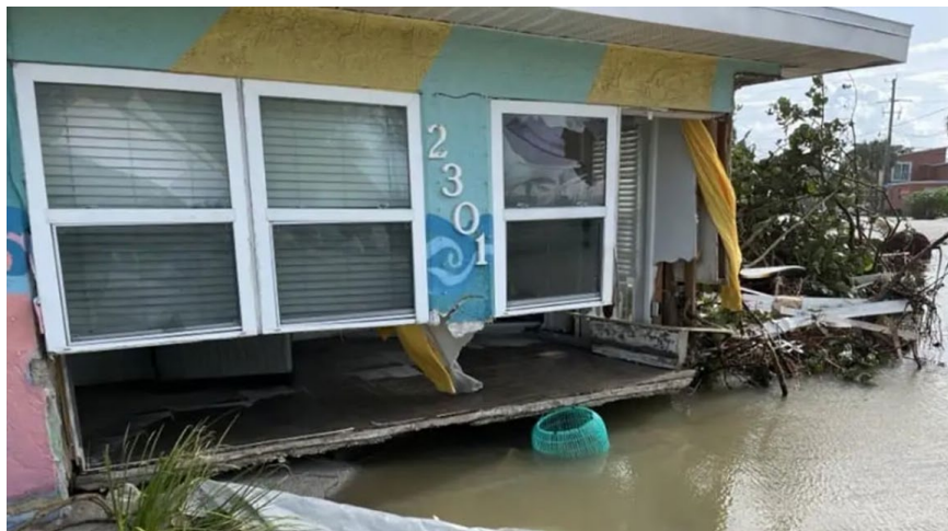
Figure 4.1.8. Non-elevated building with damaged exterior walls and foundation scouring in Manatee County, FL (Source: Manatee County Government ).
