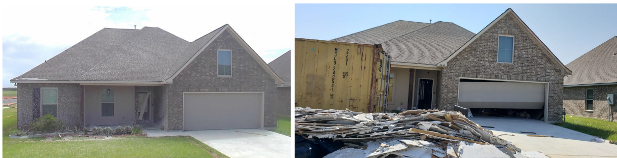
Figure 4.7. Progression of garage door damage on a home near the Chennault International Airport between hurricanes: (left) undamaged following Hurricane Laura and (right) buckled following Hurricane Delta, also note interior damages from Hurricane Laura as evidenced by debris pile at curb (Credit: FAST-1).
