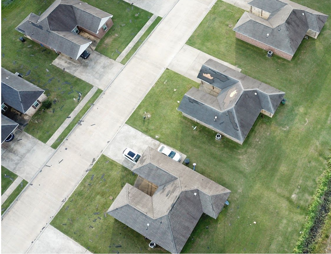
Figure 4.4. Typical roof cover damage levels in older (~2005) residential cluster in Abbeville (Credit: FAST-1).
