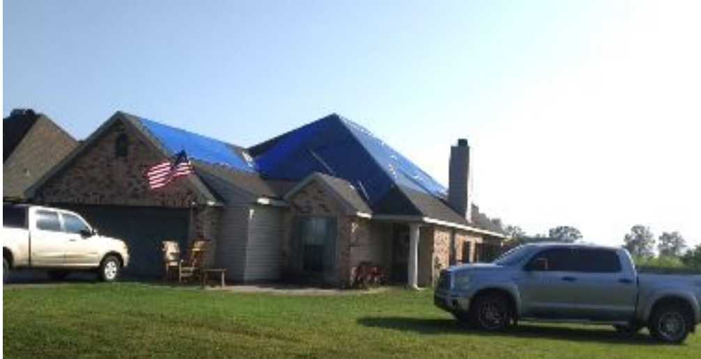
Figure 4.2. Example of roof damage to house at end of block in Youngsville (Coordinates: 30.102928, -92.056204) (Credit: FAST-2).
