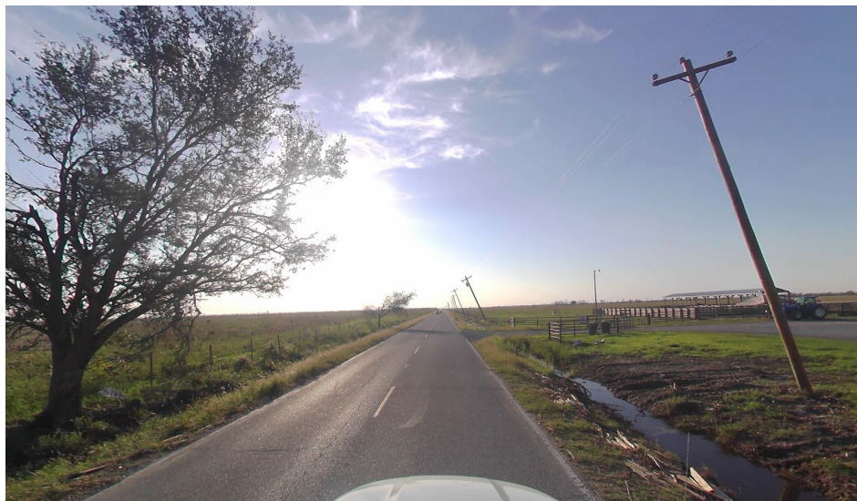
Figure 4.9. Power poles installed after Hurricane Laura already leaning severely along LA-27 (Credit: FAST-1; GPS: 30.0722, -93.1192). This location was subjected to approximately 85 mph peak gust wind speeds and 15-20 inches of rainfall.
