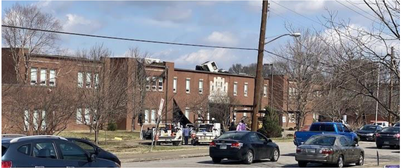
Figure 4.17. Meigs Middle Magnet School Damage (GPS: 36.176388, -86.760729). Source: Nashville Metro Schools .
