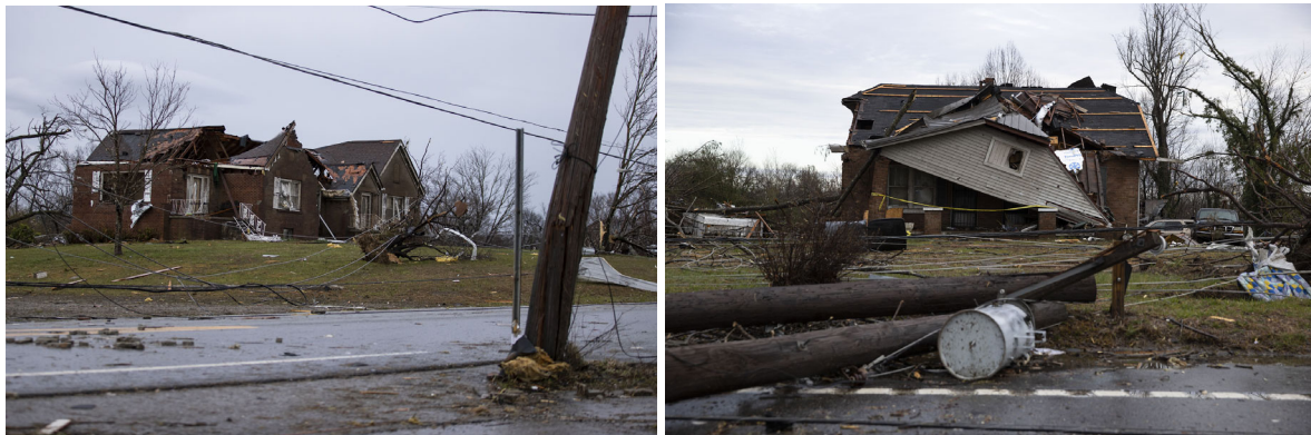
Figure 4.5. Single-family home damaged by the tornado in Cookeville, TN ( House Cookeville )
