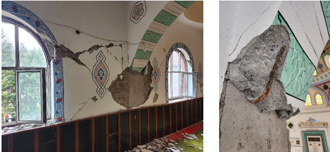
Figure 4.11. Damage to Saridere village mosque in Golyaka at 40.819°N, 30.994°E. (Source: Demir).
