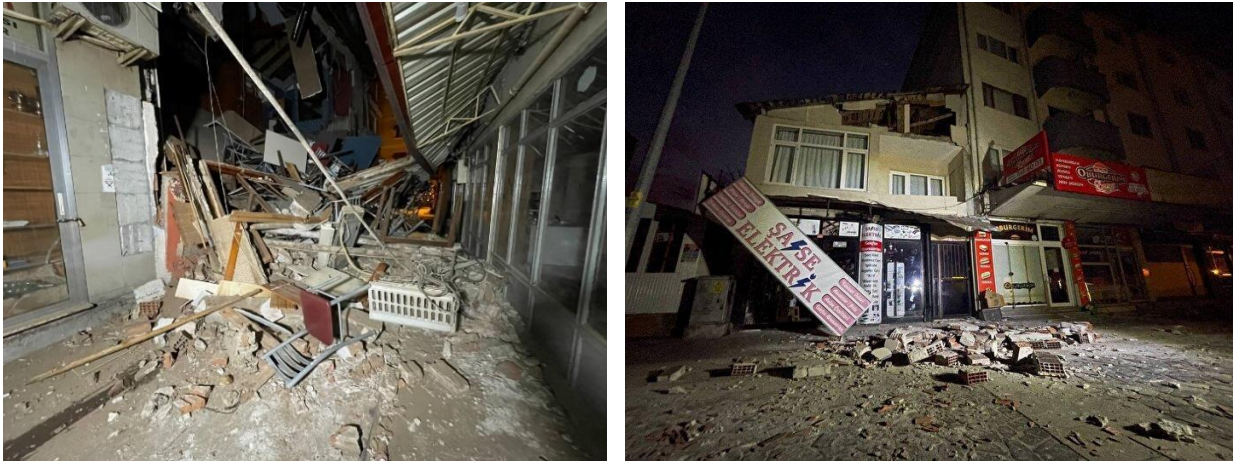
Figure 1.5. Damage in shopping areas and store fronts (Source: Yenisafak (2022)).
