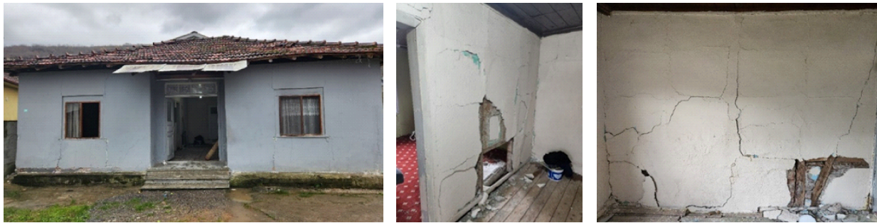
Figure 4.9. Damage in timber-masonry load-bearing walls of a building in Golyaka (coordinates: 40.824°N, 31.001°E) (Source: Demir).
