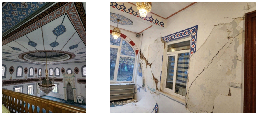
Figure 4.10. Damage on the dome (left) and walls (right) of Kiremitoğlu mosque at 40.838°N, 31.145°E. (Source: Demir).
