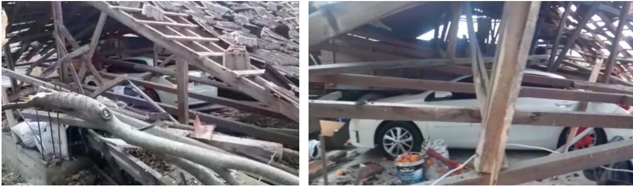
Figure 1.7. Damage to a parked vehicle due to damage to a non-engineered parking structure (Source: Arslan).
