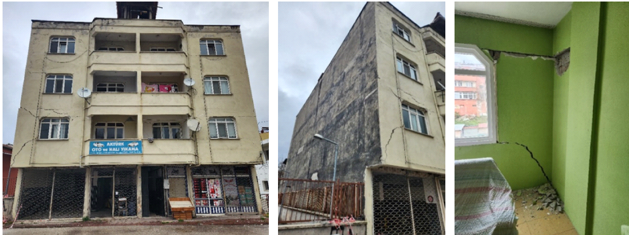
Figure 4.6. Damage to an RC apartment building in Golyaka at 40.779°N, 30.989°E (Source: Demir).
