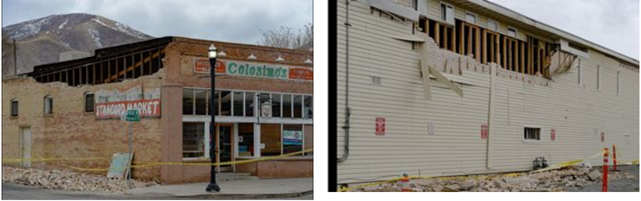
Figure 5. Brick veneer wall damage in Magna (The Salt Lake Tribune, 2020)
