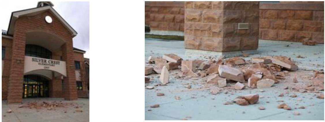
Figure 6. Front façade damage experienced in Silver Crest Elementary resulting in masonry debris striking the ground in front of the main entrance (Valley Journals, 2020; Deseret News, 2020)
