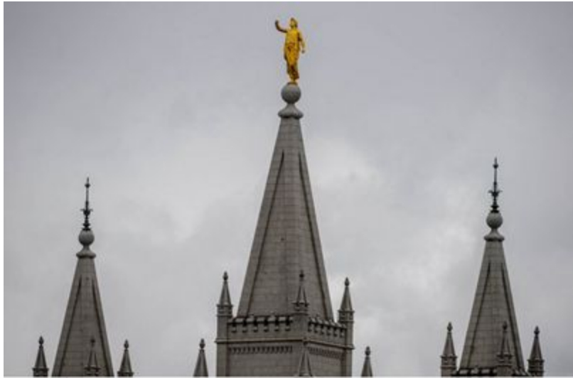
Figure 7. The statue of Moroni at the top of the Salt Lake temple damaged during the earthquake (The Salt Lake Tribune, 2020)
