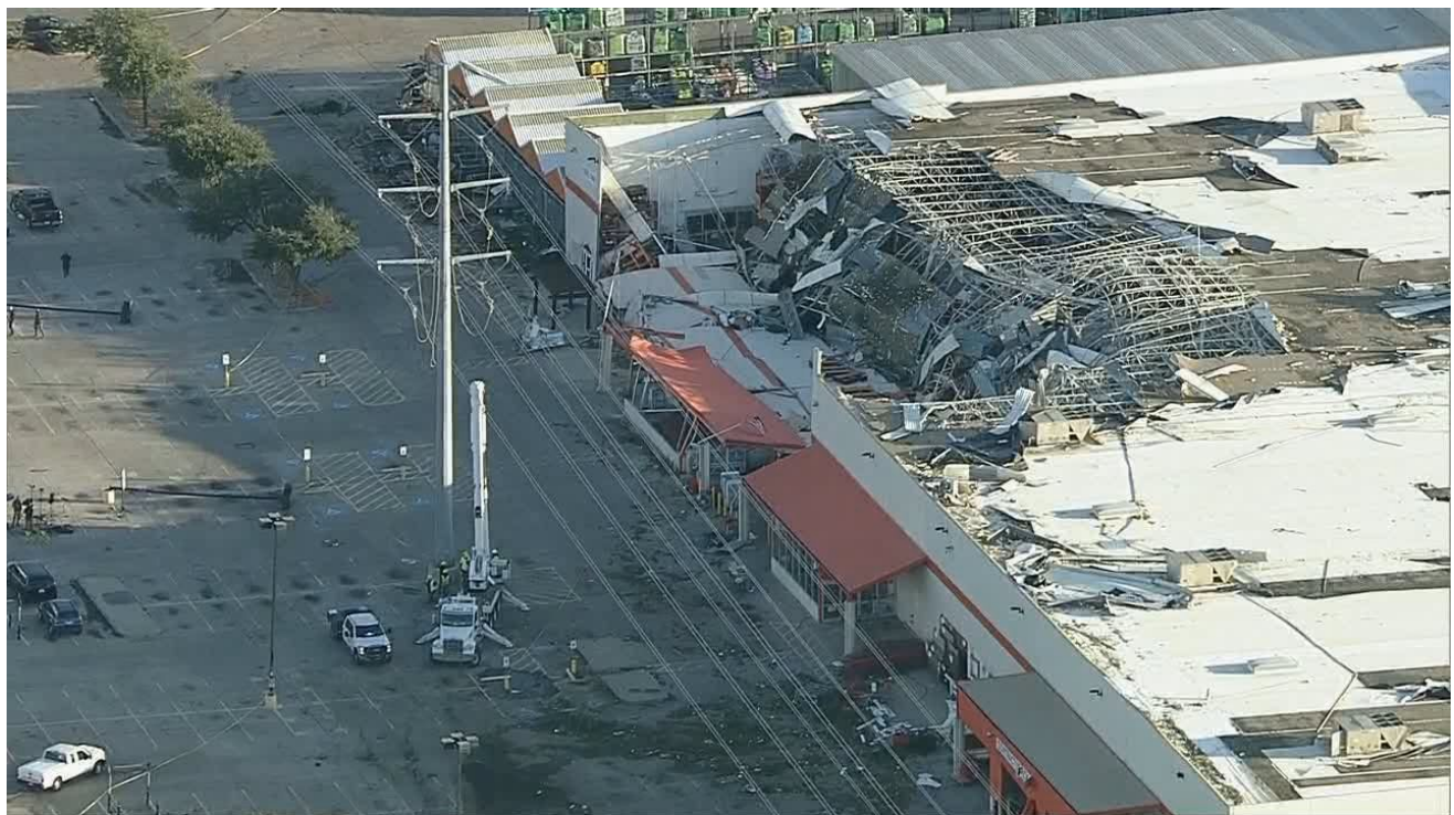
Figure 10. Aerial view of damage to the Home Depot (Lat: 32.906987; Long: -96.764696) (Sources: Fox 4 News ).
