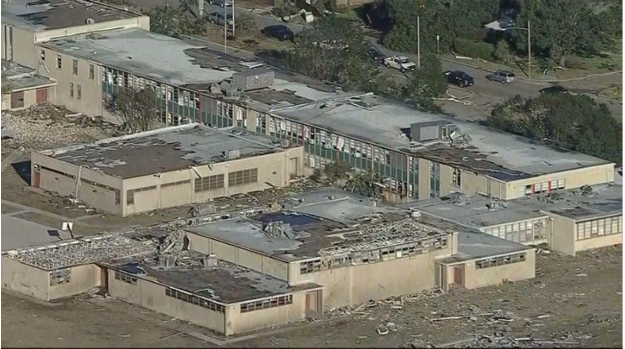
Figure 4. Cary Middle School with severe damage to cladding and fenestration and some structural roof damage (Source: WFAA TV ).
