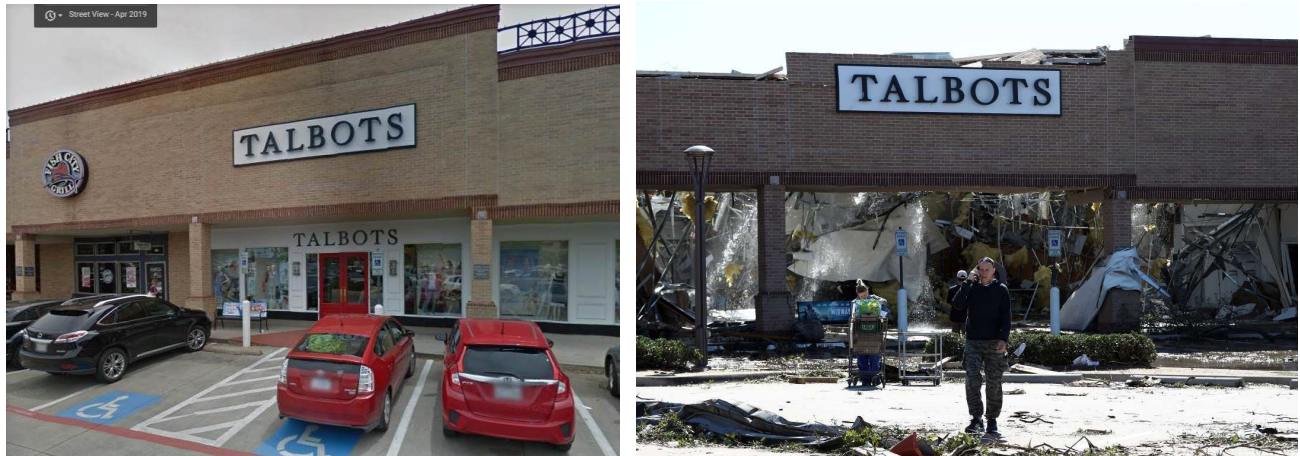
Figure 9. Google Street View before tornado and roof failure after tornado at Preston Royal Shopping Center (Lat: 32.8935N; Long: 96.8023W) (Sources: MSN 2019, Ronald Martinez/Getty Images)
