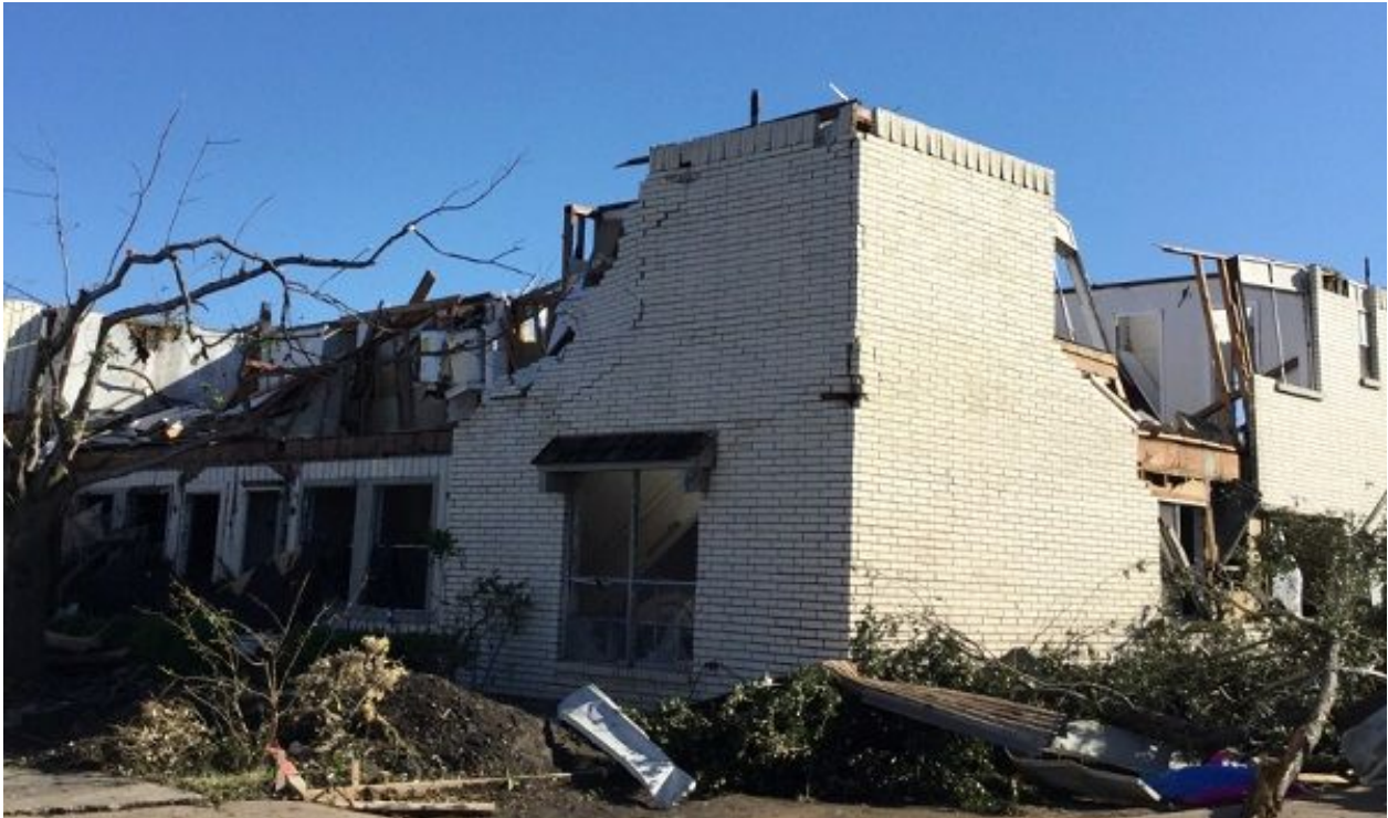
Figure 13. Damage to apartments located in Walnut Hill (Source: NWS Fort Worth ).
