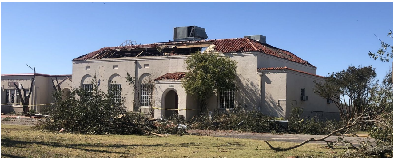
Figure 5. Walnut Hill Elementary School with structural roof damage (Source: Fox 4 News ).
