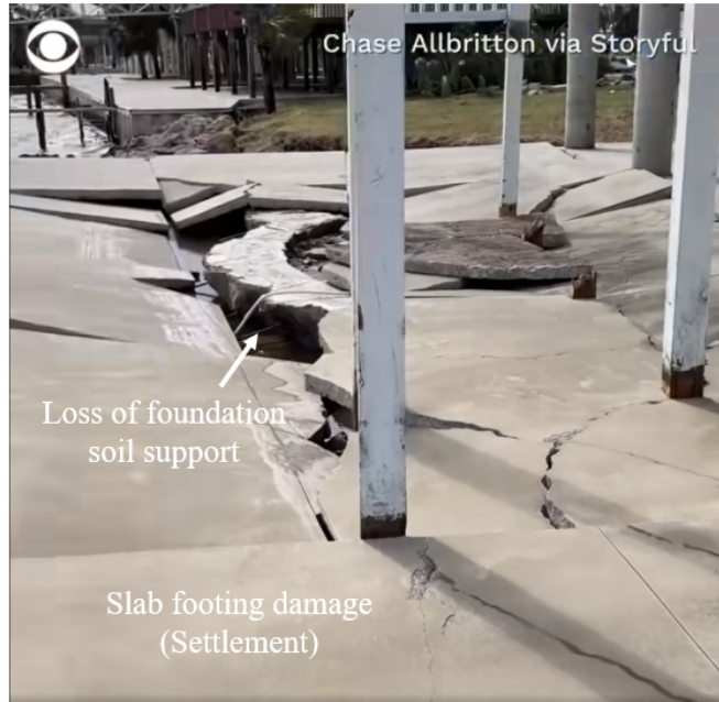
Figure 6.1. View of Shallow foundation (slab footing) damage of residential structure showing severe washout (Source: Chase Allbritton via Storyful ).
