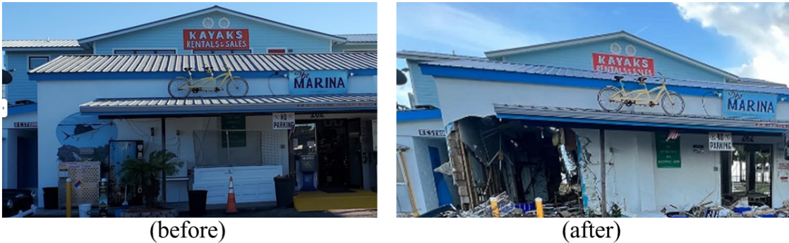
Figure 4.1. Collapse of concrete masonry wall of commercial building in Horseshoe Beach, FL (Source: Vic Micolucci via Facebook ).
