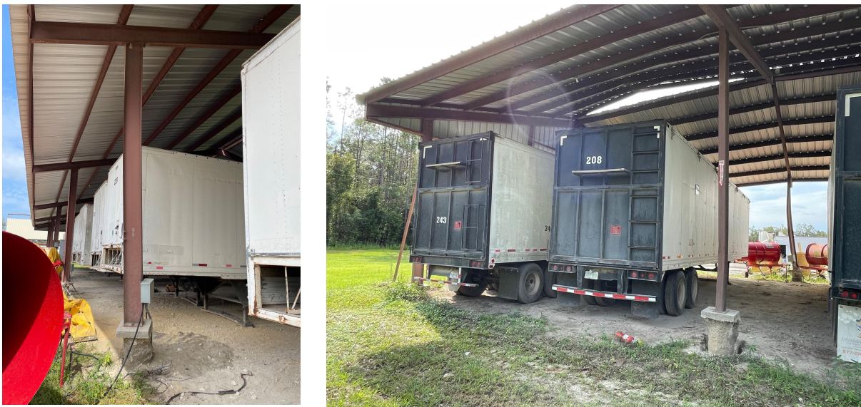
Figure 6.2. Column-foundation pull-out capacity failure. (Source: UF Building Performance Observation Survey on 2023-hurricane-idalia-vast design safe slack channel )
