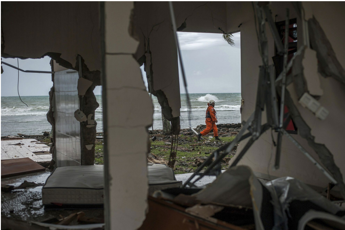
Figure 22: Damage to masonry structure on shoreline (Credit: Associated Press / Fauzy Chaniago)
