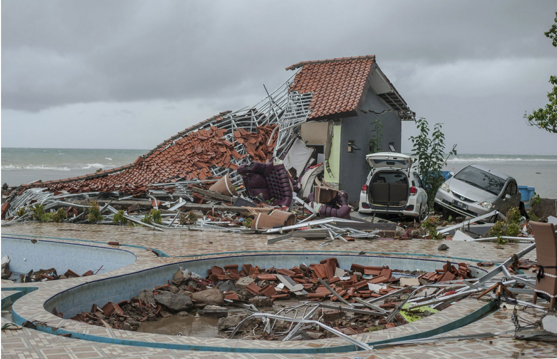
Figure 21: Damage to masonry structure on the shoreline (Credit: Associated Press / Fauzy Chaniago)
