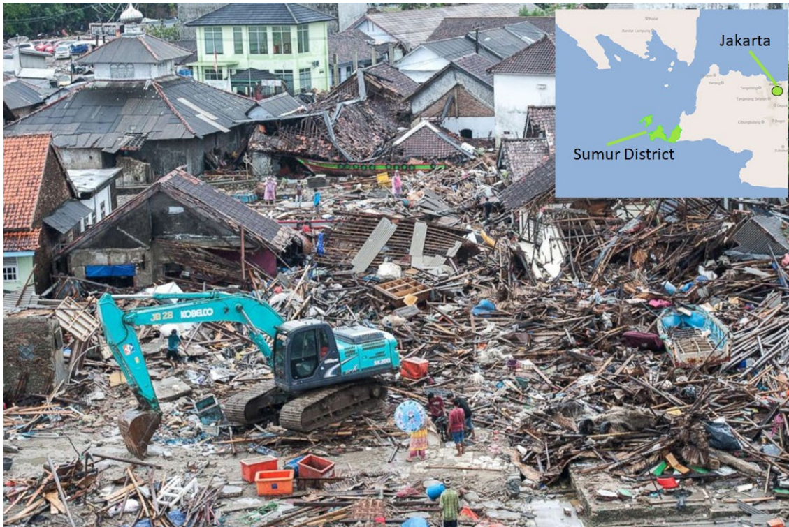
Figure 19: Debris clean-up underway in the Sumur district of Pangdeglang, Banten Province, Indonesia. Photo by Veri Sanovri/Xinhua via Newscom and ABC News .
