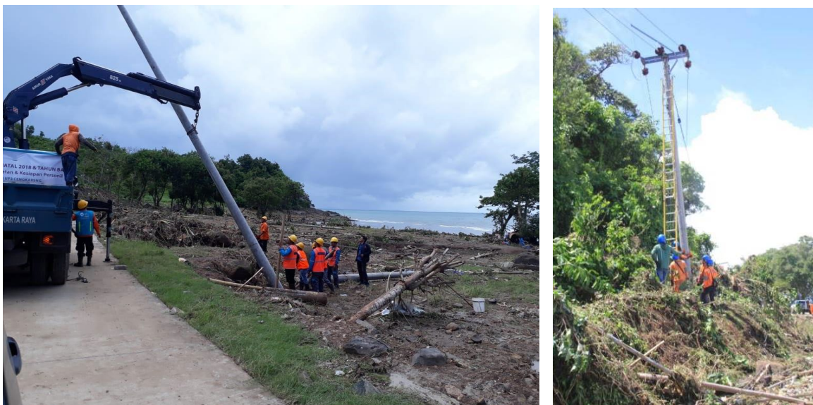
Figure 35: Crews installing new power transmission line poles the day after the tsunami (Source: https://twitter.com/Sutopo_PN/status/1077091875448737792 )
