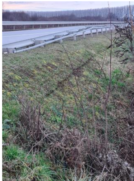
Figure 5.19. Partial lateral ground slide close to Brest Bridge (source: Nenad Bijelić).
