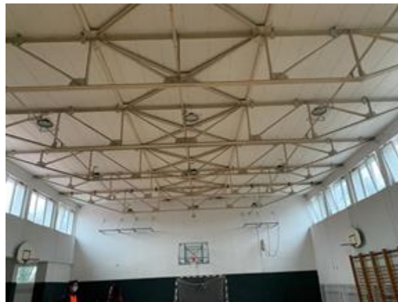
Figure 4.58. Sports hall at Elementary School Dragutin Tadijanović in Petrinja (source: Nenad Bijelić and Damir Lazarević).
