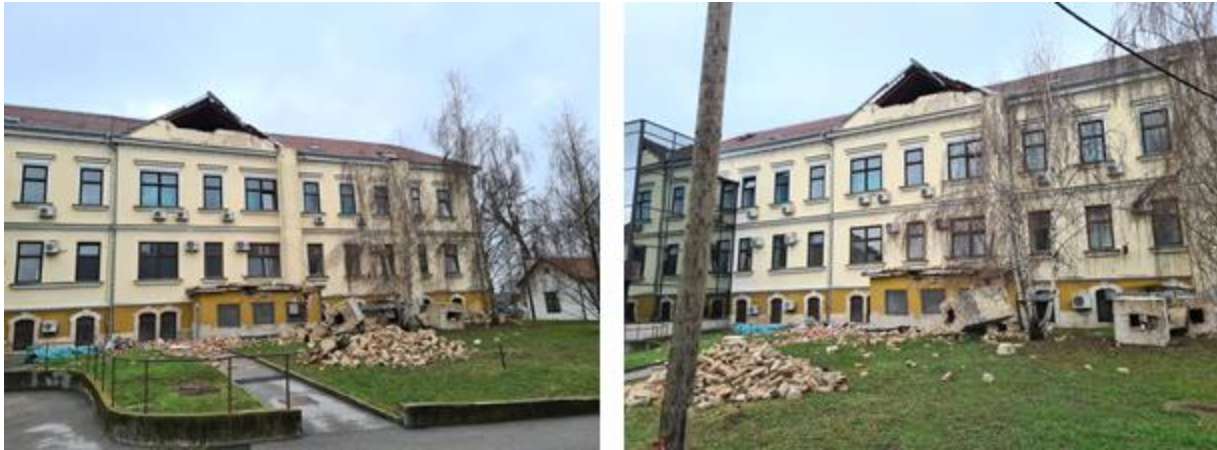
Figure 4.119. Fallen chimneys and gable end wall in hospital Dr. Ivo Pedišić in Sisak (source: Nenad Bijelić and Marko Bartolac).
