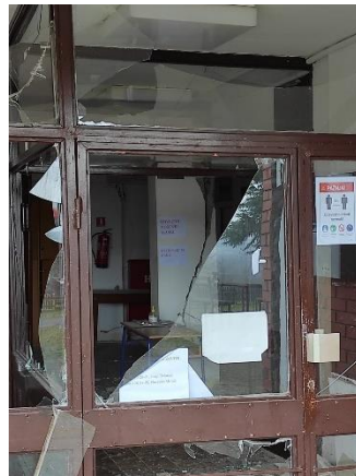
Figure 4.64. Broken glass in entryway door (source: Nina Čeh).
