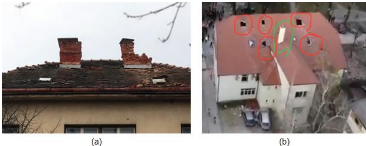
Figure 4.118. Damaged chimneys (source: (a) Getty and (b) Twitter 2021).
