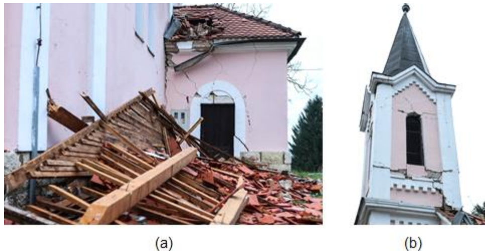
Figure 4.103. Church in Mračaj, near village Majur: (a) heavy cracking in the interface between adjacent shorter unit and the main nave (source: Marko Pripic/PIXSELL) and (b) severe cracking of the bell tower (source: Marko Pripic/PIXSELL).
