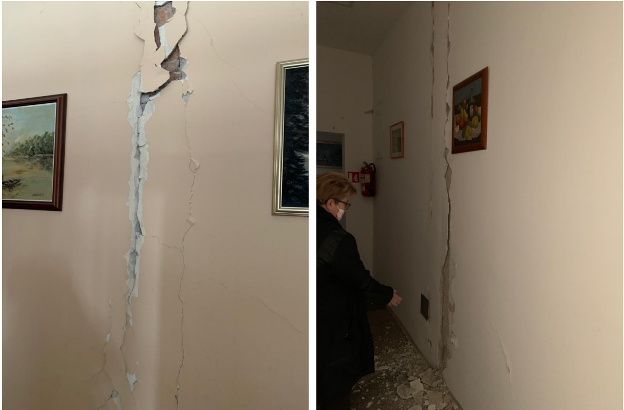
Figure 4.33. Cracks along the interface between a masonry infill and an RC column (source: Damir Lazarević).
