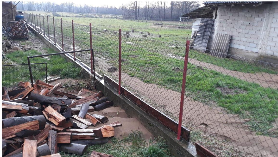
Figure 6.18. Crack between two houses due to liquefaction (45.4540, 16.2611). The line of liquefaction spreads through several yards and under houses, Brest Pokupski (source: Tomislav Ivšić, Sonja Zlatović, Igor Gukov).
