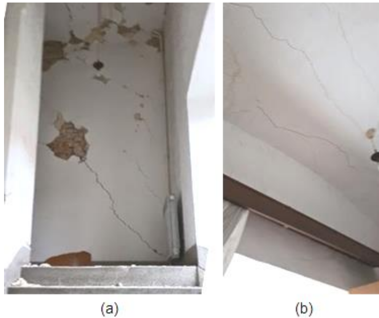
Figure 4.77. Details of Town Hall building damage: (a) In-plane shear crack in a load-bearing wall in the transverse direction (source: Nenad Bijelić) and (b) Cracking of a masonry vault, indicating a potential formation of an arch mechanism (source: Nenad Bijelić).
