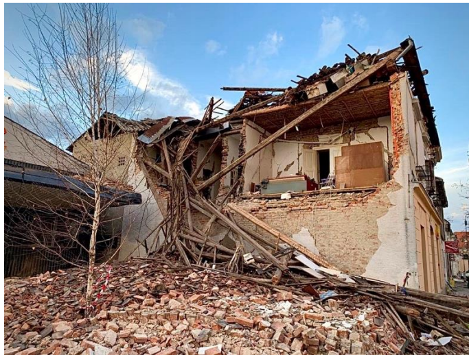
Collapsed unreinforced masonry building on Strossmayer St. in Petrinja, Photo by Damir Lazarević
