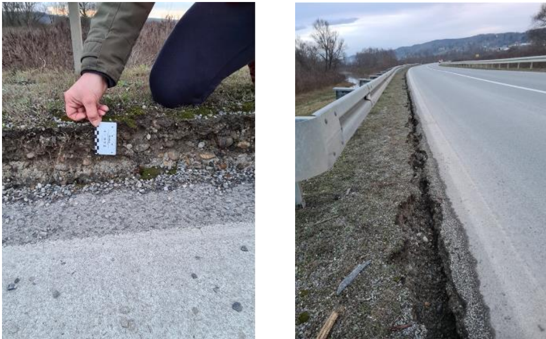
Figure 5.17. Ground failure of a road close to Brest Bridge (source: Nenad Bijelić).
