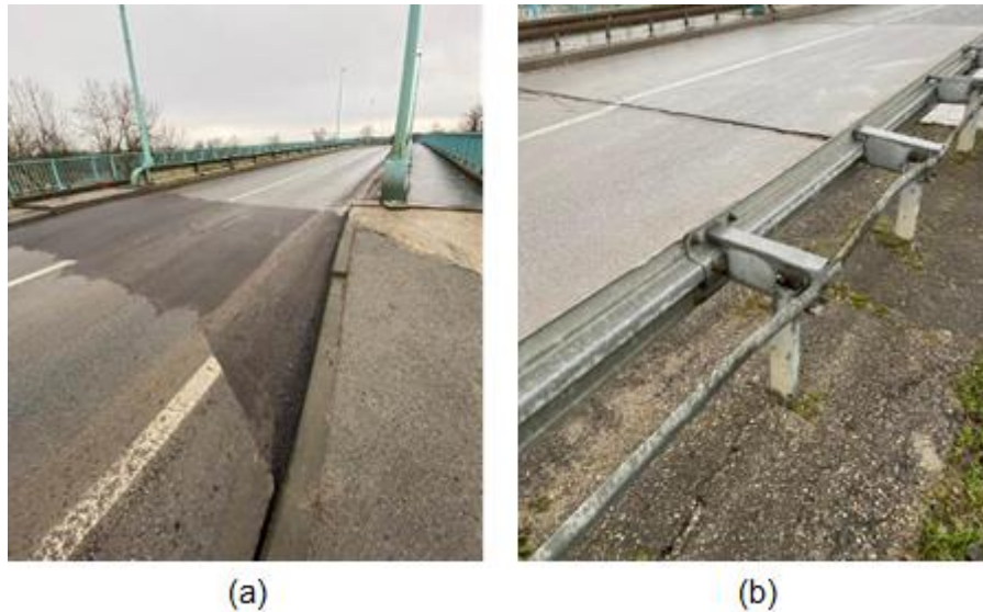
Figure 5.7. Asphalt at right-hand side abutment (a) and asphalt at left-hand side of abutment (b) of the Brest Bridge (source: Mate Baričević).
