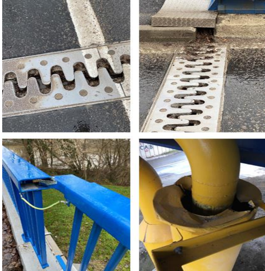
Figure 5.12. Damage due to lateral displacement of the bridge relative to the slab approach, Galdovo Bridge (source: Mate Baričević).
