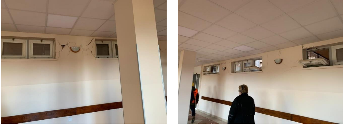
Figure 4.31. Shear cracks in infill masonry walls of the retirement home in Petrinja (source: Damir Lazarević).
