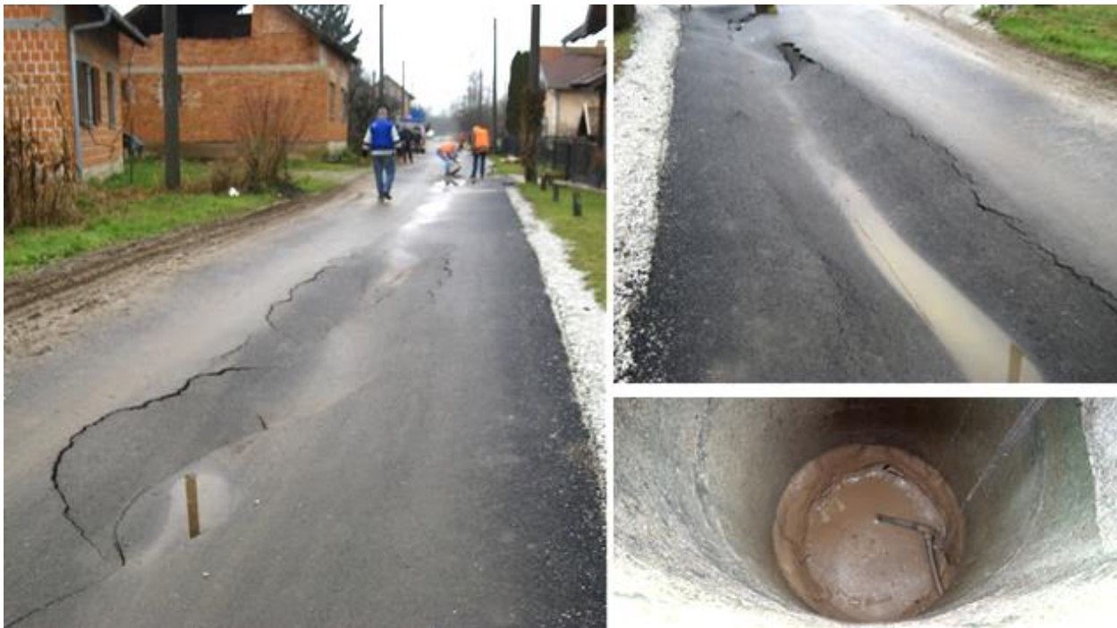
Figure 6.20. Settlement of the road along which the sewage system was renovated recently. It is possible that the material around the pipes was not compacted properly during construction, but liquefaction might have been the main reason for the settlements as a nearby well (45.4562, 16.3164) was filled with sandy material. Nova Drenčina, Drenačka ulica. (source Sonja Zlatović).
