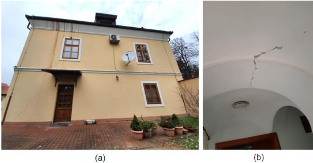
Figure 4.87. St. Lawrence parish church rectory that was built in 1783 in late Baroque style: (a) Façade shows diagonal cracks in the piers. Overall response was good. It is possible that small openings to the total area of walls had a beneficial effect. Chimneys collapsed. (b) Cracked vault inside the house (source: Marko Bartolac).
