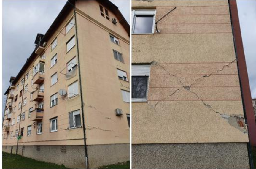
Figure 4.21. Damage to Building 4, a 5-story building with a vertical extension (source: Marko Bartolac).
