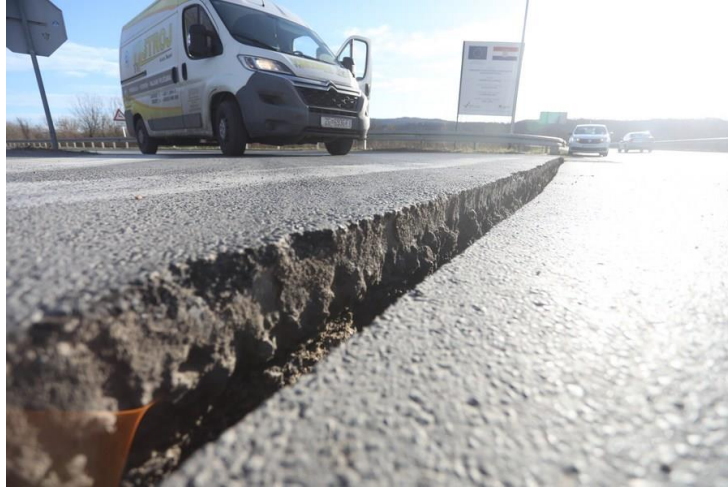
Figure 5.14. A major fissure in the road in Sisak was observed after the December 29, 2020 earthquake (source: Marin Tironi/Pixsell via Xinhua).
