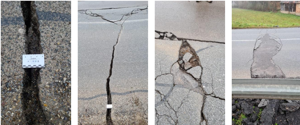
Figure 5.15. Damage to roads in Brest, north of Petrinja (source: Nenad Bijelić).
