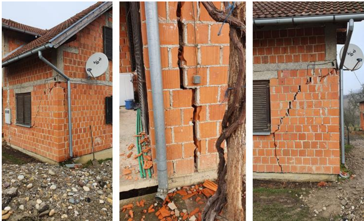
Figure 4.13. Damage of a partially confined masonry building in the Graberje village due to the absence of RC tie-columns at wall intersections. The damage is in the form of wide vertical cracks along the wall intersection and stepped shear cracks expanding from the ground to the second floor slab (source: Hrvoje Ljubojević, Tenzor d.o.o).
