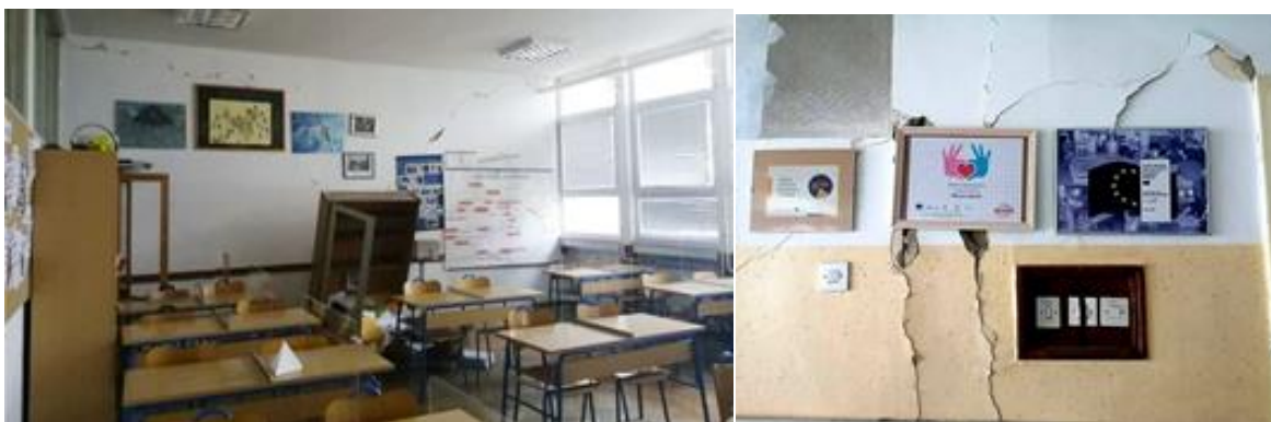
Figure 4.60. Earthquake damage in Glina High School (source: Facebook Page - Srednja škola Glina).
