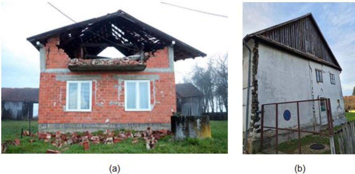
Figure 4.9. Performance of gable walls: (a) collapsed gable wall in a partially confined masonry building (with discontinuous RC tie column) and without a RC ring beam along the wall-to-roof interface (source: Sanjin Strukic/Pixel) and (b) good performance of a gable wall in a form of light-weight wooden panel (source: Nenad Bijelić).
