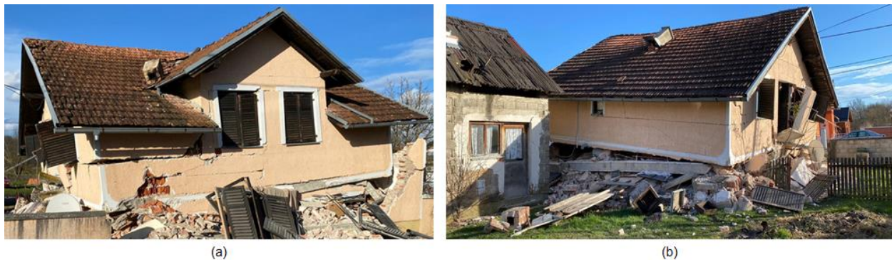
Figure 4.14. Collapsed partially confined masonry building in Prekope village, close to Glina (sources: (a) Damir Sencar AFP Getty and (b) Krešimir Micić).
