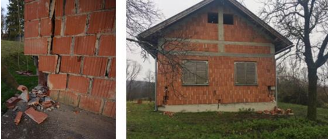
Figure 4.12. Damage of a partially confined masonry building due to the absence of RC tie-columns at the ground floor level (sources: J. Miskovic/Cropix (left) Hrvatska Danas 2021 (right)).
