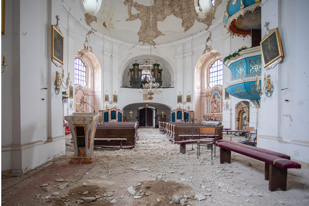
Figure 4.94. Interior of the Church of St. Marije Magdalene in Sela. Extensive cracking visible in the dome, as well as plaster detachment (source: Facebook Page Sisačka biskupija).
