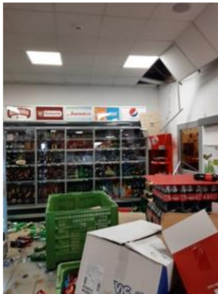
Figure 4.27. Damage to hung ceiling assembly in the KTC supermarket (source: Sonja Belovarac Radenovic).
