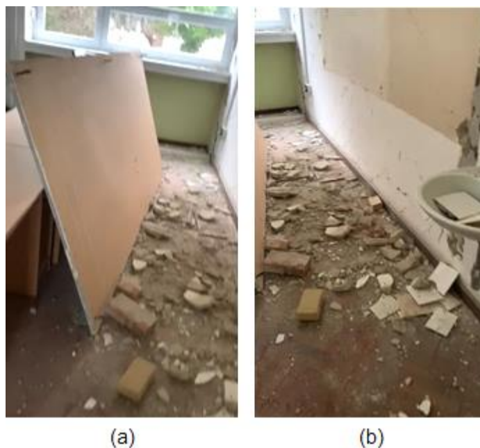
Figure 4.113. Detachment and collapse of the school board in one classroom (Faculty of Education - Učiteljski fakultet) (source: Marko Bartolac).
