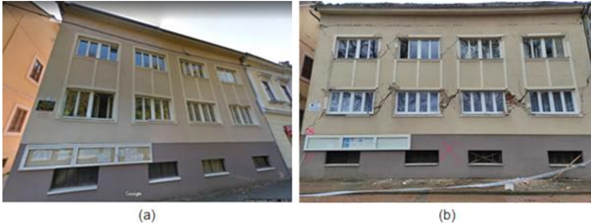
Figure 4.80. Chamber of Crafts building: (a) before the earthquakes (source: Google Maps) and (b) after the earthquakes. All central piers developed deep in-plane shear cracks. A wide continuous horizontal crack extends throughout the façade at the roof level (source: Nina Čeh).
