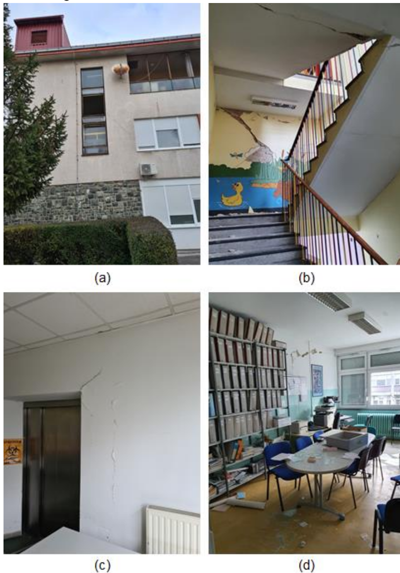
Figure 4.41. Building #1: (a) external view, (b) diagonal cracks in masonry infills, (c) cracks near elevator shafts, and (d) horizontal cracks along masonry-concrete joints (source: Nenad Bijelić).
