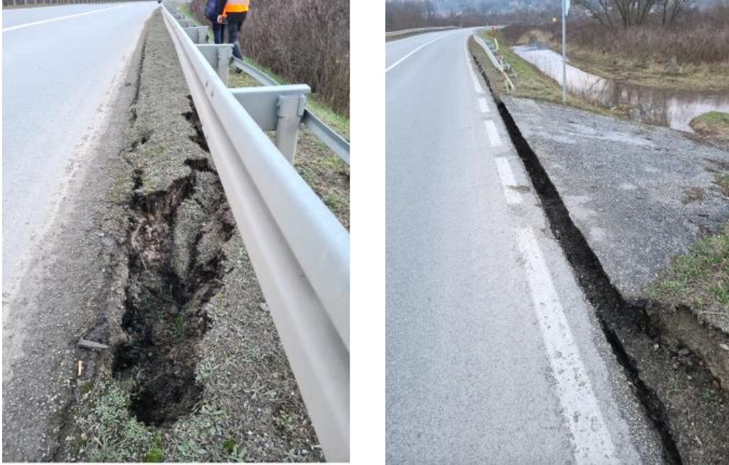
Figure 5.18. Partial ground slide due to reduced ground bearing capacity in the road close to Brest Bridge (source: Nenad Bijelić).
