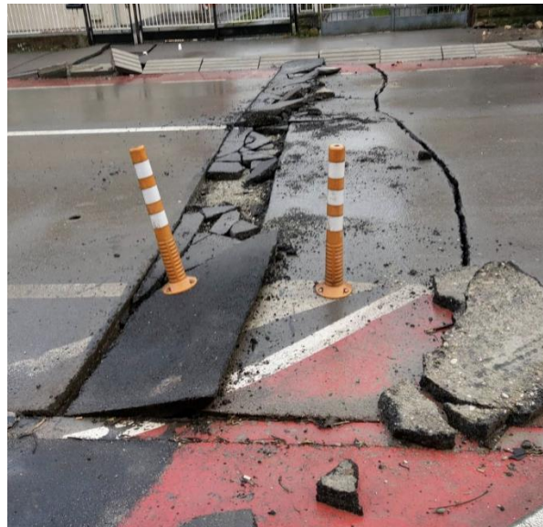
Figure 6.23. Road pavement cracking (45°29'45.108"N,16°22'36.888"E, source Zeljko Arbanas).
