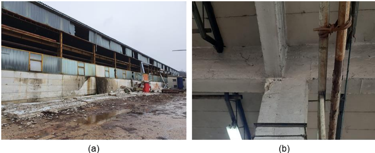
Figure 4.108. Damage to exterior cladding and concrete columns in an industrial facility in Sisačka ul. 116, 44250, Petrinja (source: Marko Bartolac).
