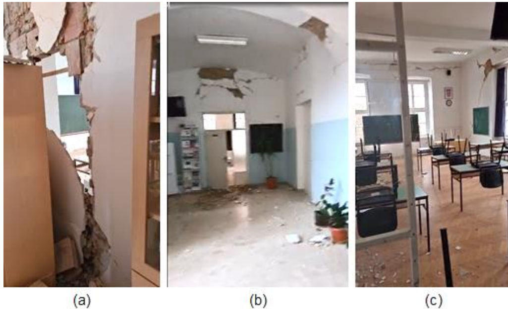
Figure 4.48. Interior damage to the First Primary School in Petrinja: (a) partial collapse of an interior partition wall showing its hollow clay tile construction, (b) damage to the interior walls, and (c) shear crack propagating from the corner of the window opening, highlighting the brittle nature of the construction (source: Nenad Bijelić).
