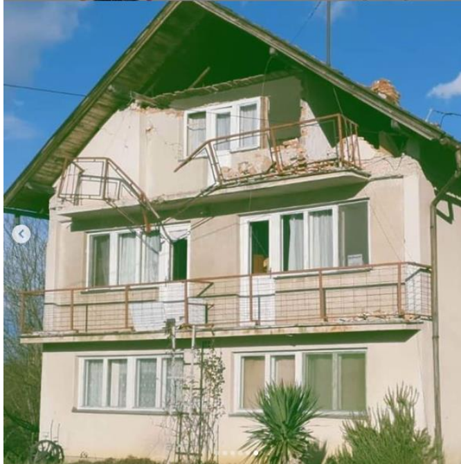
Figure 4.117. Damaged balcony guardrail in a family house in Sisak due to collapse of the gable end wall above (source: Instagram account on_a_binge_art).
