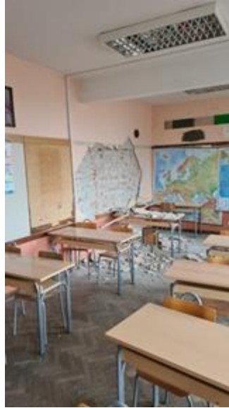
Figure 4.55. Plaster fell off of the wall exposing masonry infill (source: Nenad Bijelić and Damir Lazarević).
