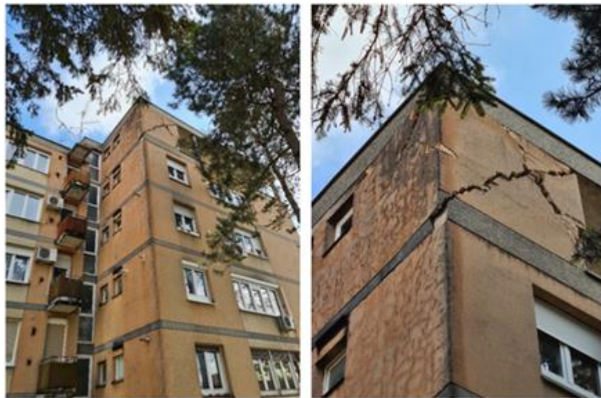
Figure 4.20. Extensive cracking experienced at the roof/terrace level of Building 2 (source: Nenad Bijelić).
