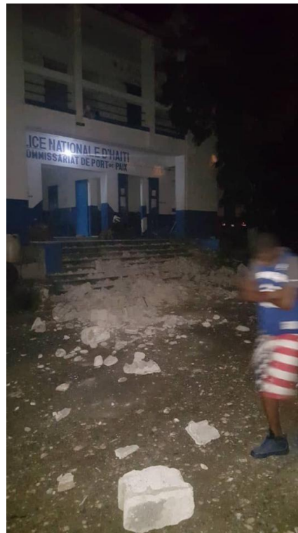
Figure 8: The damaged police station after the 2018 Haiti Earthquake
