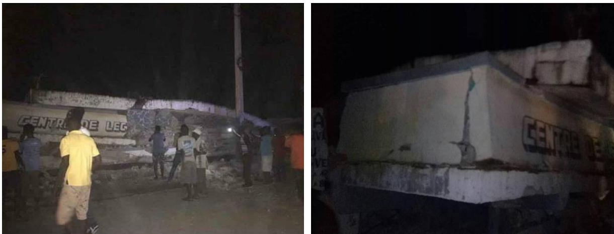
Figure 6: The collapsed auditorium after the 2018 Haiti Earthquake
