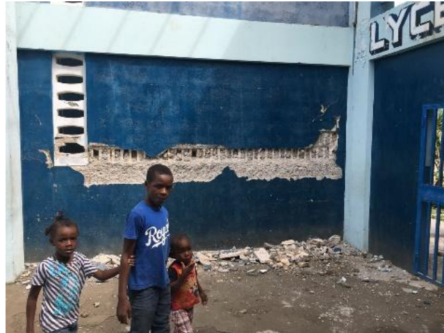
Figure 13. Damaged infill wall of the Lycee Jacques Roumain Educational Center in Gros-Morne after the 2018 Haiti Earthquake
