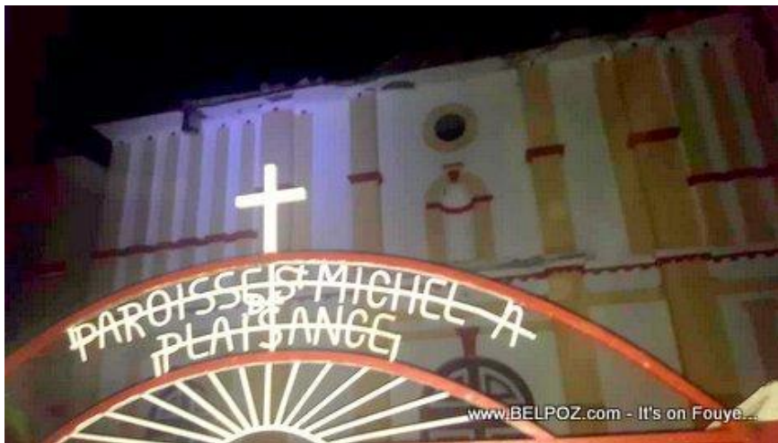
Figure 11: Damaged Paroisse Saint Michel Archange de Plaisance church after the 2018 Haiti Earthquake, note the decorative gable atop the front face in Figures 8 and 9 detached in the earthquake.
