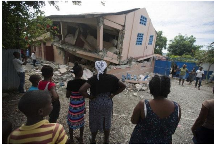
Collapsed School Building in Gros-Morne, Haiti
