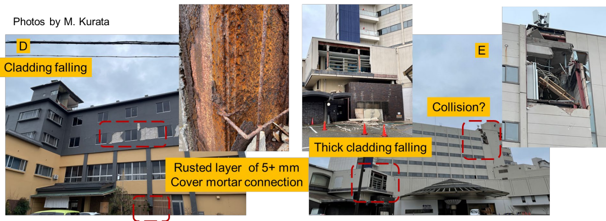
Figure 4.8. Damage to mid-rise steel buildings (Credit: M. Kurata).
