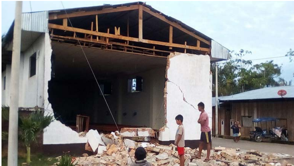
Figure 9.57. Out-of-plane collapse of a masonry wall at a church in Santa Cruz, Alto Amazonas province, in the Loreto region (Source: Rotafono [2]).
