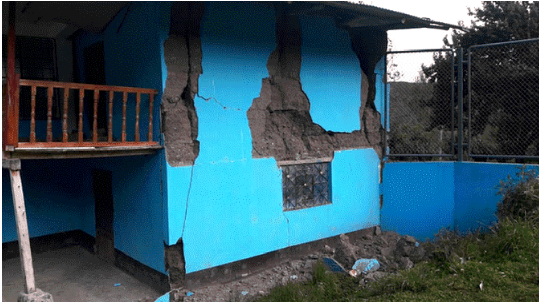
Figure 9.67. Damage in an two-story adobe school building in Cascapuy, Perú (Source: Diario La República [4]).
