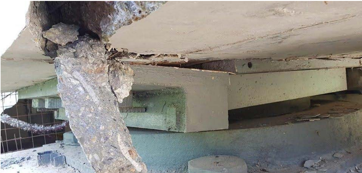
Figure 9.71. Concrete spalling near one of the supports of the bridge that crosses the Zamora river in Zamora Chinchipe province, Ecuador (Source: Bomberos El Pangui [7]).
