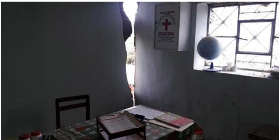
Figure 9.66. Masonry damage in junior high school building in Trujillo, Perú (Source: Diario La Industria [6]).
