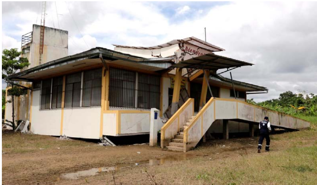
Figure 9.61. General structural damage in a healthcare facility in Huatapi, near Yurimaguas, in the Amazon region of Perú (Jourdan et al. 2019).
