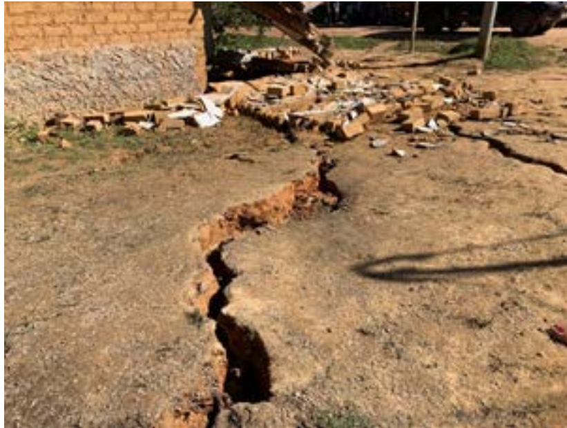
Figure 9.40. Apparent lateral spreading damage in buildings at the 2 de Mayo village, Yurimaguas. (Reategui and Mora, 2019).
