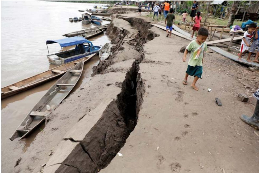
Figure 9.10. Lateral spreading along the Huallaga river at the Santa Gema near Yurimaguas in the Amazon region of Peru (Jourdan et al. 2019).
