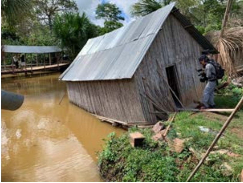
Figure 9.44. Apparent liquefaction-induced effects in buildings located at the 2 de mayo village, Yurimaguas (Reategui and Mora, 2019).
