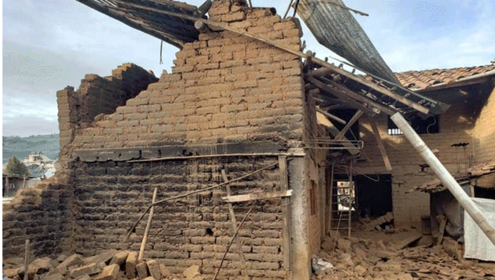
Figure 9.47. Collapse of old-housing dwelling built of adobe brick units in Huamachuco (Source: Diario La República [4]).
