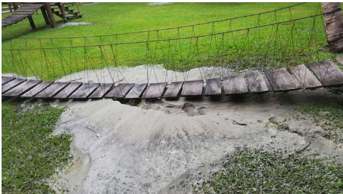
Figure 9.23. Liquefaction ejecta in El Sauce Resort, Tarapoto. (Source: Rotafono [2]).
