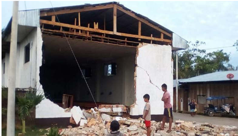
Earthquake damage in Santa Cruz, Alto Amazonas Province, Perú on May 26, 2019. (Source: Rotafono [2])
