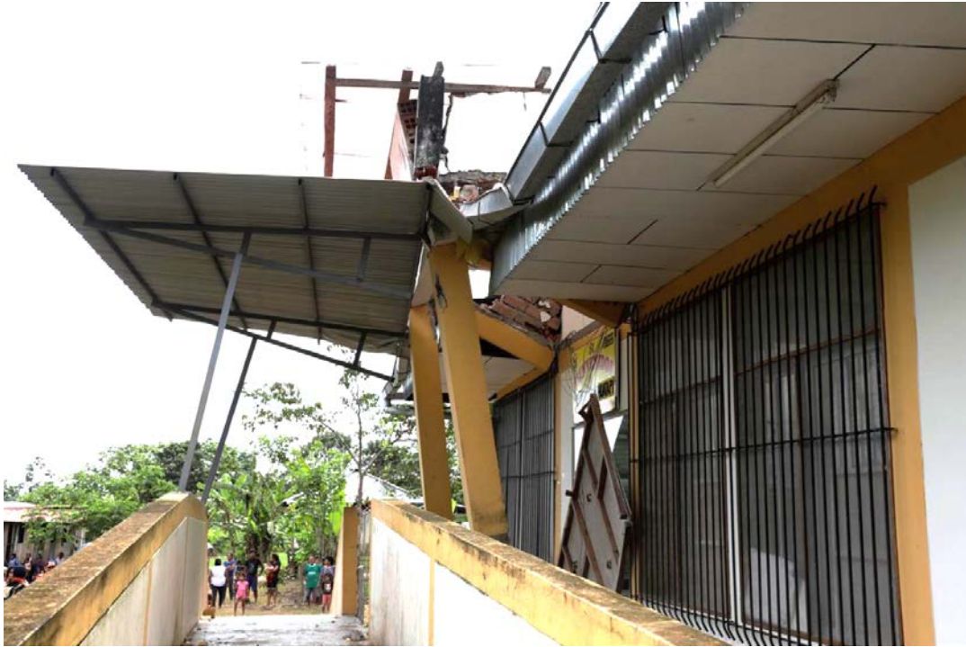
Figure 9.60. General structural damage in a healthcare facility in Huatapi, near Yurimaguas, in the Amazon region of Perú (Jourdan et al. 2019).
