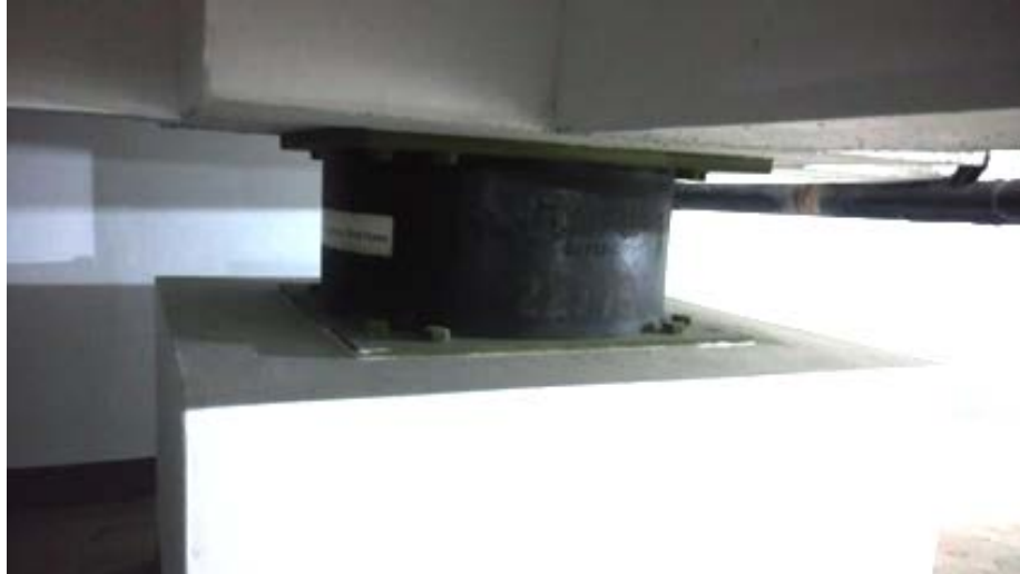
Figure 9.64. Lead-core rubber bearing base-isolator at hospital in Yurimaguas region (Courtesy of CVI Ingeniería Antisísmica).
