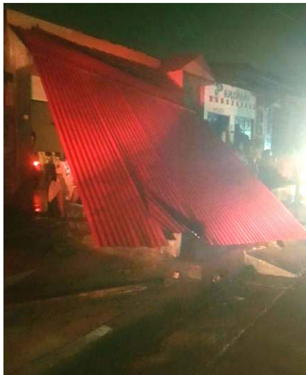
Figure 9.48. Collapsed roof structure in, Yurimaguas City, Loreto Region (Holguin, 2019 Source: Peruvian Fire-Department [7]).
