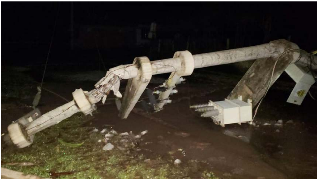
Figure 9.21. Damage to a power pole and electrical transformer caused by liquefaction at the Sauce district and Caserio 2 de Mayo in San Martin. (Source: Rotafono [2]).
