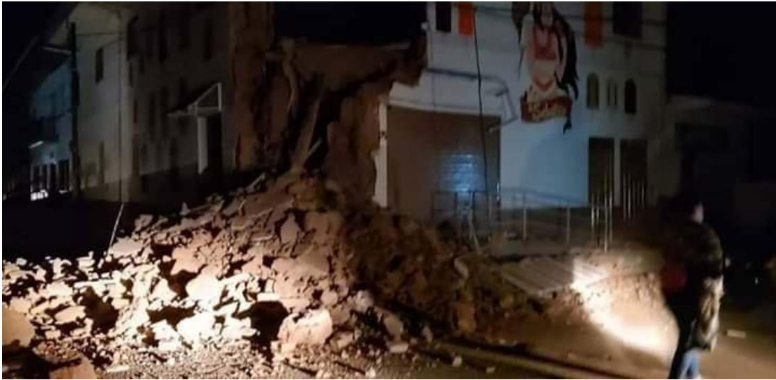
Figure 9.52. Partial collapse of the same two-story adobe building in Yurimaguas City (COEN, 2019).
