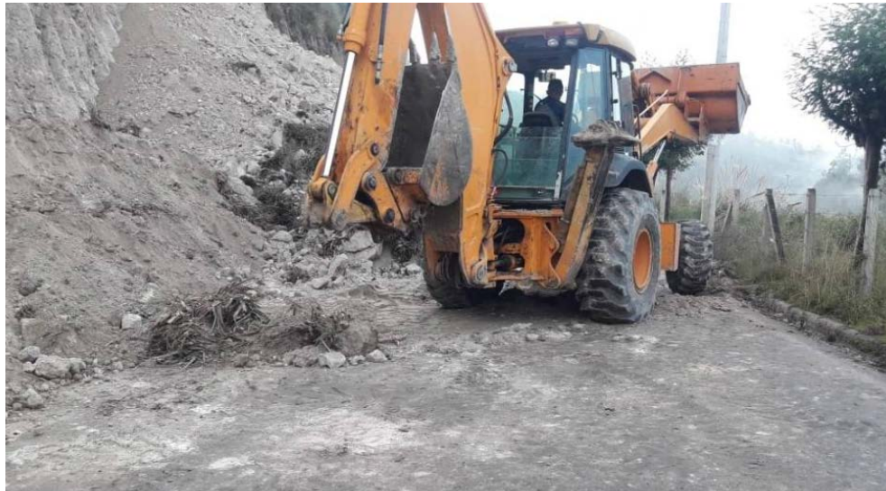
Figure 9.7. Landslide at the Gualaceo-Sigsig highway at the Province of Azuay (Source: Diario El Universo [1]).
