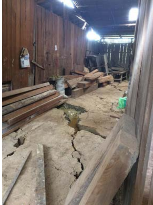
Figure 9.26. Seismically-induced ground damage due to apparent liquefaction and lateral spreading at El Sauce District (Source: Ministerio de Vivienda del Perú - Photo by Miguel Estrada).
