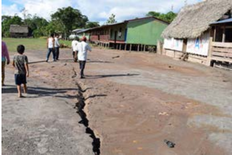
Figure 9.28. Seismically-induced ground damage due to liquefaction and lateral spreading at El Sauce District (Source: Ministerio de Vivienda del Perú - Photo by Miguel Estrada).
