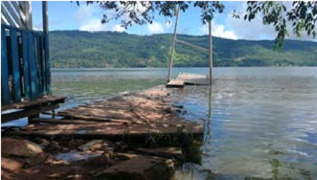
Figure 9.45. Failure of a wharf structure along the Huallaga river near Yurimaguas (Reategui and Mora, 2019).
