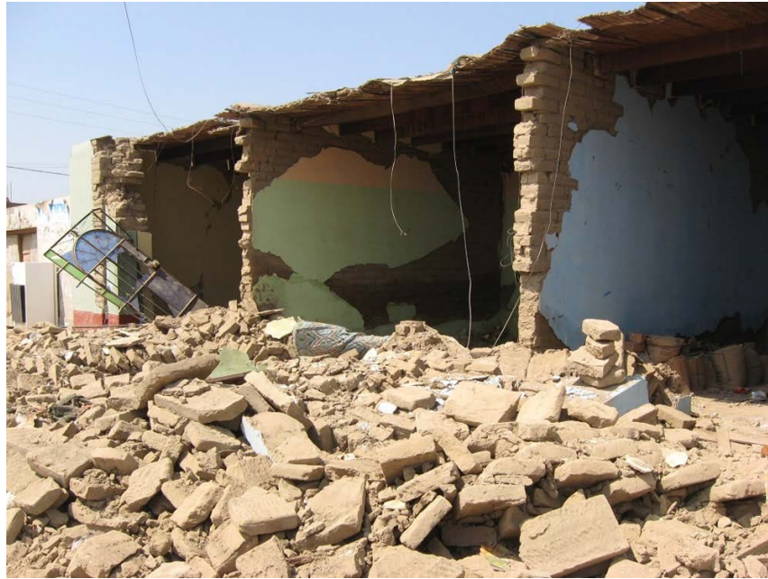
Figure 6.3. Example of collapse of non-engineered adobe construction in Perú as a result of the 2007 Pisco earthquake (Source: EERI Housing encyclopedia).
