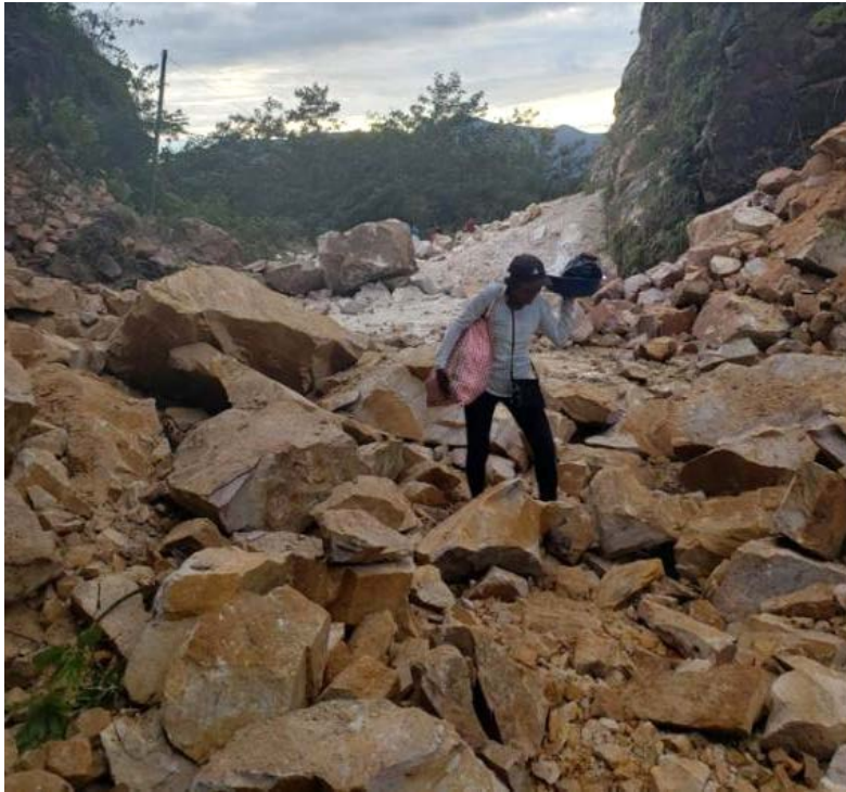
Figure 9.16. Damaged highway Tarapoto -Yurimaguas (Holguin, 2019).
