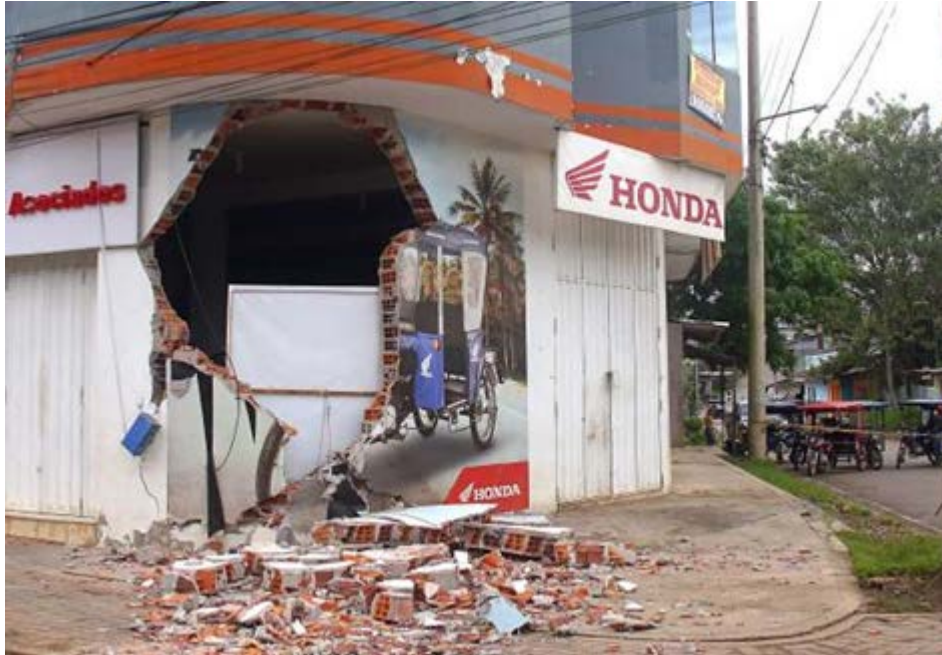
Figure 9.54. Out-of-plane failure of a masonry infill wall in a commercial building located in Yurimaguas (Source: AFP [3]).
