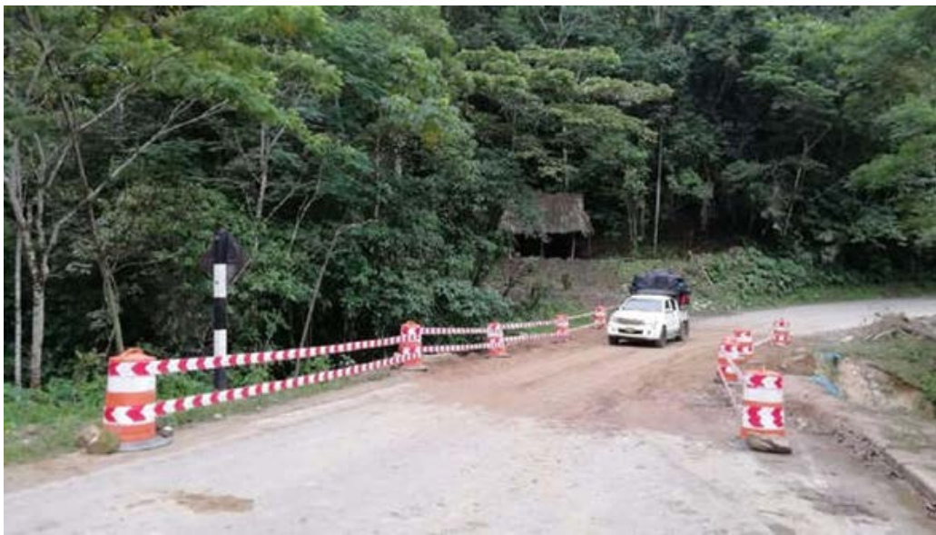
Figure 9.69. Bridge between Yurimaguas and Tarapoto (Puente Shimbillo) which suffered minor damaged after the earthquake [5].
