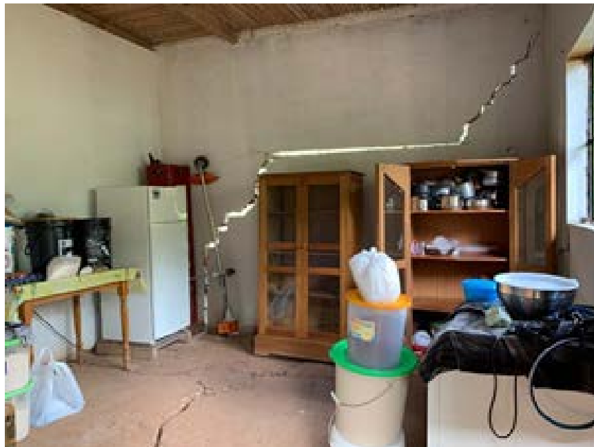
Figure 9.41. Severe damage in residential construction caused by ground deformations at the 2 de Mayo village, Yurimaguas (Reategui and Mora, 2019).
