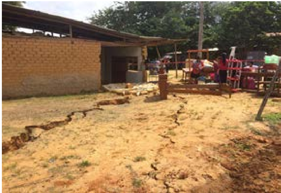
Figure 9.29. Seismically-induced ground damage at El Sauce District (Source: Ministerio de Vivienda del Perú - Photo by Miguel Estrada).
