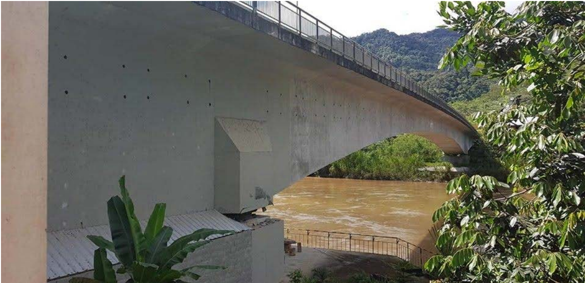
Figure 9.70. Overall view of the bridge that crosses the Zamora river in Zamora Chinchipe province, Ecuador (Source: Bomberos El Pangui [7]).
