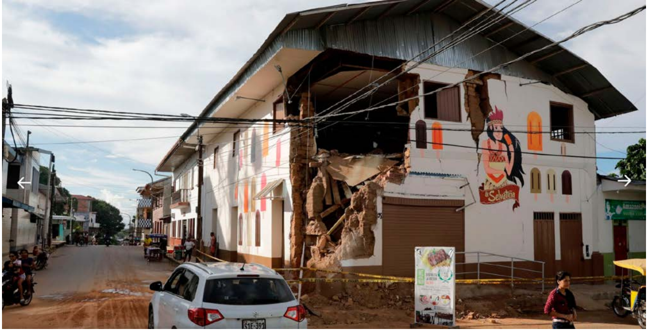
Figure 9.51. Partial collapse of a two-story adobe building in Yurimaguas, Perú (Holguin, 2019).
