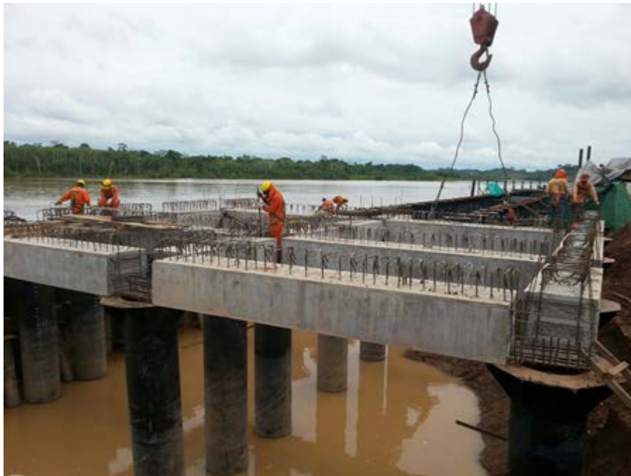
Figure 9.74. Overview of the port of Yurimaguas during construction. (Source: Postensa SAC. Dr. Luis Bozzo).
