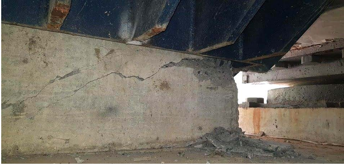
Figure 9.72. Shear cracking at the base of one of the supports of the bridge that crosses the Zamora river in Zamora Chinchipe province, Ecuador (Source: Bomberos El Panguí [7]).
