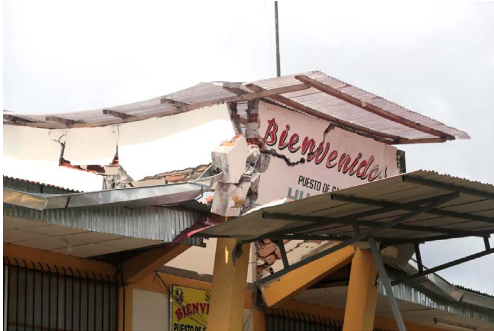
Figure 9.62. General structural damage in a healthcare facility in Huatapi, near Yurimaguas, in the Amazon region of Perú (Jourdan et al. 2019).
