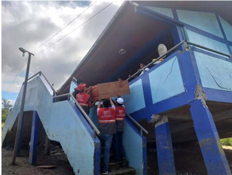
Figure 9.65. Structural damage in upper first story columns in a school building in La Esperanza, Perú (Source: Diario La Industria [6]).
