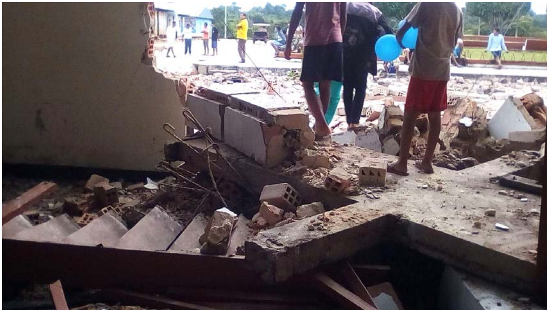
Figure 9.58. Out-of-plane collapse of a masonry wall at a church in Santa Cruz, Alto Amazonas province, in the Loreto region (Source: Rotafono [2]).
