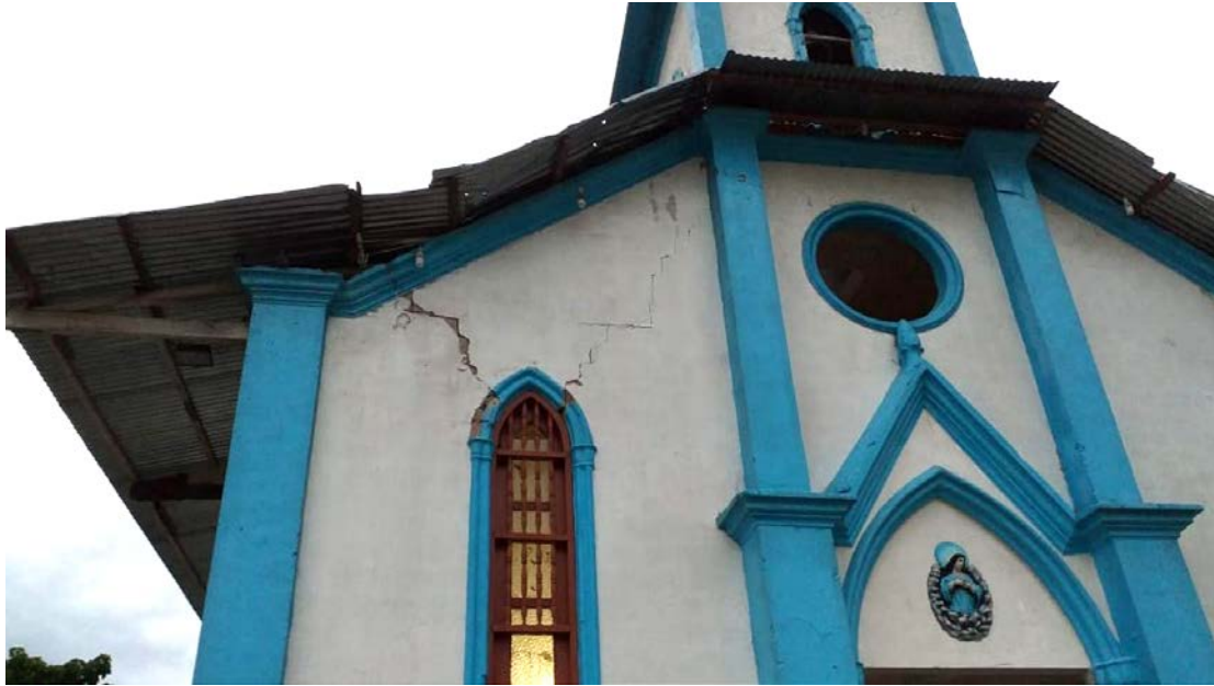
Figure 9.59. Diagonal cracking in the facade of a church after the earthquake at Alto Amazonas province, in the Loreto region (Source: Rotafono [2]).
