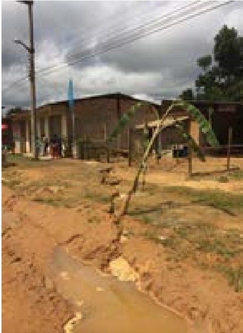
Figure 9.31. Seismically-induced ground damage due to apparent liquefaction and lateral spreading at El Sauce District (Source: Ministerio de Vivienda del Perú - Photo by Miguel Estrada).
