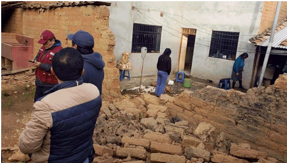
Figure 9.46. Collapse of old-housing dwelling built of adobe brick units in Huamachuco (Source: Diario La República [4]).
