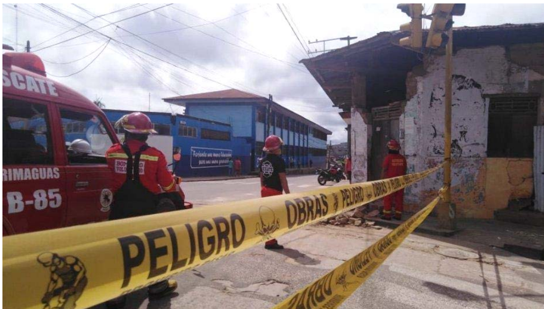
Figure 9.50. Damaged to adobe building in Alto Amazonas, Loreto (Holguin, 2019).
