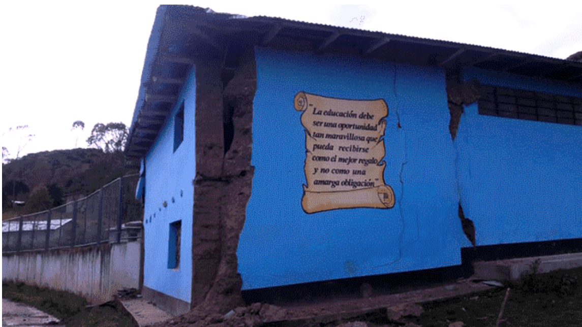
Figure 9.68. Damage in an adobe school building in Cascapuy, Perú (Source: Diario La República [4]).
