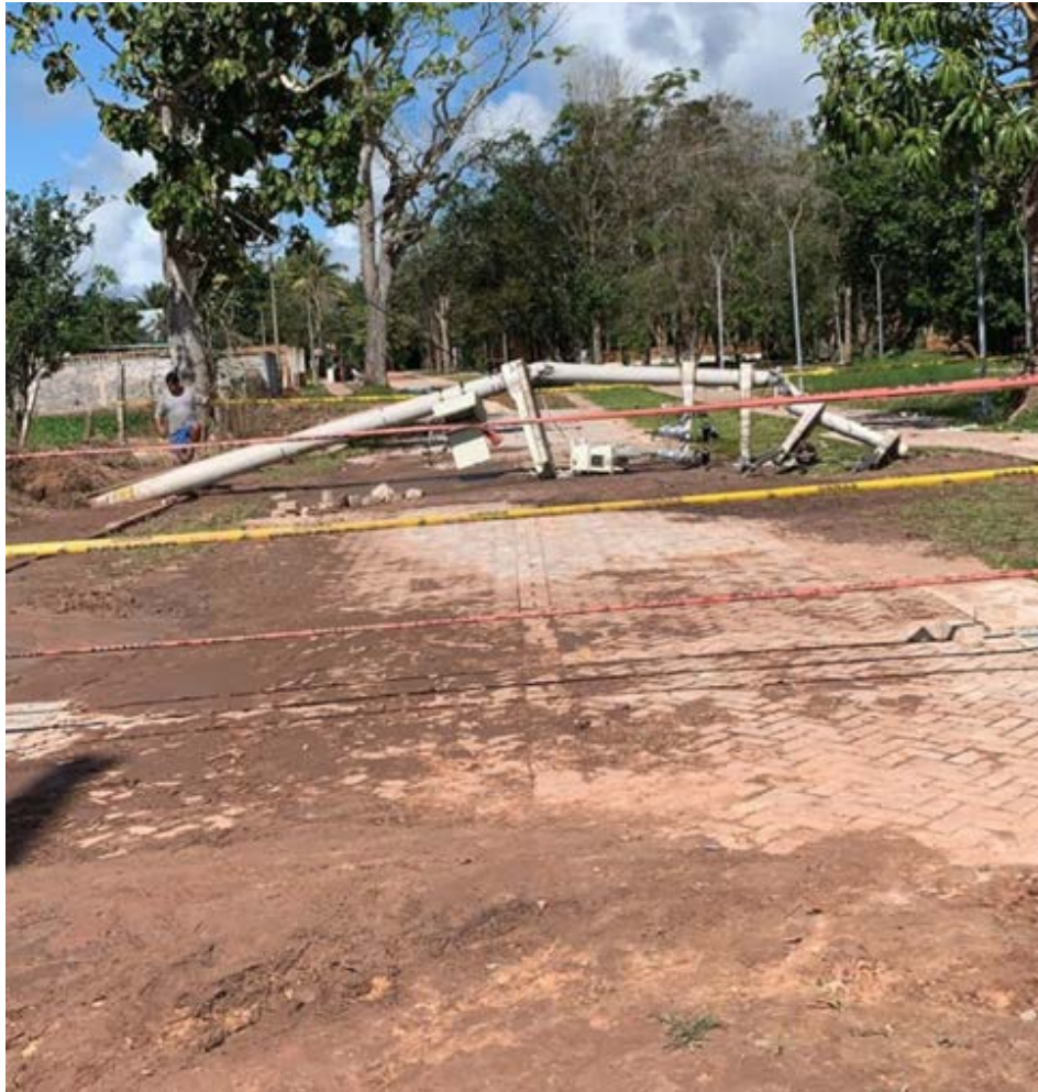
Figure 9.22. Collapse of a power pole and electrical transformer caused by liquefaction-induced failure of its footing foundation at the Sauce district and Caserio 2 de Mayo in San Martin. (Source: Rotafono [2]).
