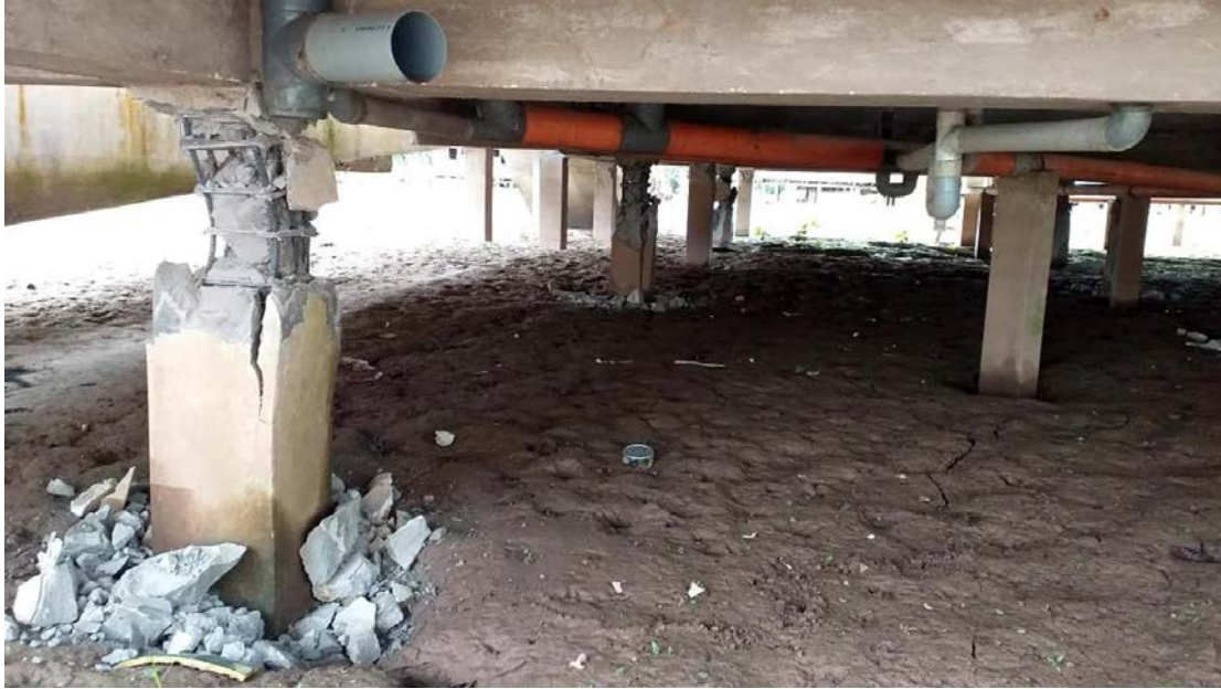
Figure 9.53. Shear failure in short foundation columns of a reinforced concrete building (Source: Rotafono [2]).
