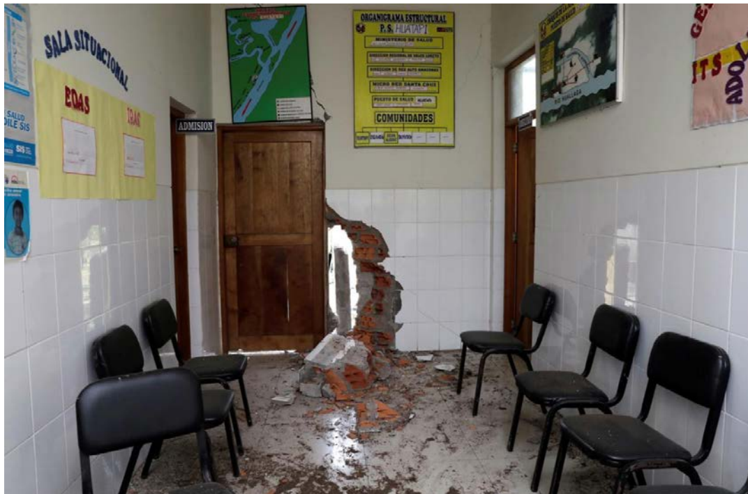
Figure 9.77. Severe damage in a masonry wall in a healthcare facility near Yurimaguas in the Amazon region of Peru (Jourdan et al. 2019).
