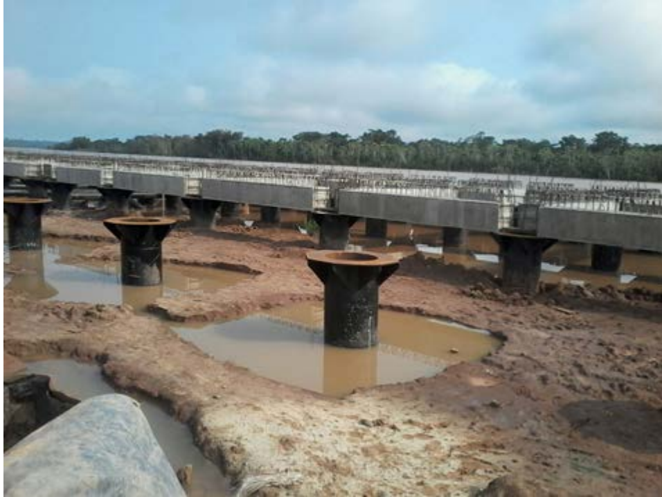
Figure 9.75. Overview of the port of Yurimaguas during construction (Source: Postensa SAC. Dr. Luis Bozzo).
