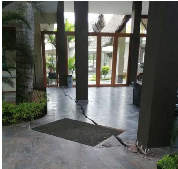
Figure 9.25. Failure of the slab-on-grade at El Sauce Resort, Tarapoto (Source: Rotafono [2]).
