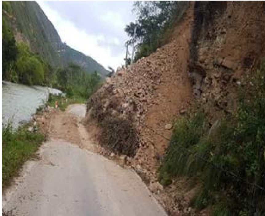
Figure 9.36. Landslides at the Leymebamba-Chachapoyas road, Ubillon sector, km 272+00, Amazonas (COEN, 2019).
