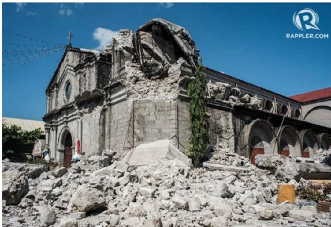
Figure 5. Collapsed stone bell tower of the 19th-century Santa Catalina de Alejandria Church
