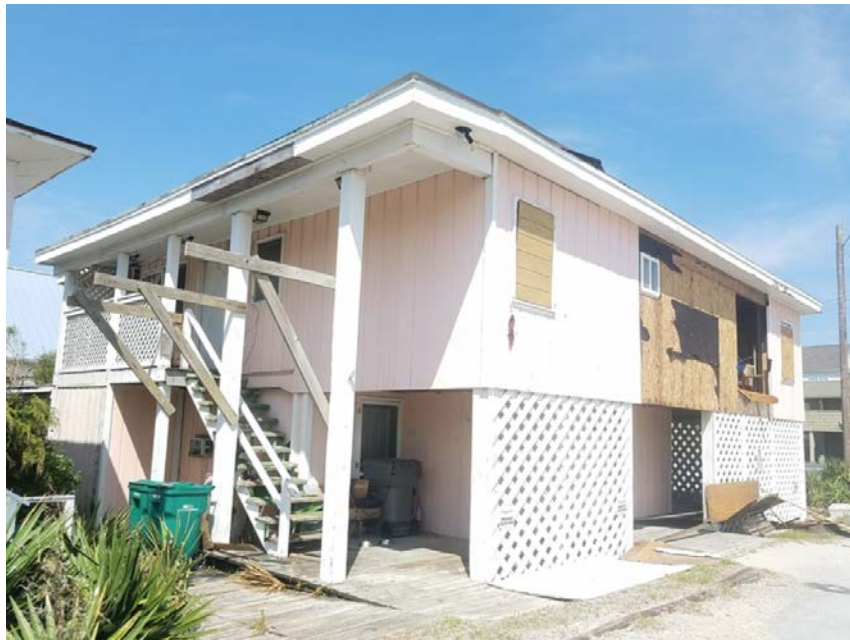
Figure 11: Loss of wood panel siding in Surf City
