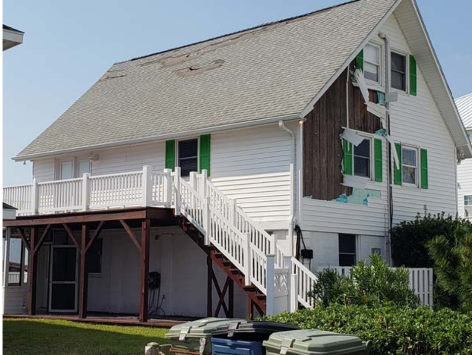
Figure 9: Loss vinyl siding installed over wood panel siding and shingle loss near roof ridge in Emerald Isle
