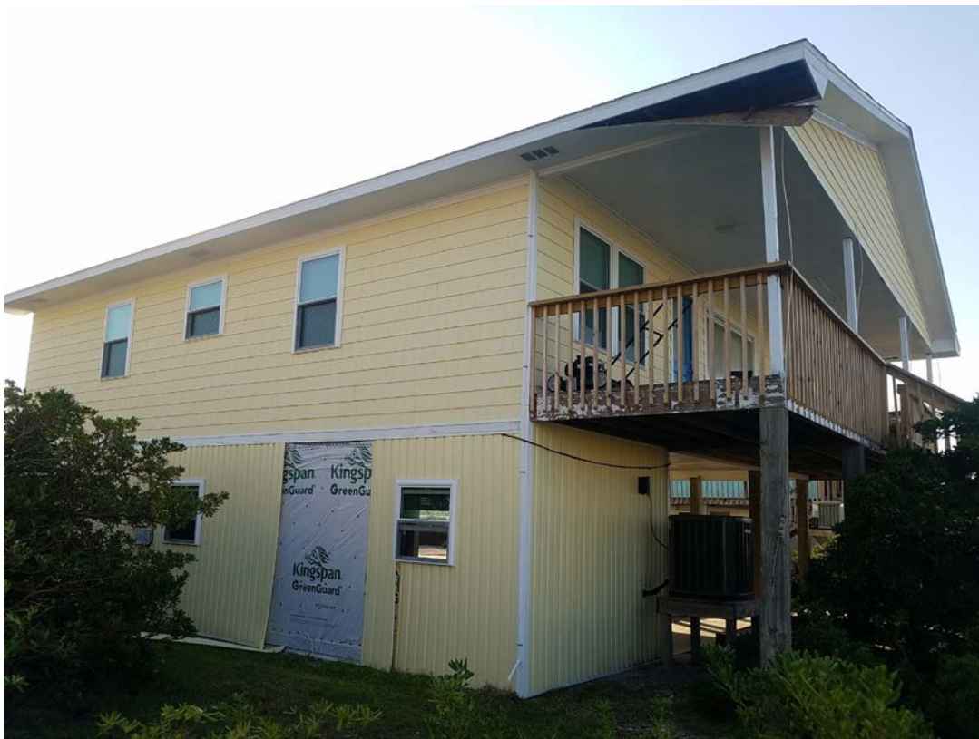
Figure 12: Damaged residence in Topsail Beach with siding loss and soffit damage
