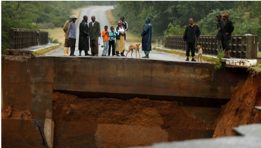
Figure 7: Abutment to bridge span crossing the Umvumvu river washed away following Cyclone Idai in Chimanimani (Photo Credit: Reuters)
