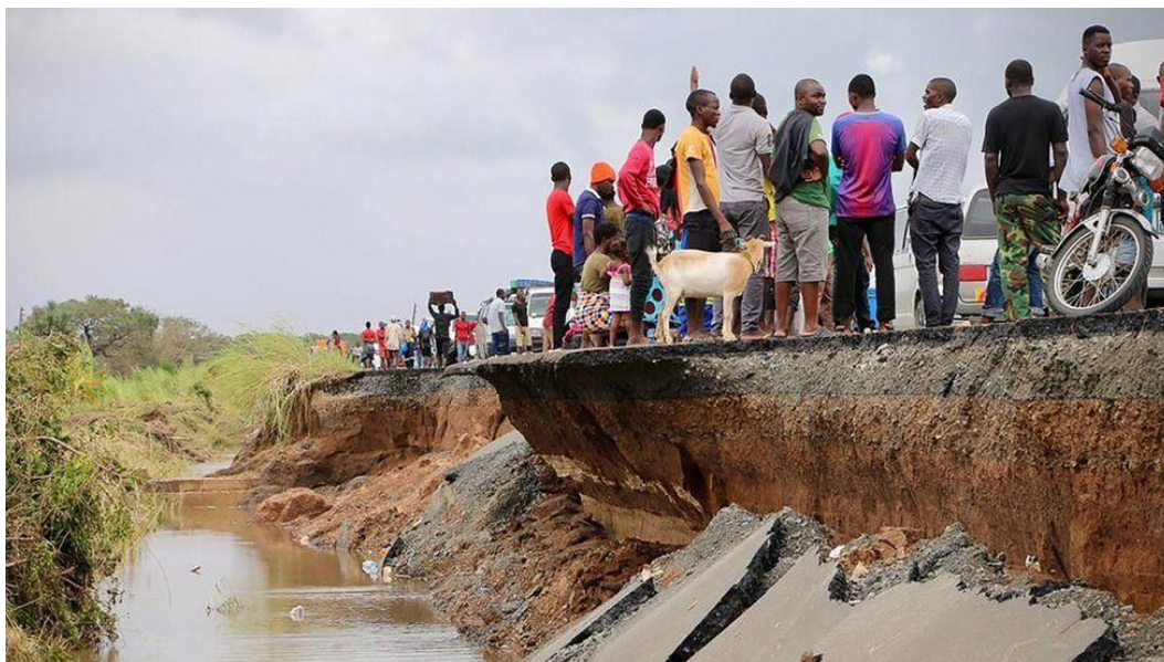
Figure 8: Damaged section of the road between Beira and Chimoio in Nhamatanda District in Central Mozambique after the area was hit by Cyclone Idai.
