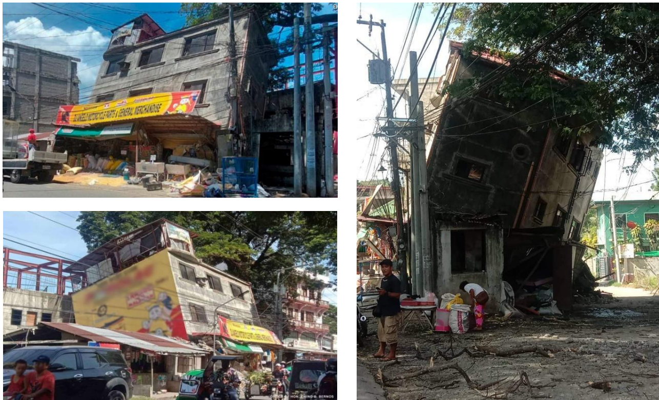
Figure 5. Collapsed soft/weak story building (CNN, 2022; CNNPhilippines, 2022; Twitter, 2022a).
