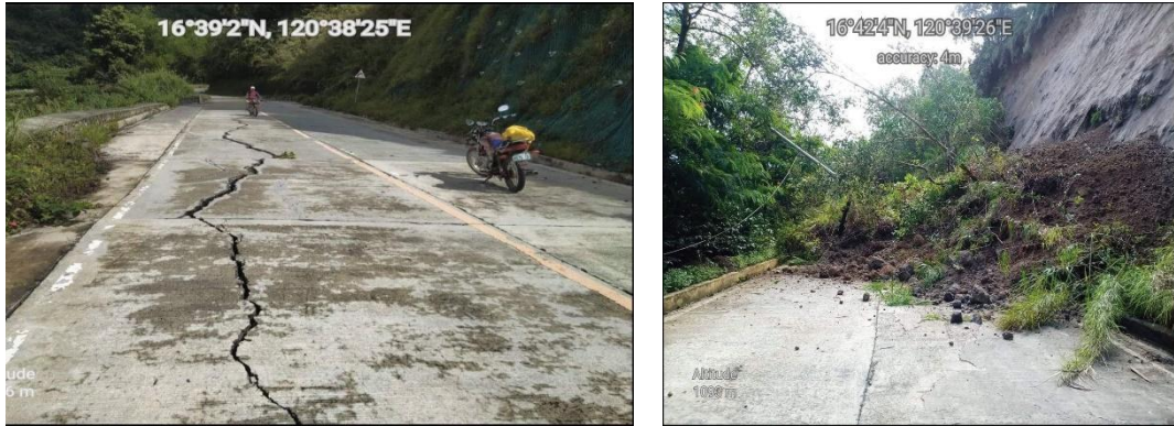
Figure 9. Damaged roads due to ground shaking and blocked by landslides (GMA News, 2022).
