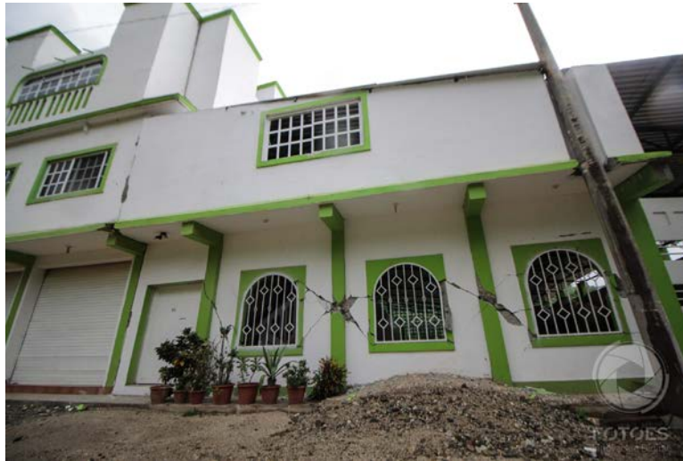
Figure 7.10. Masonry wall facade damage in a multi-family building. Damage is heavily concentrated in the first story (Diario Marca, 2020b).
