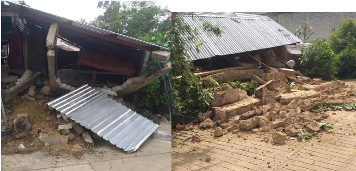
Figure 7.1. Out-of-plane collapsed walls in single family buildings. Left, Ozolotepec municipality in Oaxaca (Twitter, 2020c), and right, Santa Catarina Xanaguía, San Juan Ozolotepec, Oaxaca (Twitter, 2020d).
