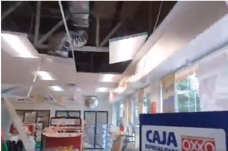
Figure 7.29. Non-structural damage in a store in Oaxaca (Twitter, 2020m).
