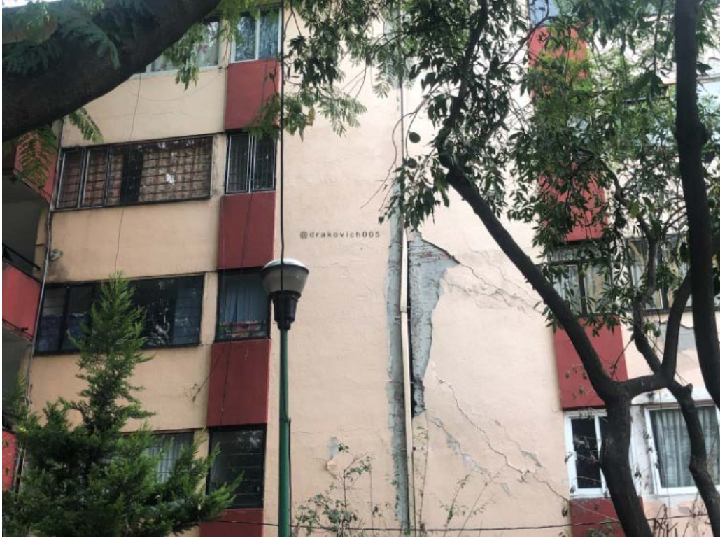
Figure 8.2. Apartment building tilted at Unidad Habitacional Lindavista-Vallejo in Mexico City.
