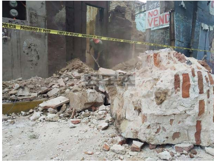
Figure 7.7. Masonry debris after single family building collapse in Oaxaca City (Daily Mail, 2020).
