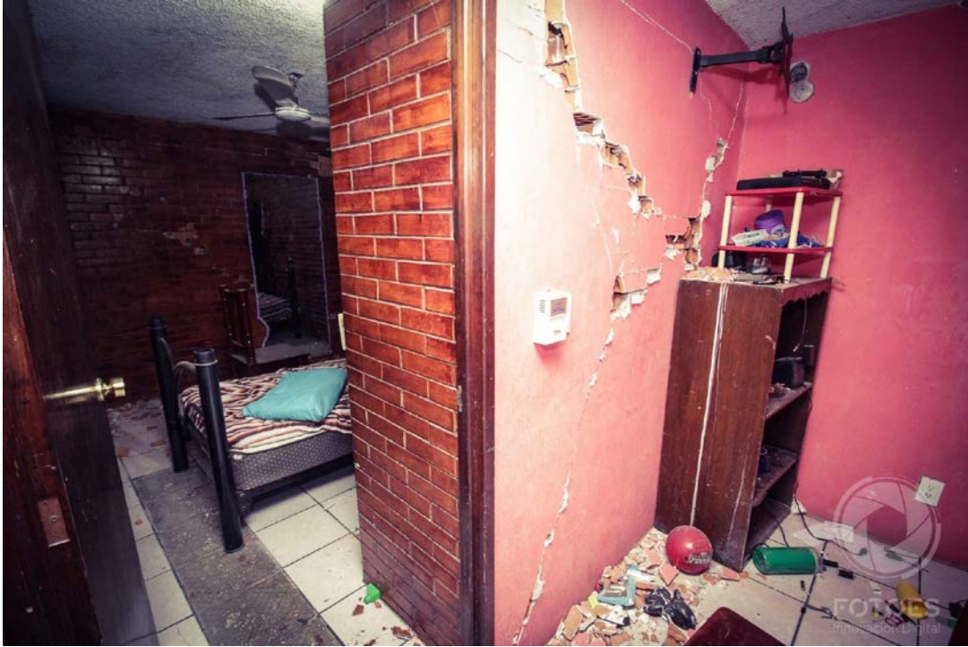
Figure 7.9. Diagonal cracking in the first story of an unreinforced masonry residence (Diario Marca, 2020a).
