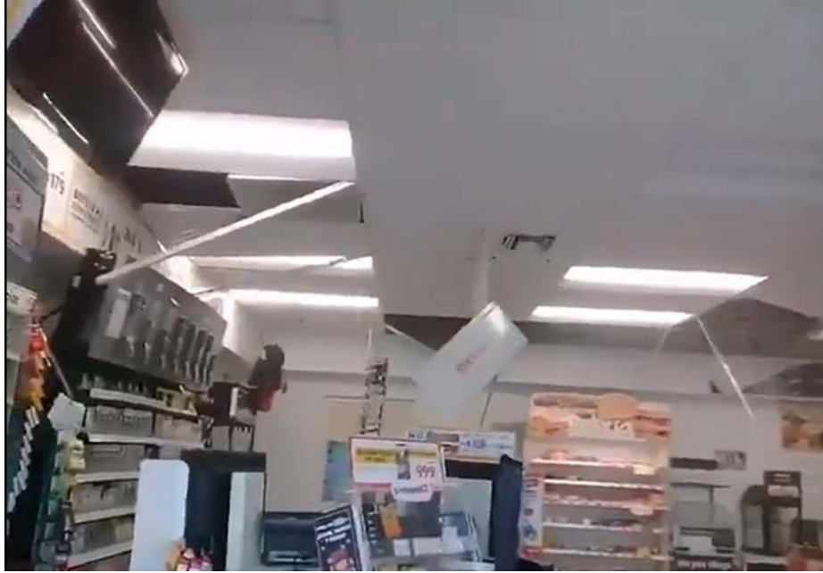
Figure 7.30. Non-structural damage in a store in Oaxaca (Twitter, 2020m).
