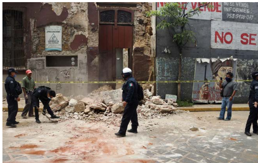
Figure 7.13. Failure of adobe walls in single-story buildings in Oaxaca. (New York Post, 2020).
