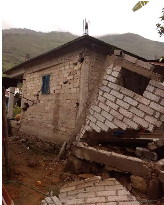
Figure 7.2. Top: Out-of-plane collapse of a boundary wall in an adobe residential construction, Oaxaca (Twitter, 2020e); Bottom: collapse of a confined masonry wall in a residential building, Santa Cruz Ozolotepec (Facebook, 2020a).
