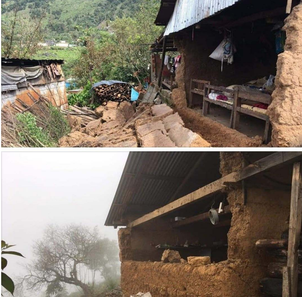
Figure 7.3. Out-of-plane collapse of the upper portion of a wall in an adobe residential construction, Oaxaca (Twitter, 2020f).
