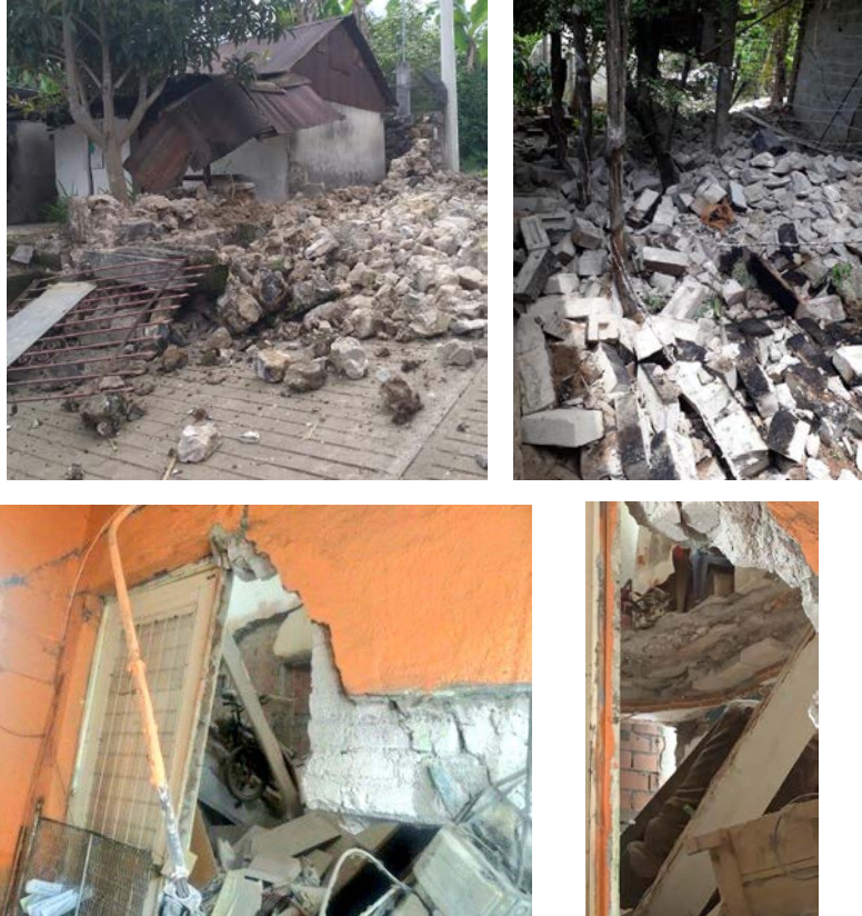
Figure 7.6. Examples of unreinforced masonry building collapse Top left: San Juan Ozolotepect (Zona Roja, 2020) and Top right: San Miguel del Puerto (Twitter, 2020h) Bottom: Bolivar Colonia Obrera in Cuauhtémoc (Integral Risk Management Secretariat via Twitter, 2020t).
