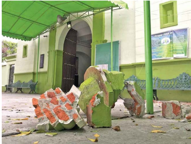
Figure 7.25. Collapse of parapet ornamentation in the church of Santísima Trinidad de las Huertas, City of Oaxaca. (Excelsior, 2020b).
