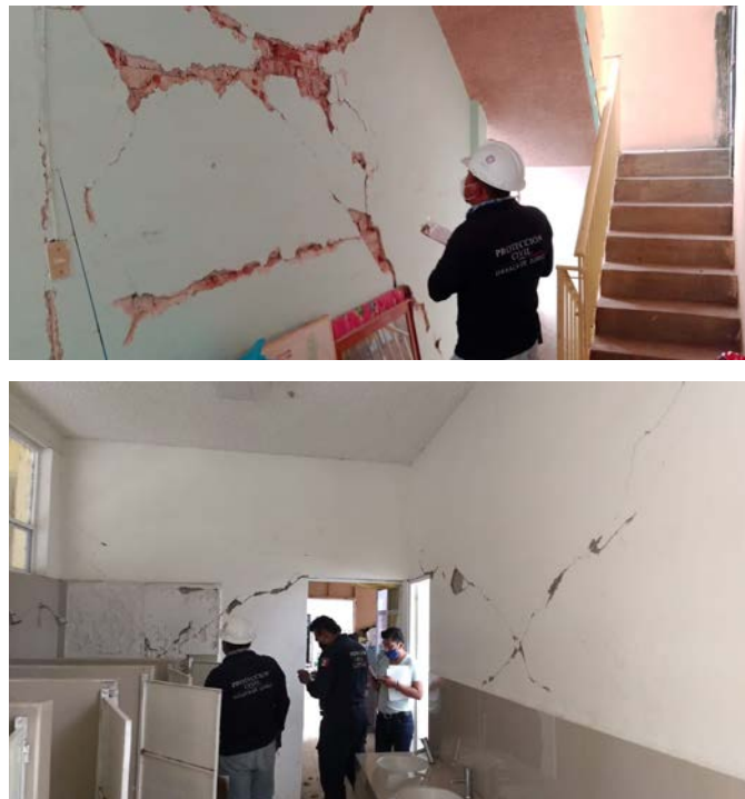
Figure 7.11. Damage inspections by Civil Protection personnel in Oaxaca (Twitter, 2020j).
