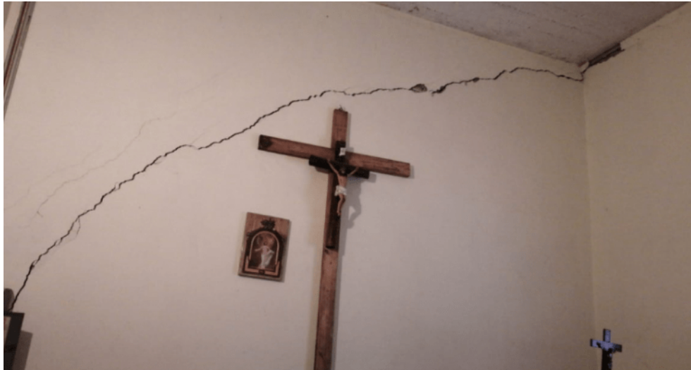
Figure 8.5. Cracks in interior walls at a religious building in Mexico City. (Espinosa, 2020a).
