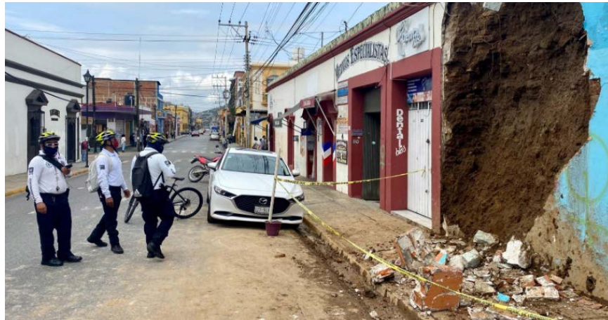
Figure 7.12. Failure of adobe walls in single-story commercial building (Animal Politico, 2020).
