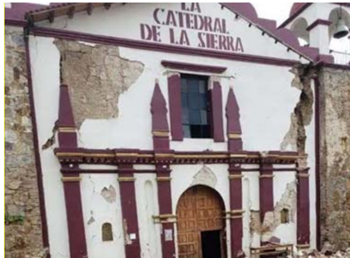
Figure 7.23. Damage to the La Catedral de la Sierra church at San Juan Ozolotepec, Oaxaca (Excelsior, 2020a).
