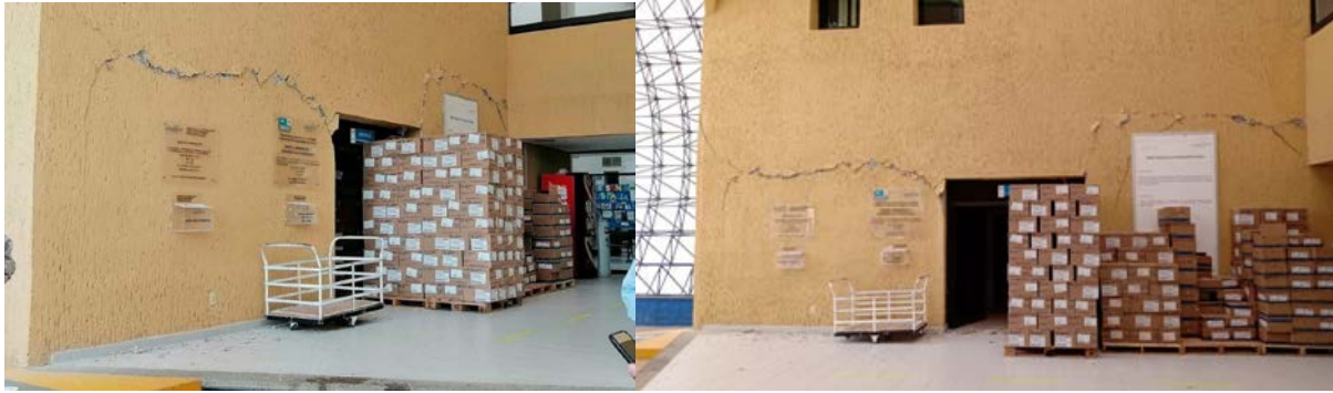
Figure 7.19. Damage to the regional Speciality hospital of Oaxaca located at San Bartolo Coyotepec, Oaxaca (Facebook, 2020b).
