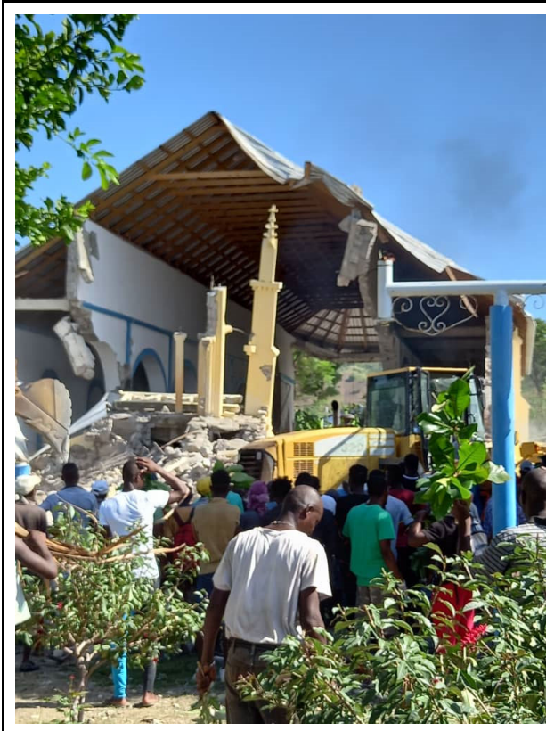
Partial collapse of the church of the Immaculate Conception in Les Anglais (Source: teleSUR )
