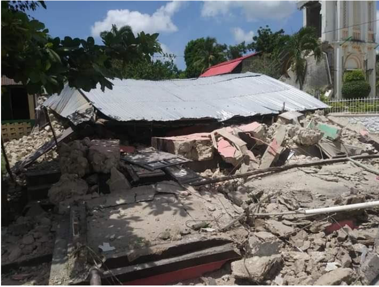
Collapsed house in the commune of Maniche, Les Cayes, Sud Department (Source: Twitter )
