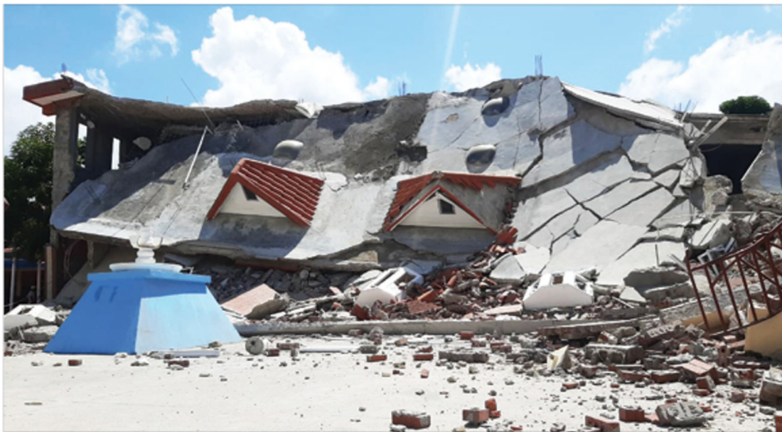
Figure 4.14. Completely collapsed Market Immaculée in Camp-Perrin, Les Cayes, Sud Department, a mixed use structure (grocery, hotel, and restaurant) (Sources: Twitter , Newspaper Le Nouvelliste ).
