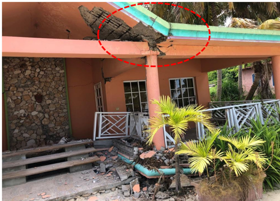
Figure 4.2. Example of damaged slab and beam-column connection in Abaka Bay Resort hotel, on the beachfront in Jeremie in Grand'Anse Department of Haiti. (Source: Jesus Chris' Twitter account; Journalist and broadcaster).
