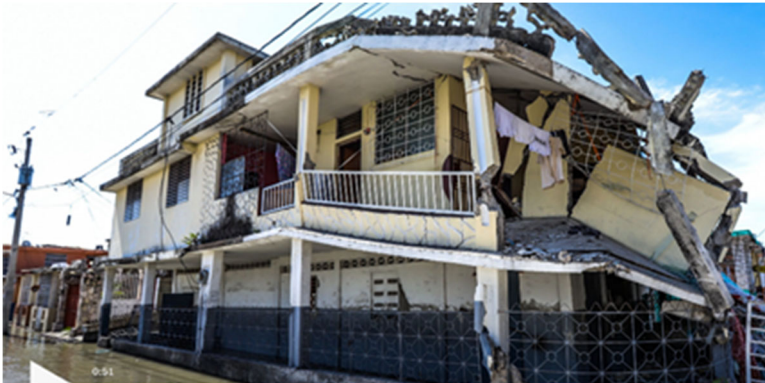
Partial collapse of a multi-family RC residential building (Still photo of a footage by Ralph Tedy Erol/AP, Source: NY Times )
