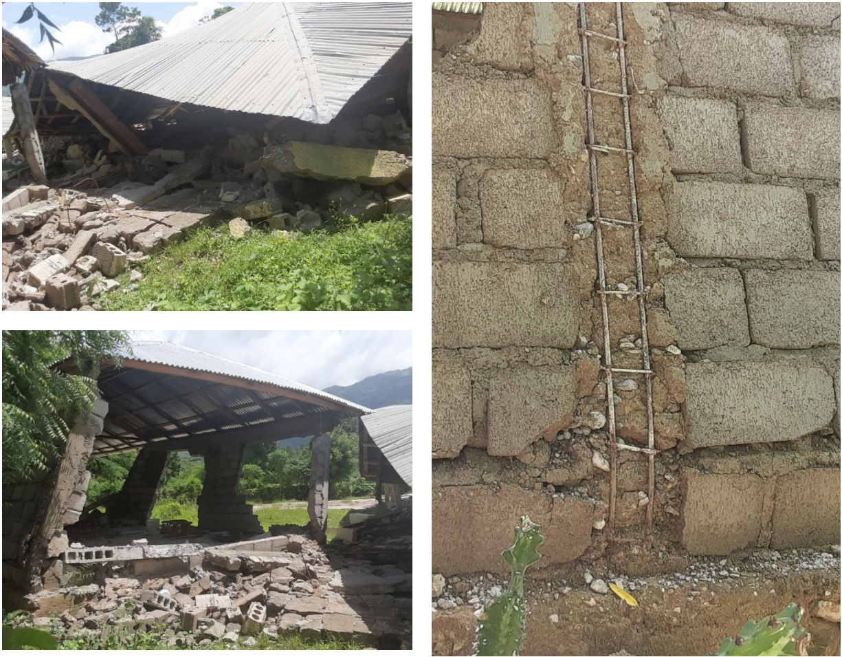
Figure 4.22. Collapse of weakly confined masonry school in L'Asile, Nippes Department (Source: Gefthe Devilme, GeoHazards International).
