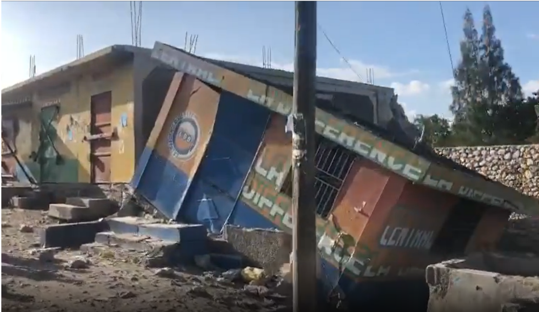
Figure 6.4. Foundation failure under small business in Saint George area in southwest Haiti (Source: Twitter ).
