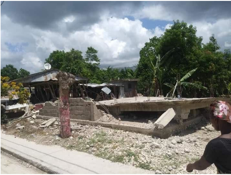
Collapse of masonry building in the commune of Maniche, Cayes, Sud Department (Source: Twitter )
