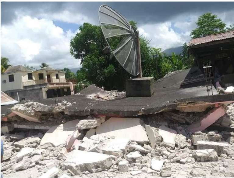
Collapse of masonry building in the commune of Maniche, Cayes, Sud Department (Source: Twitter )
