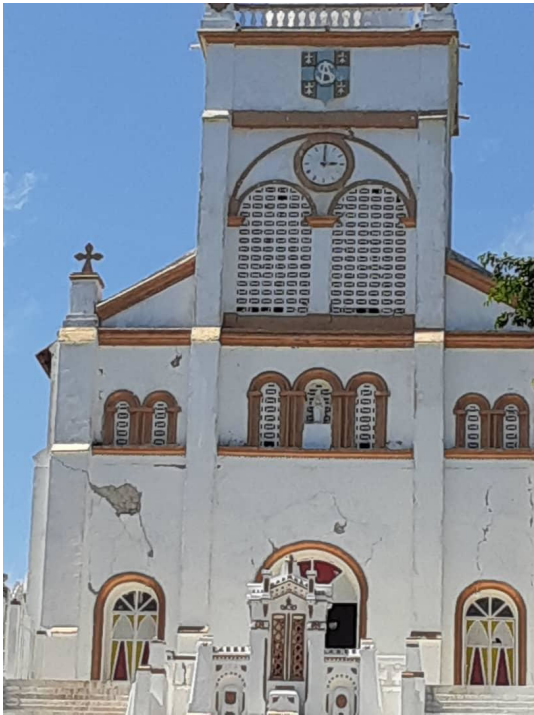
Damage to the cathedral of Saint Anne in the commune of Anse-à-Veau (Source: GeoHazards International).
