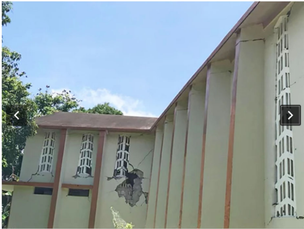
Damage to the church of Saint Anne, in La Sucrerie Henry, commune of Aquin, Sud Department (Source: Mona Lisa Lives Here )
