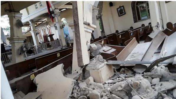
Damage to the church of Saint Joseph in the commune of L'Asile (Source: Boston Pilot )
