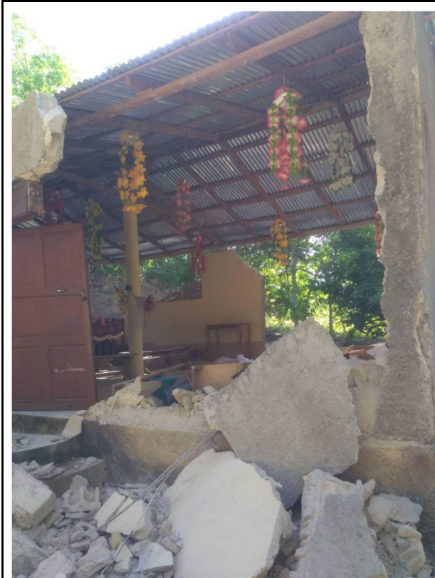
Collapse of the Shekinah Free Methodist Worship Center in Corail (Source: New Haven Register )
