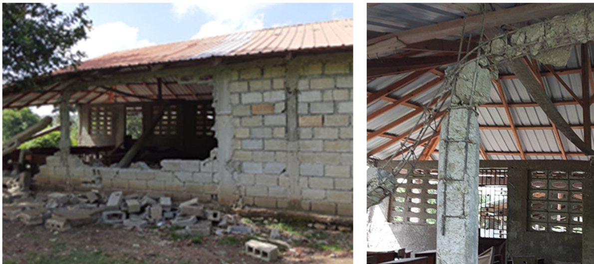
Figure 4.21. Severe damage of school in Baltazar (Source: Gefthe Devilmé, GeoHazards International).
