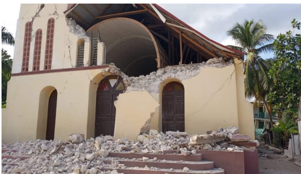
Partial collapse of the parish church in the commune of Corail, Grand d'Anse Department (Source: Twitter )
