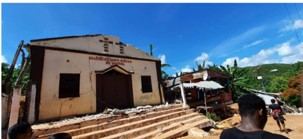
Partial collapse of the Baptist MEBSH church of Pestel (Source: Twitter )
