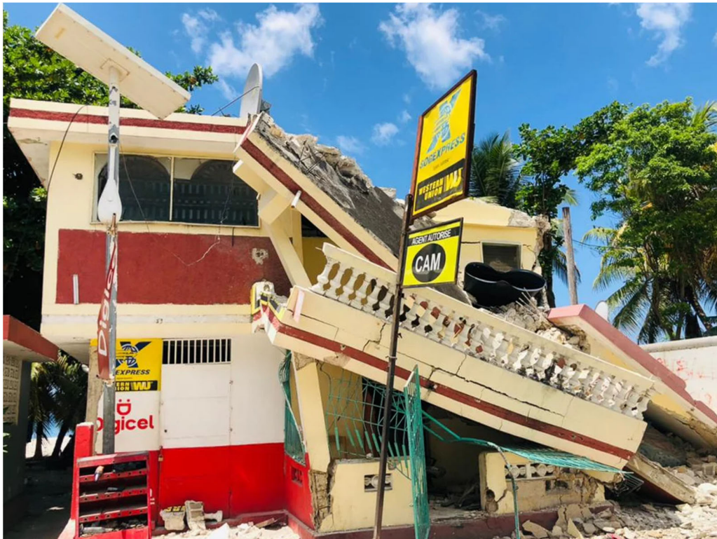
Figure 4.13. Collapse of small business in Petite-Rivière-de-Nippes (Source: npr ).
