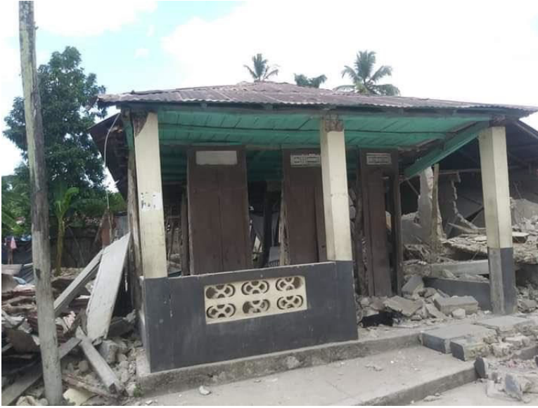
Damage to infill walls in homes in the commune of Maniche, Cayes, Sud Department (Source: Twitter )
