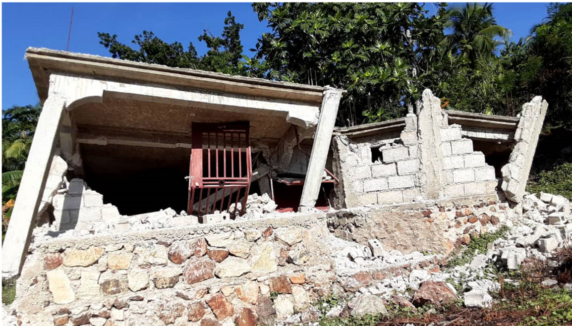
Figure 4.6. Damage of a single-story home in Anse-a-Veau (Credit: Gefthé Dévilme, GeoHazards International).
