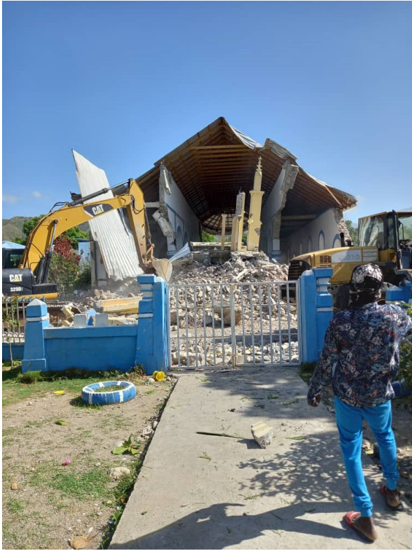
Partial collapse of the church of the Immaculate Conception in Les Anglais (Source: teleSUR )
