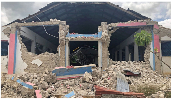
Damage to the church of the Sainte Famille du Toirac, in Toirac, commune of Camp Pérrin (Source: Boston Pilot )
