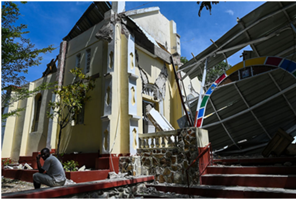
Damage to the church of Saint Joseph in the commune of L'Asile (Source: Washington Post )
