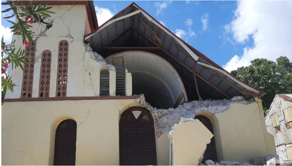
Partial collapse of the parish church in the commune of Corail, Grand'Anse Department (Source: Milícia da Imaculada )
