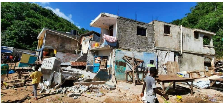
Damaged houses in the commune of Pestel, Corail Arrondissement, Grand'Anse Department (Source: Twitter )
