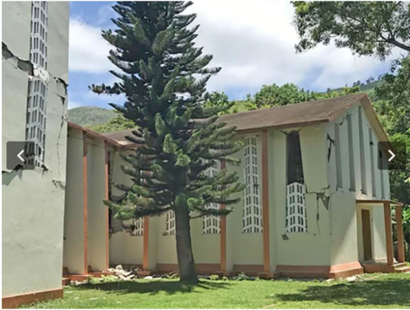
Damage to the church of Saint Anne, in La Sucrerie Henry, commune of Aquin, Sud Department (Source: Mona Lisa Lives Here )
