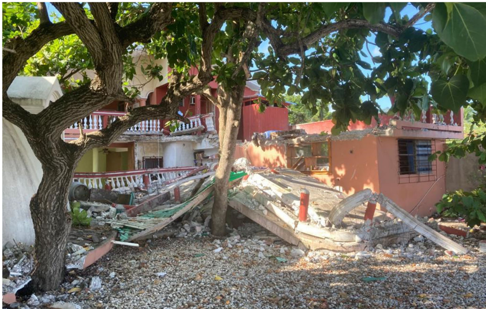
Figure 4.11. Collapsed Manolo Inn Hotel in Petite Riviere de Nippes (Credit: Gefthé Dévilmé, GeoHazards International).
