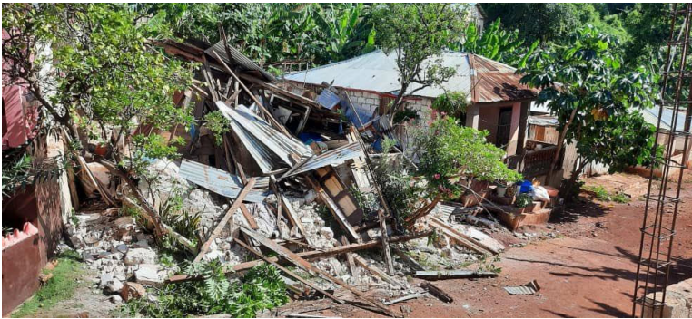
Collapsed house in the commune of Pestel, Corail Arrondissement, Grand'Anse Department (Source: Twitter )
