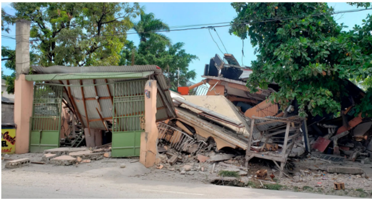
Cayimite Hotel collapse in Les Cayes, Aug. 14, 2021 (Source: US today )
