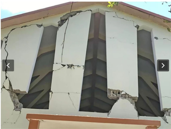
Damage to the church of Saint Anne, in La Sucrerie Henry, commune of Aquin, Sud Department (Source: Mona Lisa Lives Here )
