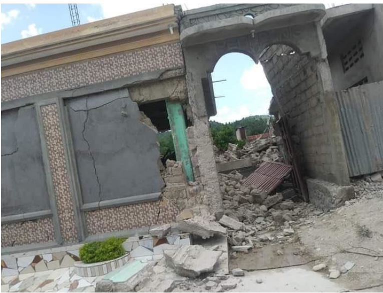
Damage to masonry in the commune of Maniche, Les Cayes, Sud Department (Source: Twitter )
