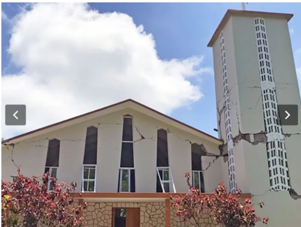
Damage to the church of Saint Anne, in La Sucrerie Henry, commune of Aquin, Sud Department (Source: Mona Lisa Lives Here )
