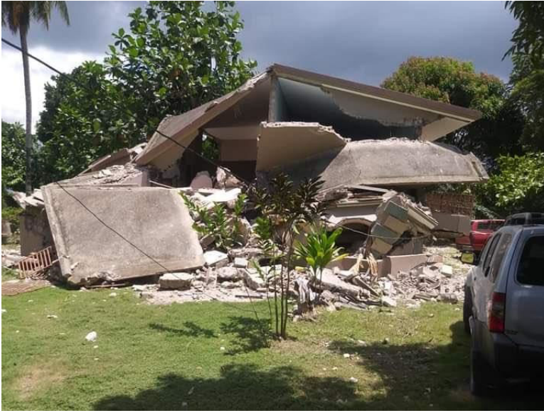
Collapse of a multi-story house in commune of Maniche, Cayes, Sud Department (Source: Twitter )
