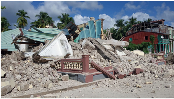
Church of Saint Peter in the commune of Baradères after the 2021 Haiti Earthquake (Source: Twitter )
