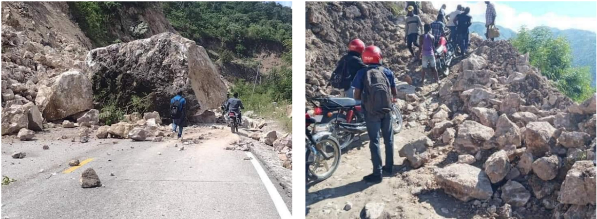
Figure 5.1. Rockslides restrict RN7 (National Route 7) from Les Cayes to Grand'Anse (Source: W10news - Facebook post ).
