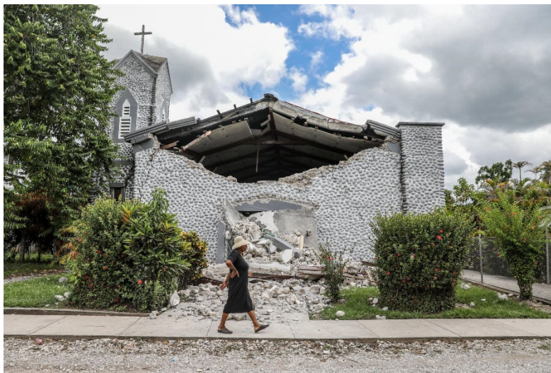
Figure 4.26. View of the damage to the Chapel of Saint Eugene, which is part of the seminary school of the Missionary Oblates of Mary Immaculate in Mazenod, Camp-Perrin (Source: NYTimes ).
