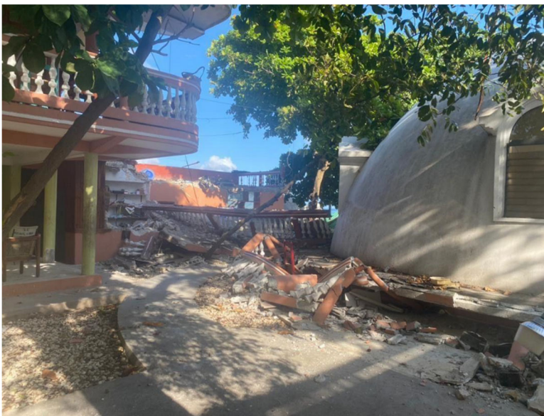
Collapsed Manolo Inn Hotel in Petite Riviere de Nippes (Source:Gefthé Dévilmé, GeoHazard International)
