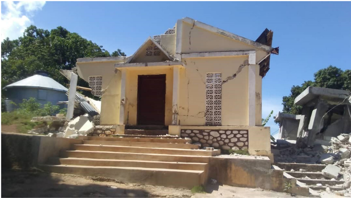
Figure 4.12. Collapse of the Bethesda World Ministries Orphanage in Ave Des Quatre Chemins, Les Cayes (Source: Orphan Grain Train ).
