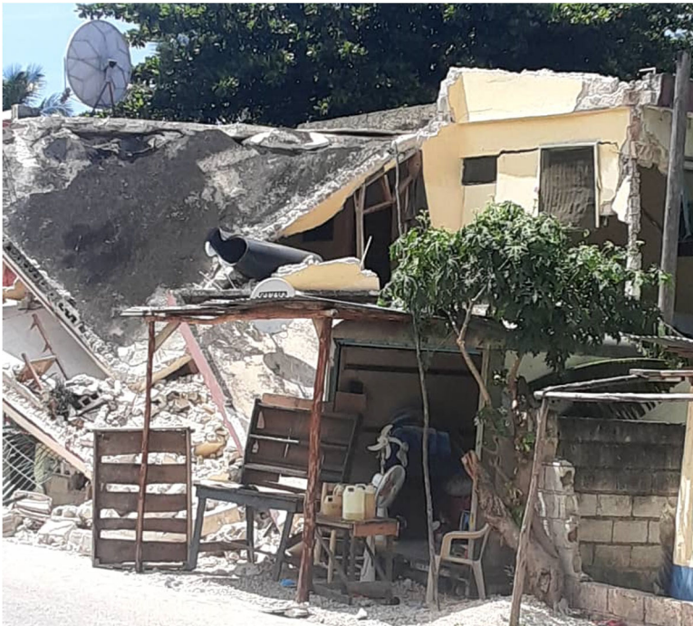
Damage of single-family houses in Petite Riviere de Nippes (Credit: Gefthé Dévilmé, GeoHazards International)
