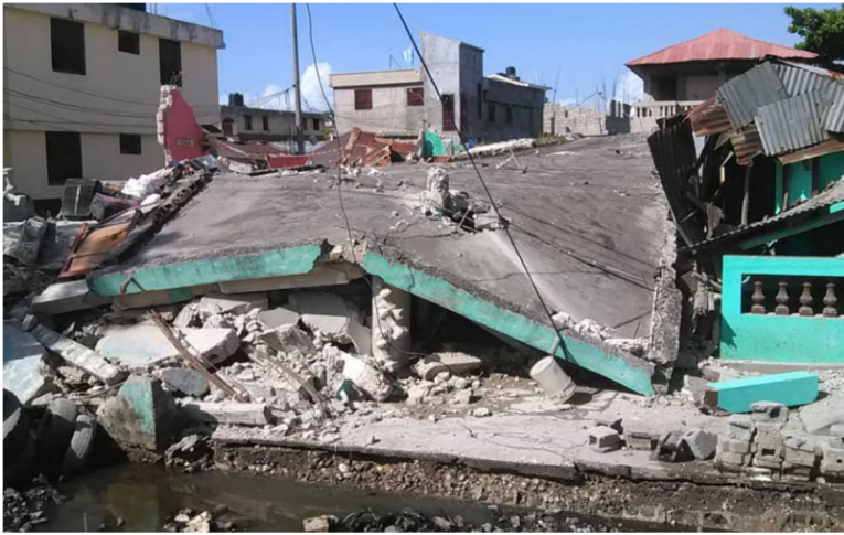
Collapse of concrete building in a residential area in Les Cayes (Source: Twitter )
