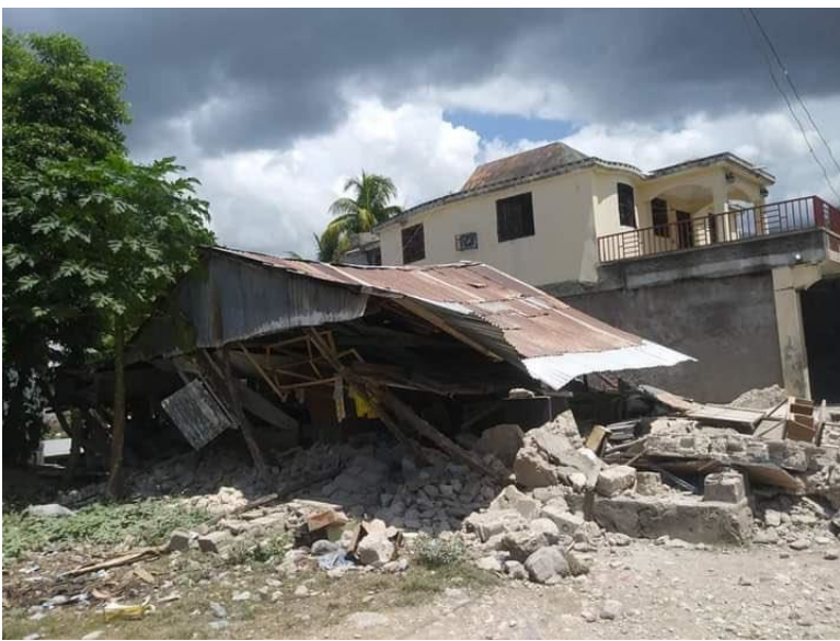
Collapse of wood-framed house in the commune of Maniche, Cayes, Sud Department (Source: Twitter )
