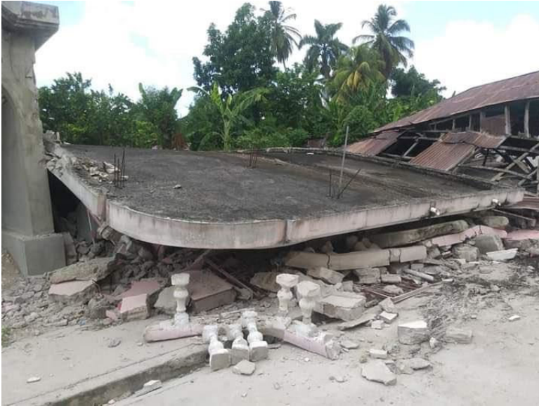
Collapsed masonry home in the commune of Maniche, Cayes, Sud Department (Source: Twitter )
