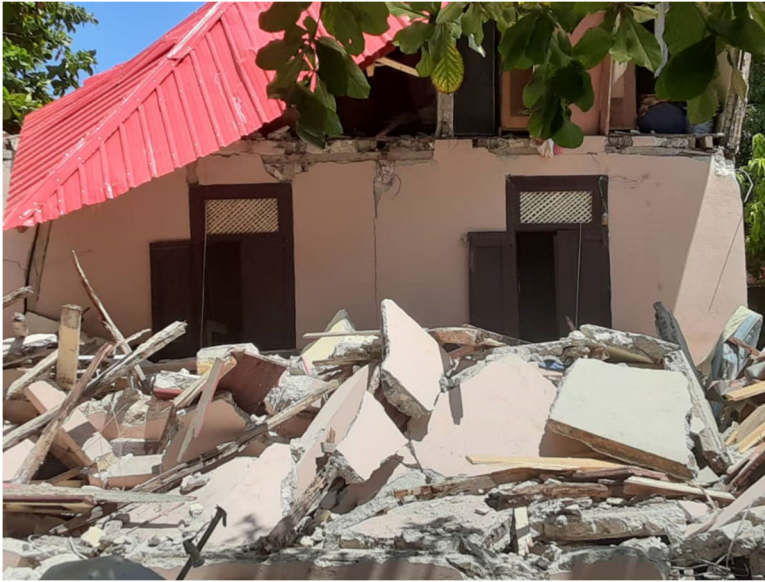
Damage of single-family house in Anse-a-Veau (Credit: Gefthé Dévilmé, GeoHazards International)
