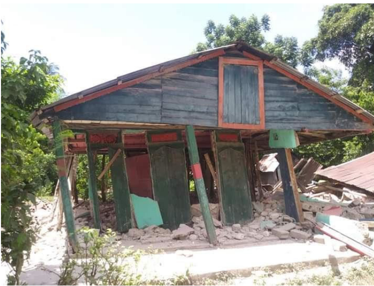
Damage to infill walls in homes of the commune of Maniche, Cayes, Sud Department (Source: Twitter )
