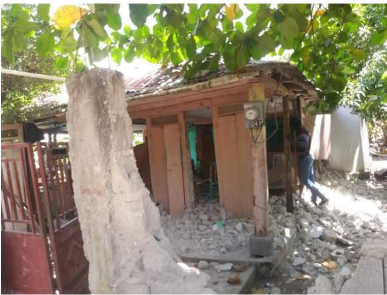
Damage to infill walls in house in commune of Maniche, Cayes, Sud Department (Source: Twitter )
