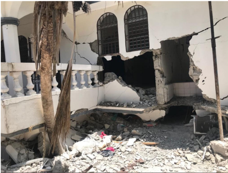
Soft story collapse of concrete building (Source: Twitter )
