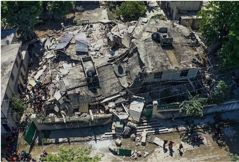
Collapse of a building in Les Cayes (Ralph Tedy Erol/EPA, via Shutterstock, Source: NY Times )
