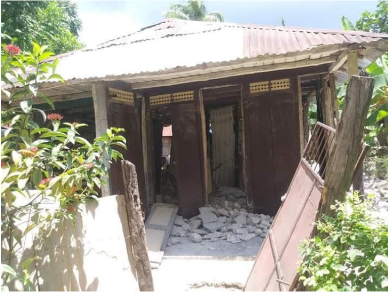
Damage to infill walls in house in commune of Maniche, Cayes, Sud Department (Source: Twitter )
