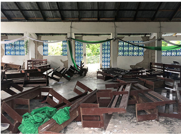
Damage to the church of the Sainte Famille du Toirac, in Toirac, commune of Camp Pérrin (Source: Boston Pilot )
