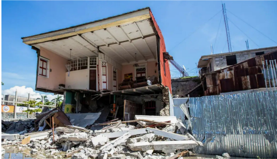
Figure 4.7. Example of an OOP failure in blended stone masonry and timber home in Les Cayes (Note poorly confined masonry construction in the background) (Source: Reuters ).
