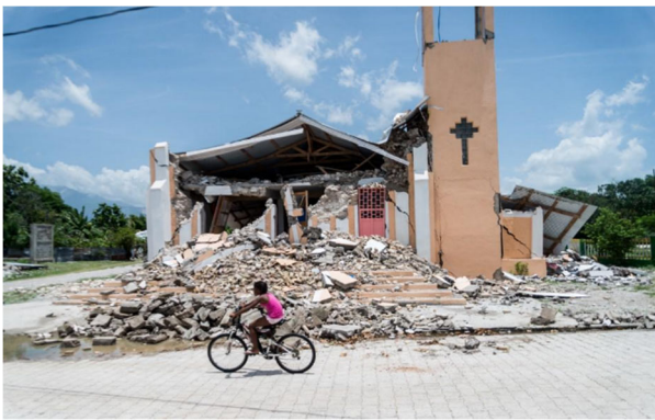
Collapse of the church of Saint Anne in Chardonnières, Sud Department (Source: USA Today )
