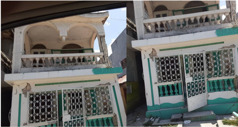
Damage of single-family houses in Petite Riviere de Nippes (Credit: Gefthé Dévilmé, GeoHazards International)
