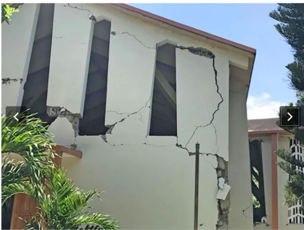
Damage to the church of Saint Anne, in La Sucrerie Henry, commune of Aquin, Sud Department (Source: Mona Lisa Lives Here )
