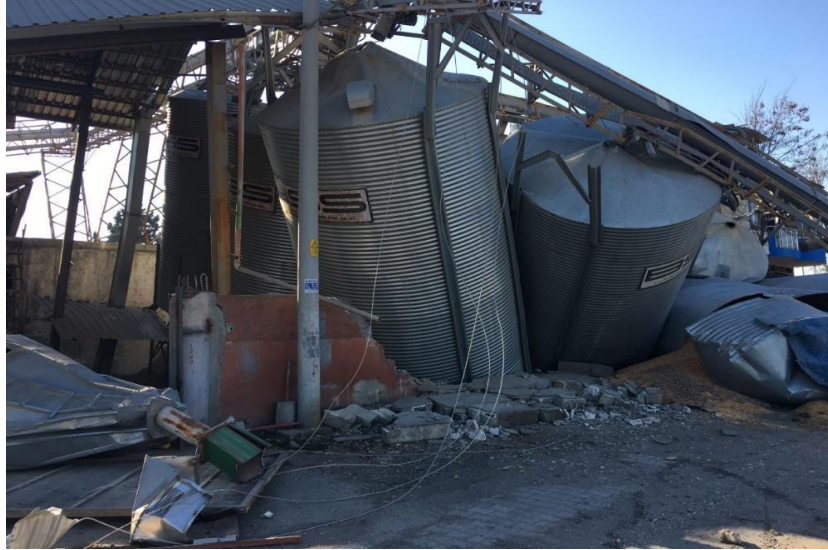
Figure 5.13. Steel storage containers damaged during the earthquake sequence due to failure of roof (Source: Mustafa Kerem Koçkar via LinkedIn ).
