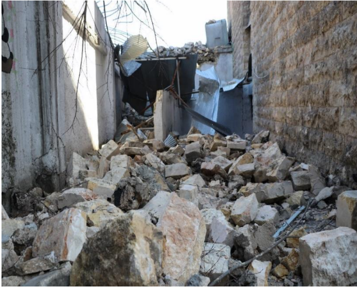
(a) Wreckage of damaged walls.
