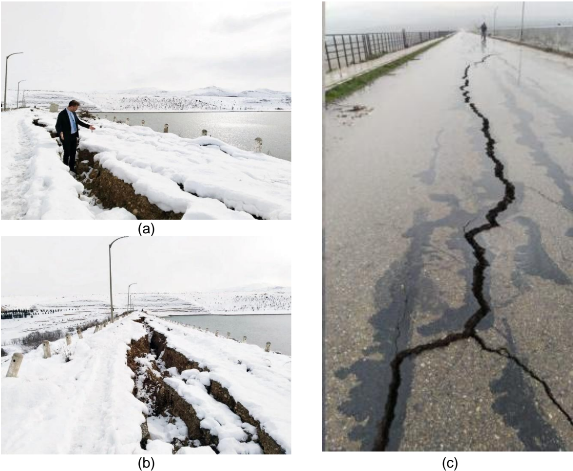
Figure 6.10. (a-b) Sultansuyu Dam with cracks along its central axis (Source: ntv.com ) and (c) longitudinal and transverse cracks in the Afrin dam (Source: Syrian Television via misbar.com ).
