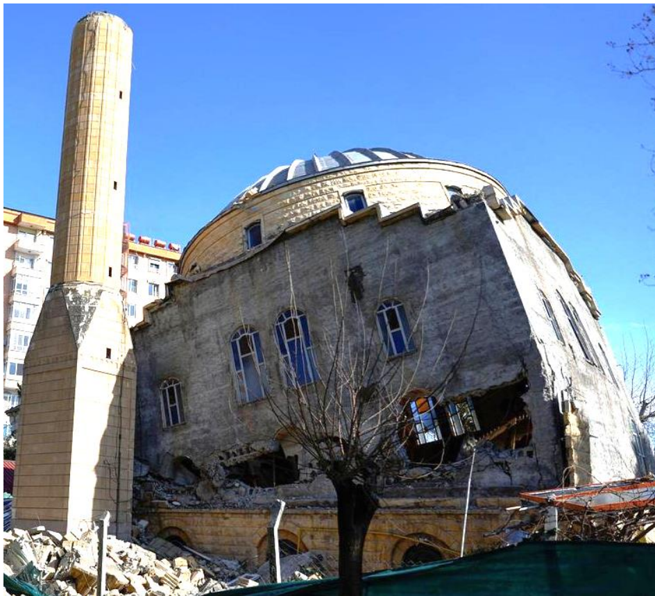
Figure 4.68. Partial collapse of an exterior wall of a mosque in Kahramanmaraş, Türkiye, while the domed roof remained intact (Source: Reuters via the Independent 2023).
