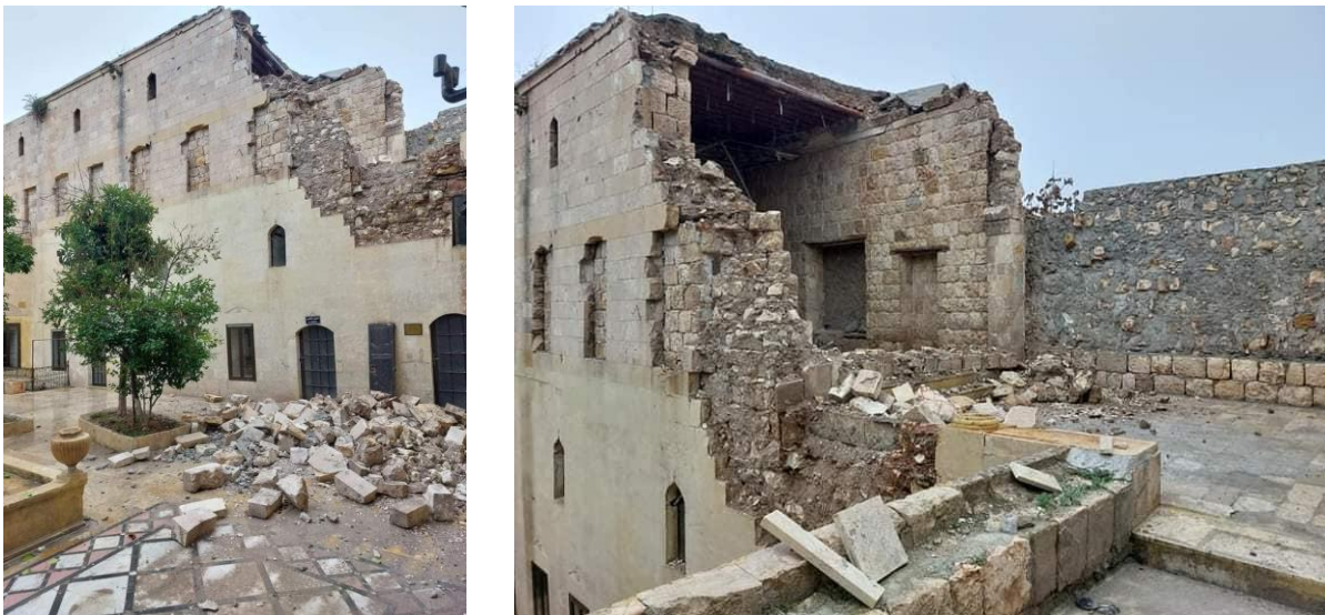
Figure 4.46. Damage at a Cilician Armenian high school of Aleppo, 36.2082°N, 37.1559°E (Source: Massis Post ).
