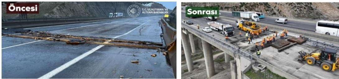
Figure 5.4. Damage and repair work of an expansion joint of a bridge on Adana-Gaziantep Highway (Source: Twitter ).
