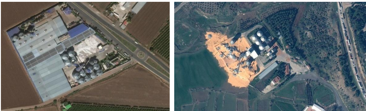
Figure 5.12. Aerial views of the damage of grain silos near Kırıkhan (Left) and near Nurdağı (Right) (Source: CNN ).
