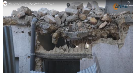
(b) Broken water lines.
