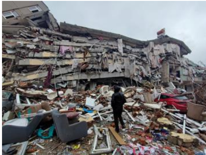
Figure 1.5. Collapsed multi-family residential building in Kahramanmaraş. The photograph illustrates how observed collapse scenarios lead to complete loss of contents and the inability to recover personal possessions (Source: Reuters via CNN ).
