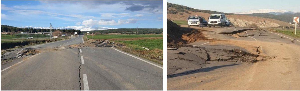
Figure 5.3. Shifting (differential movement) of the roadway near the Tevekkelli village (Source: Veryansin TV ).
