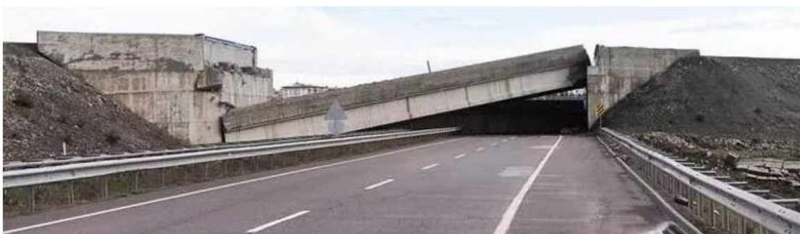
Figure 5.6. Unseating failure of an overpass in Gaziantep Nurdağı (Source: hurriyet.com ).
