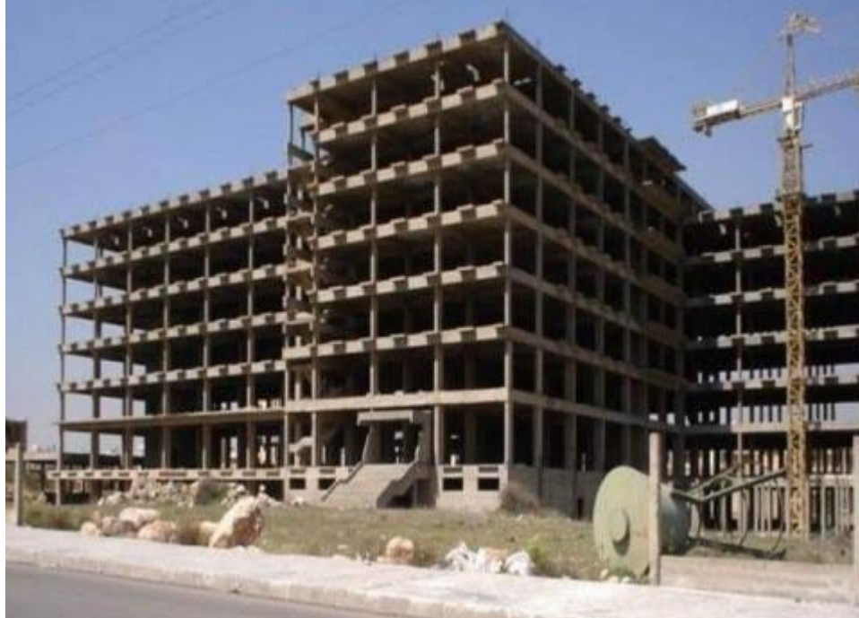
Figure 3.3. The structure of Aleppo military Hospital, Aleppo City - Construction was not compatible with the study (Source: Salah Haj Ismail personal Archive).
