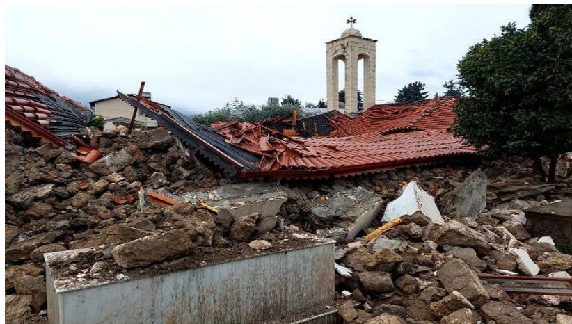
Figure 4.70. Collapsed Mar Yuhanna Orthodox Church in Arsuz where walls were constructed of unreinforced stone masonry (36.4120N 35.8849E) (Source: haber.sat7turk.com 2023).
