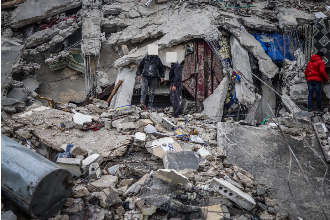
Figure 4.32. Collapsed RC building in Idlib. Notice the poor or absent confinement in columns, small and light longitudinal column bars, and poor concrete quality (Source: Anas Alkharboutli/picture alliance via CNN ).
