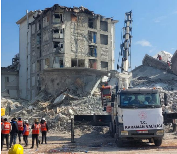
(a) Post-earthquake view from the west of the hospital ( Twitter ), showing minimal structural tie-in between the collapsed and still standing portions of the northwest wings of the hospital.
