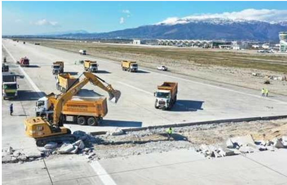
Figure 5.8. Image posted on February 8 1:04 am documenting repair work on the Hatay airport runway (Source: Railynews ).
