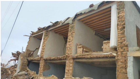
(a) Severely damaged house.
