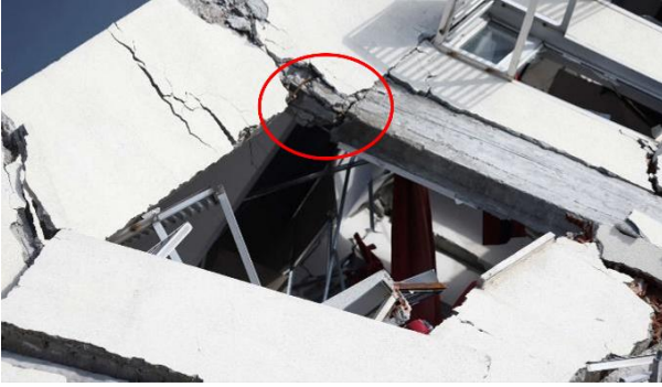
(a) Exposed reinforcing bars in beams and columns with evidence of corrosion, which could limit the ductility of the connection during the earthquake sequence (Reuters via zawya.com ).
