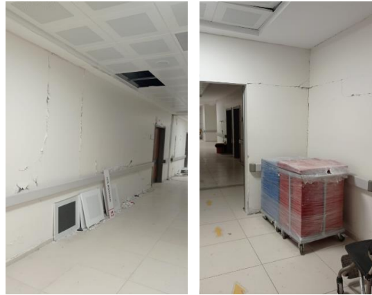
(c) Cracking evident in the covering of multiple gypsum/plaster division walls.
