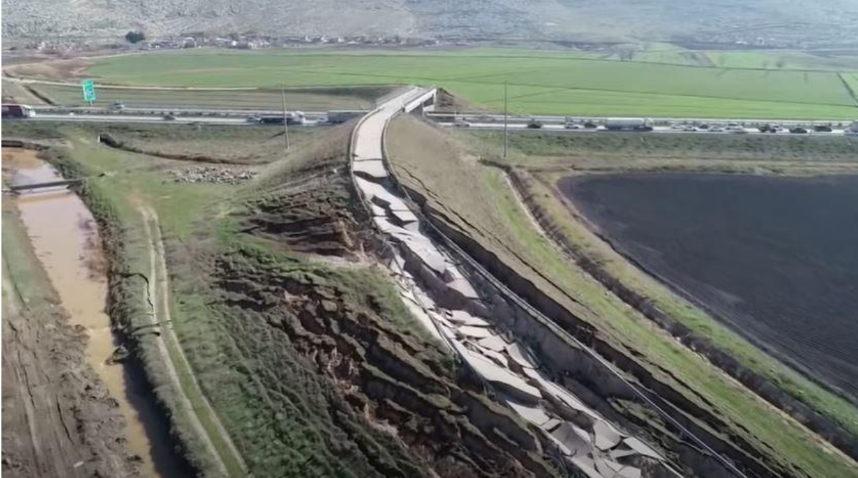
Figure 6.11. Failure of the embankment road in the village of Koseli, which passes over the Adiyaman-Sanlıurfa-Gaziantep Highway in the Adiyaman province (Source: Reuters via Washington Post ).
