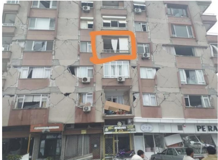
(b) Residents sought help from a rescue team as they were stuck inside the building due to stairwell collapse (Source: Husamettin Dogan via Twitter ).
