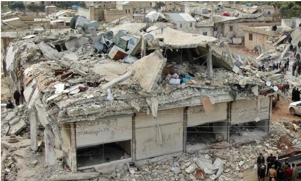
Figure 4.33. Collapsed concrete slab without beams and lacking continuity and integrity reinforcement. Note also the extremely narrow columns in one direction (Source: The Telegraph, 2023b).
