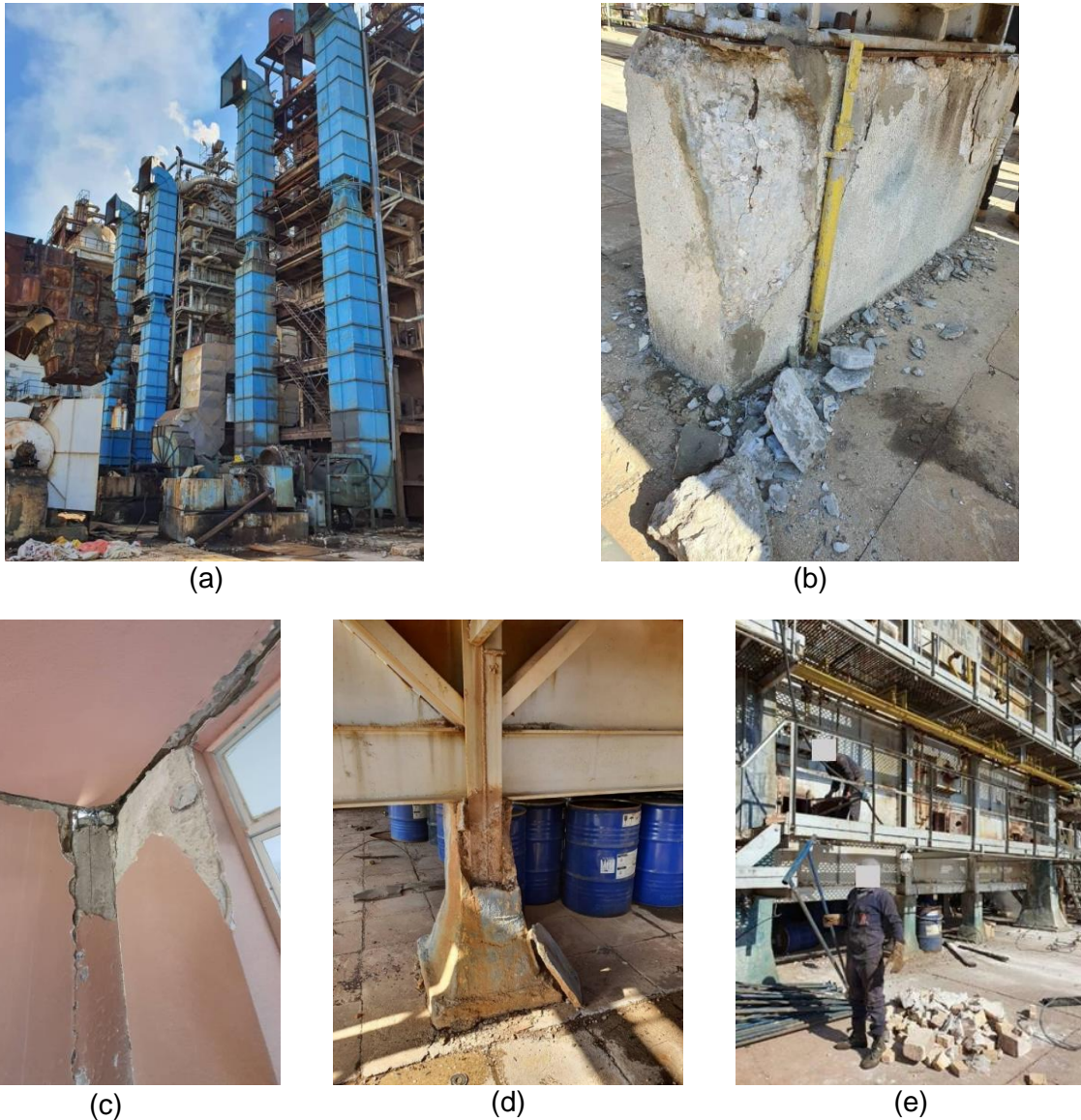
Figure 5.15. Damage of Baniyas Oil Refinery in Syria (Source: Syrian Ministry of Oil and Mineral Resources ).
