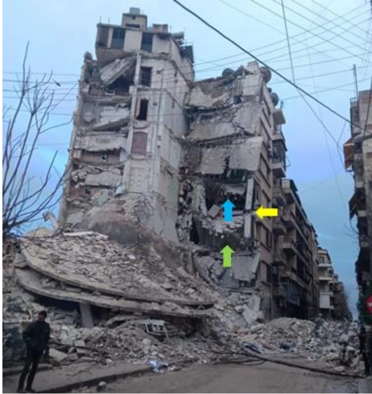
Figure 4.27. A partially collapsed building in Syria. Notice light column reinforcement (yellow arrow), the absence of beams and slab integrity steel (blue arrow), and poor reinforcing bars anchorage (green arrow) (Source: https://yle.fi/a/74-20016582 ).
