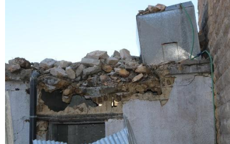
(c) Fallen non-structural component.
