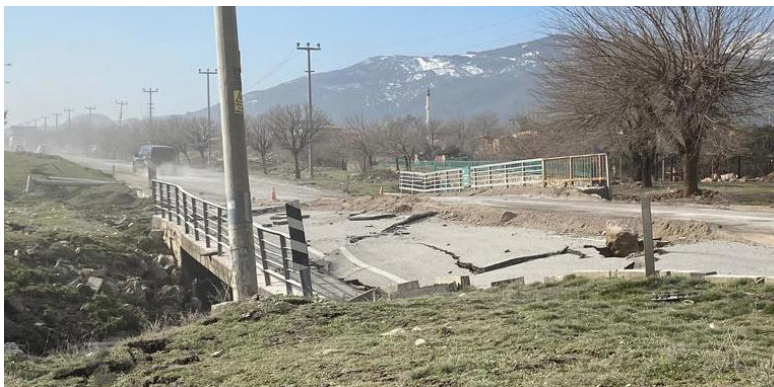
Figure 5.5. Extensive damage at the deck of Şekeroba Bridge (Source: Olay53 ).
