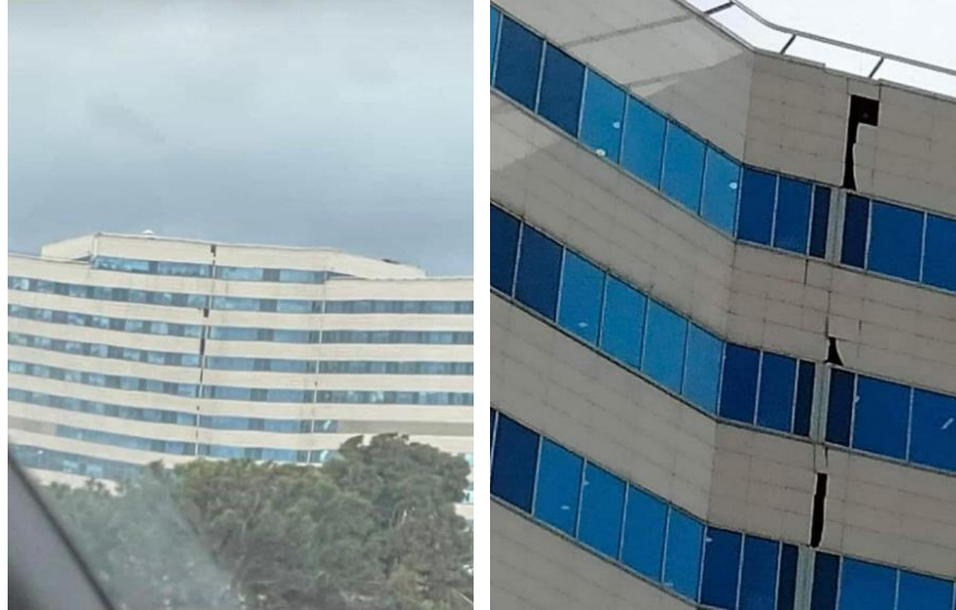
Figure 4.74. Damage to Mersin City Hospital, Türkiye (Source: Twitter ).
