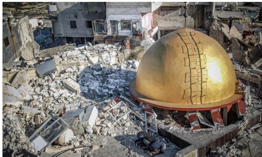
Figure 4.72 Collapsed mosque in Idlib, Northwest Syria (Source: Getty Images via Foreign Policy , 2023). The heavy dome roof appears to have been supported on a long-span roof supported by rectangular reinforced concrete columns with inadequate reinforcement.
