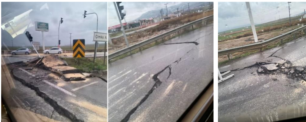
Figure 5.2. Surface failure of roadway (Source: Channel News Asia ).
