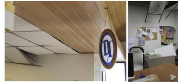
Daily Independent Newspaper office damage [6] Credit: Jessica Weston (AP)
