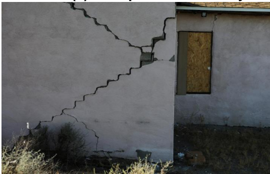
(b) Cracks in exterior walls
