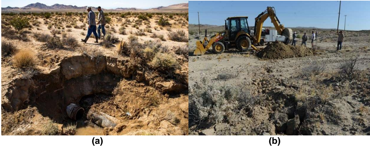
Figure 40. (a) Exploded water pipe reported during the M 6.4 event, consequently forming a crater near Ridgecrest (Source: AP Photo/Etienne Laurent, EPA-EFE 36 ; (b) Crews dealing with a water main that ruptured during the earthquake 37
