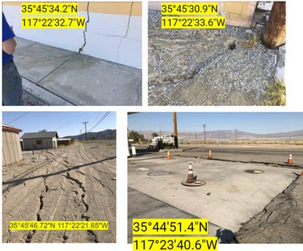
Figure 51. Liquefaction induced lateral spreading and sand boils causing damage to the roadway, and infrastructure in the Trona area (source for all: courtesy of Kenneth Hudson, one of EERI field investigation team members) [clockwise from top left: Esparza restaurant commercial building distance from – closest distance to Searles Lake 0.6 mile; US Post Office Building – closest distance to Searles Lake 1.0 mile; corner of California Street and Argus Avenue; Shell gas station – closest distance to Searles Lake 1.0 mile].
