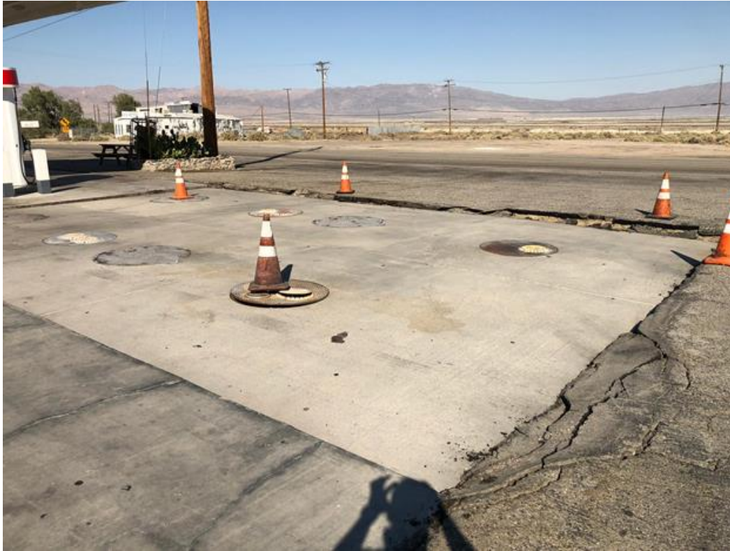
Figure 52. Closer look at ground failure observed at underground storage tank at Shell gas station on Trona Road (Source: courtesy of Kenneth Hudson, one of EERI field investigation team members).
