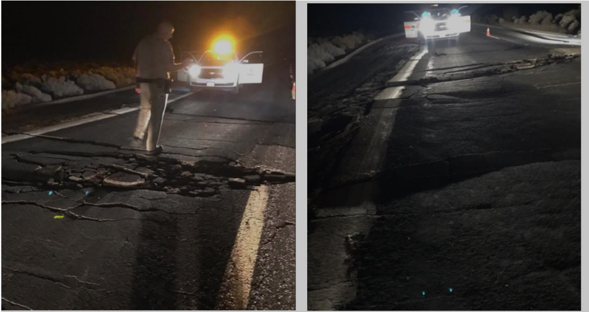
Figure 48. Multiple ground cracks along SR 178 (Source: Caltrans8 Twitter page 56 , taken from the VERT report, Appendix B)
