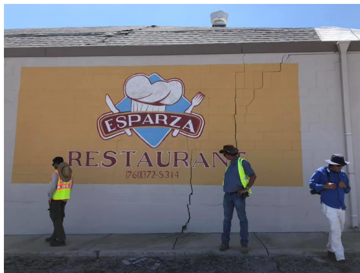
Figure 16. Cracks in masonry walls in Trona following the M 7.1 event (Photo by Christine Goulet, SCEC)
