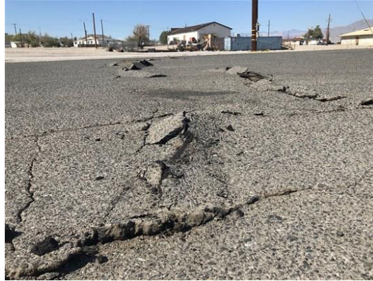
Figure 32. A road in Trona slightly damaged during M 6.4 event (AP Photo/M. Hartman 25 )
