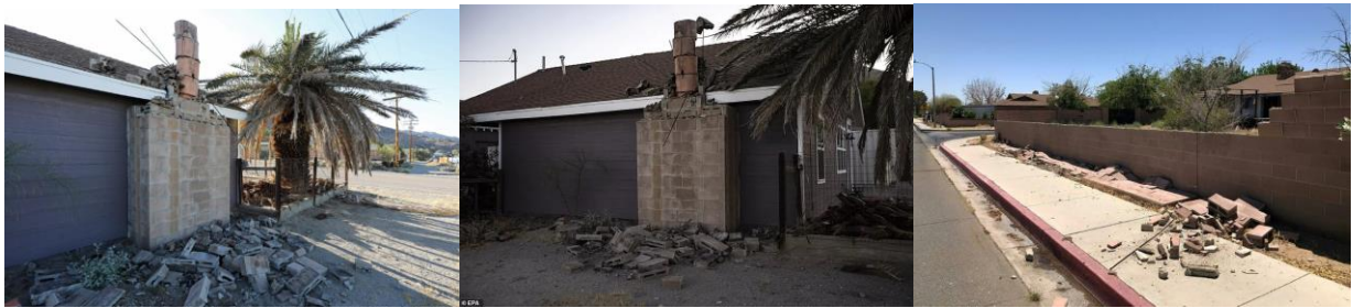
(a) Collapse of a chimney and upper section of a masonry wall
