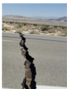
The California Transportation Agency said all repairs have been made and all roads are now open - July 6, 7:30 am [9]
