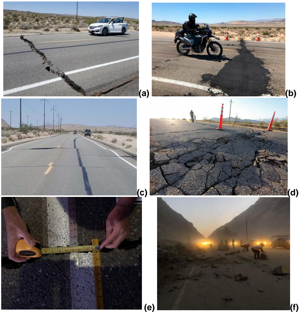
Figure 31. Damage reported in Highway 178 (a) Large crack formed near Trona 20 (b) a motorcyclist rides over a temporarily repaired part of the damaged highway in Ridgecrest one day after the earthquake, demonstrating the rapid response of repair crews; (c) damage reported in Ridgecrest during the M 6.4 event 21 ; (d) surface cracks near Ridgecrest following the M 6.4 event 22 (AP Photo/David McNew) (e) Crack length near Ridgecrest after the July 4th event 23 ; (f) rockslides cause closure of the highway from the M 7.1 event on Friday night; announced clear Saturday at 1 AM by Kern Country 24
