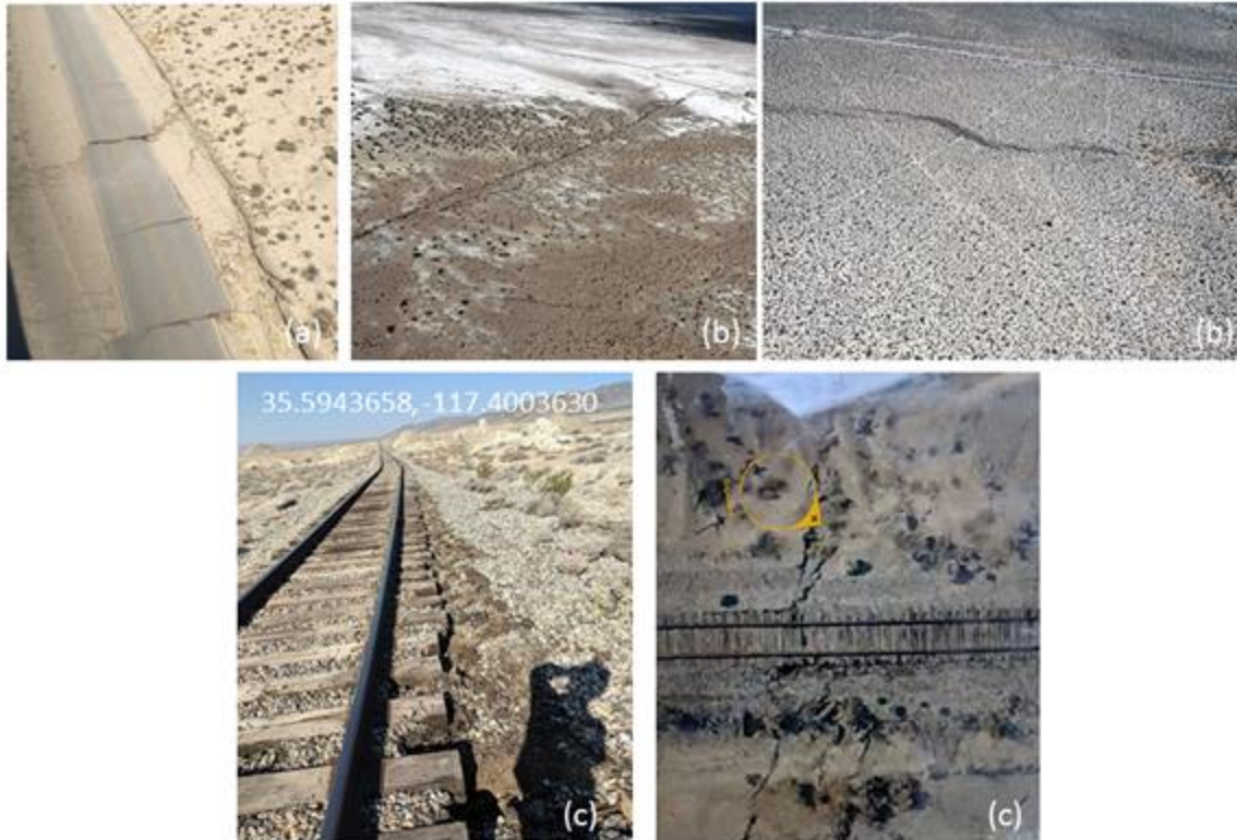
Figure 46. (a) Aerial view of the faulted road on the China Lake NWAS base, about 6.5 feet (248 mm) right lateral (RL) and 3 feet (114 mm) vertical offset 51 , (b) North-West trending fault rupture measuring 6 feet (229 mm) of right-lateral offset on the China Lake NWAS base 52 , and (c) Bent railroad track due to the fault rupture , close to 3 feet (114 mm) of RL offset 53
