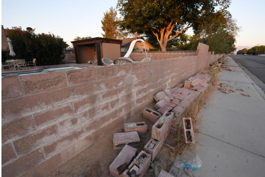
Figure 19. A cinderblock wall partially destroyed in Ridgecrest following the magnitude 7.1 Earthquake (CNN, 2019)
