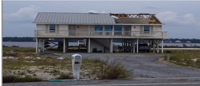
Figure 4.3. Atypical damage to a residential roof in Gulf Shores with loss of roof sheathing.
