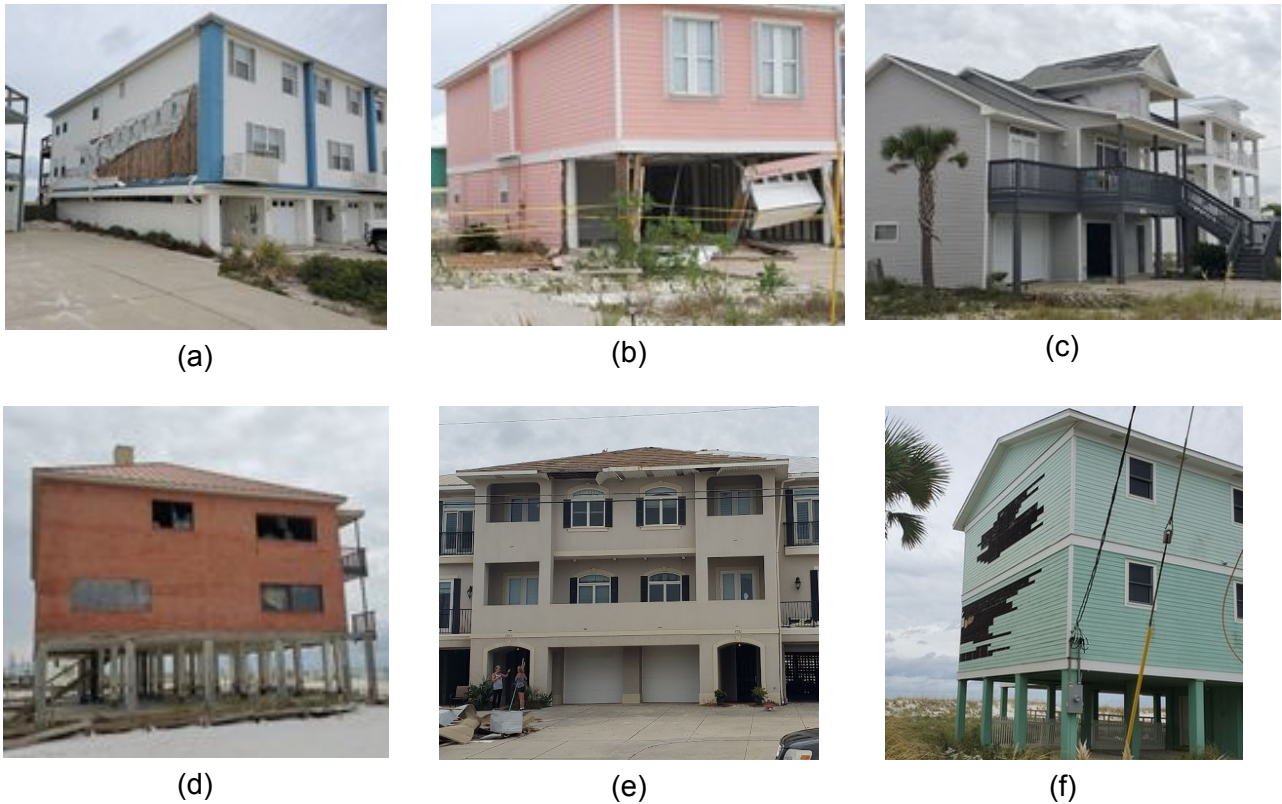
Figure 4.9. Illustrative wind damage on Santa Rosa Island: (a) siding damage, built 1999; (b) collapsed garage, built 2001; (c) roof damage - water intrusion, built 2000; (d) wind-borne debris impacts, year built unknown; (e) metal roof damage, built 2003; (f) siding damage, built 2000.
