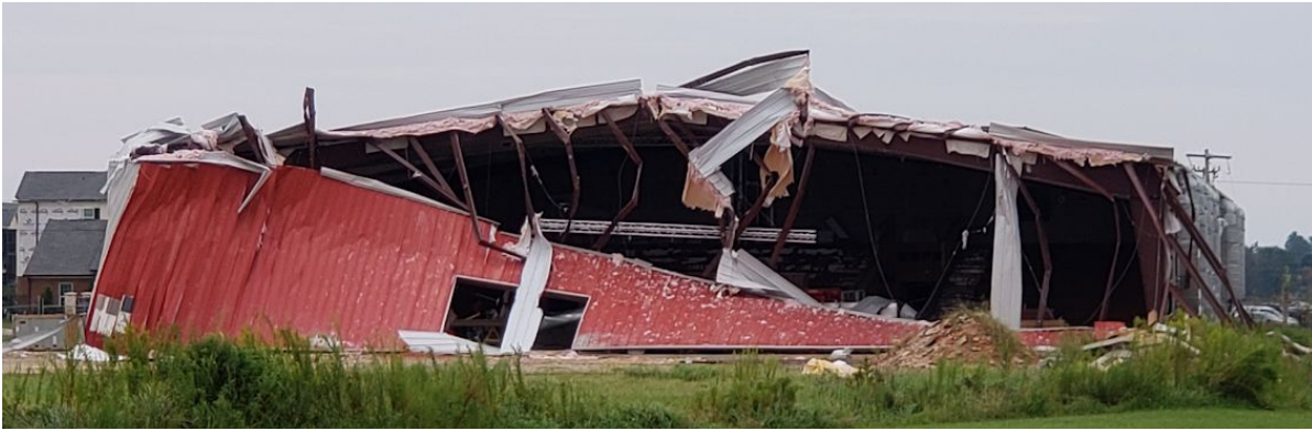
Figure 4.14. Endwall collapse (north-facing wall) of a metal building near Foley, AL (GPS: 30.356369, -87.659019).
