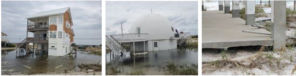
Figure 4.10. Illustrative surge damage on Santa Rosa Island: (left) ground floor damage and siding (wind), built 1992; (middle) ground floor damage, built 1982; (right) scouring damage, year built unknown.
