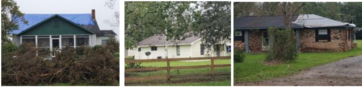
Figure 4.11. Illustrative damage in Elsanor: (left) roof damage, built 1955; (middle) roof damage, year built unknown; (right) roof & siding damage, year built unknown.
