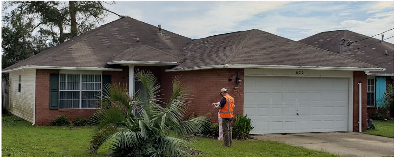
Figure 4.15. Typical shingle loss in a neighborhood of single-family homes in West Pensacola constructed in 2001.
