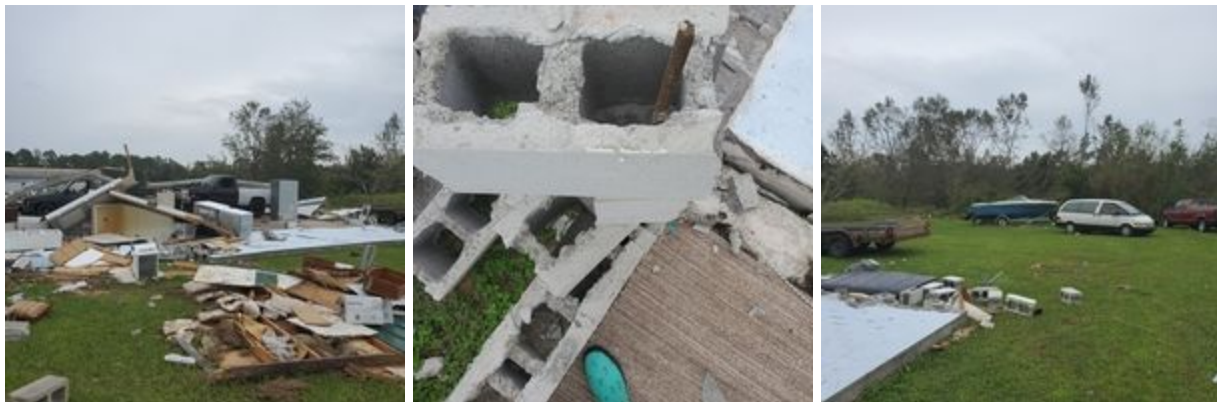
Figure 4.13. An unreinforced masonry block structure in Foley, AL was destroyed.
