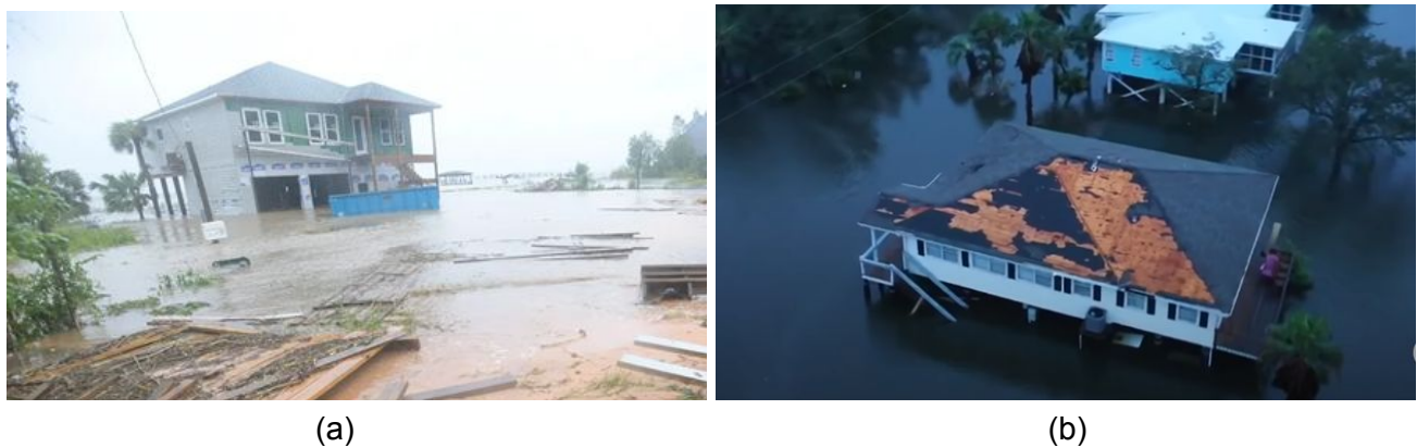
Figure 3.1. Envelope damage in Sally: (a) siding loss on a house in Pensacola, FL; (b) roof cover loss on a house in Gulf Shores, AL. (Sources: (a) www.pnj.com , (b) abcnews.go.com )
