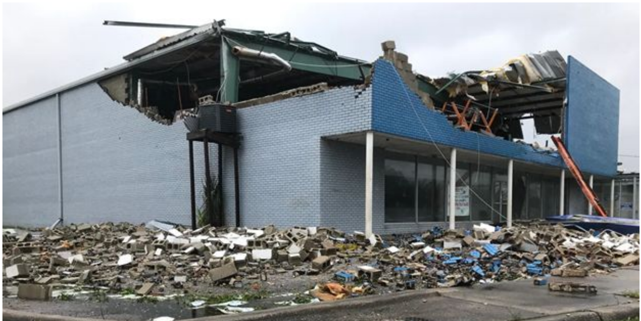
Figure 3.7. Roof damage at a commercial building in Brownsville (West Pensacola) causing failure of infill masonry walls and brick veneer. (Source: www.pnj.com )
