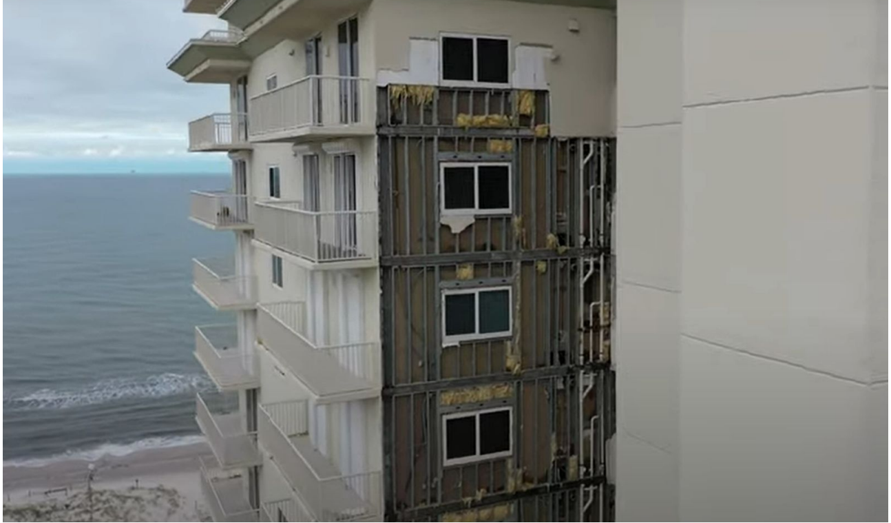
Figure 3.4. Aerial image (by drone) shows loss of curtain wall on high-rise building in Fort Morgan, AL (Source: WXChasing www.youtube.com )
