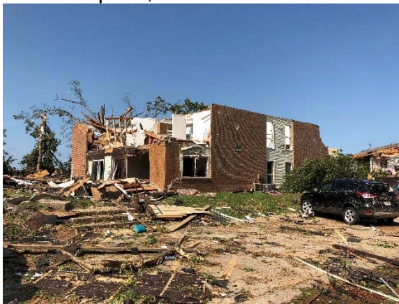
Fig. 18 Entire roof was blown away; wall collapsed; brick veneer fell off; glass was broken.
