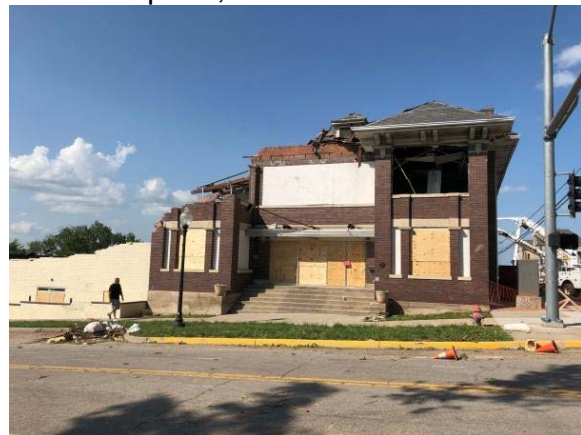
Fig. 19 Partial roof was blown away; wall collapsed; glass was broken.
