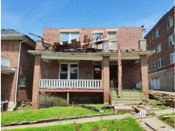
Fig. A9 Entire roof was blown away.
