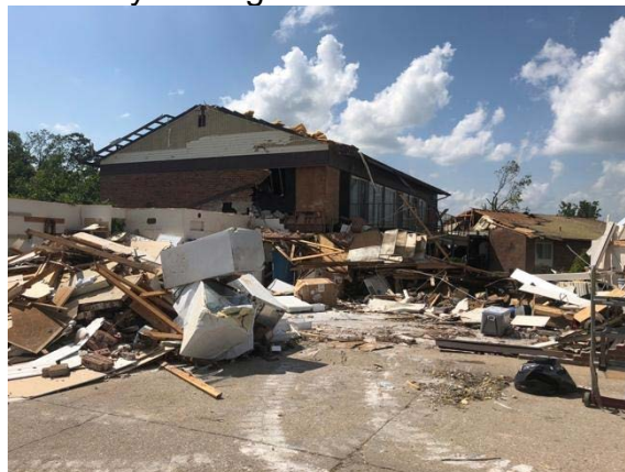
Fig. A15 Partial roof was blown away; wall collapsed; brick veneer fell off.
