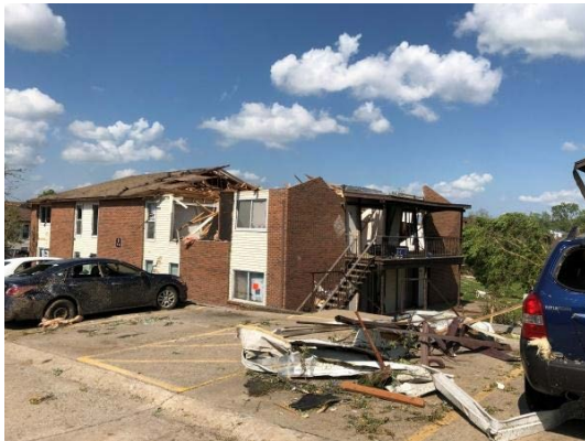
Fig. A11 Partial roof was blown away; brick veneer fell off.
