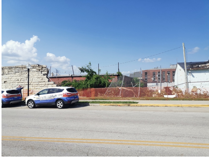
Fig. 10: State Penitentiary wall was blown over by wind.
