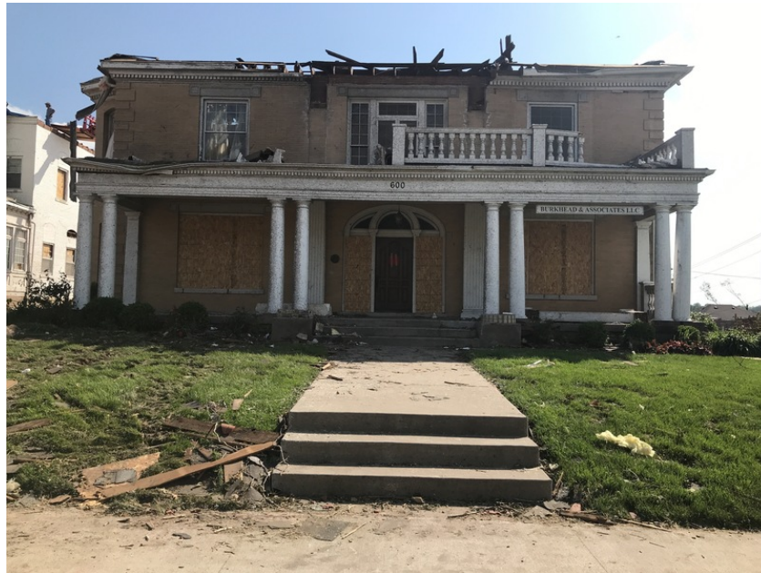
Fig. 9: Historical building that was used as an office. Total roof collapse visible from street.
