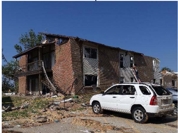
Fig. A6 Partial roof was blown off; brick veneer fell off.
