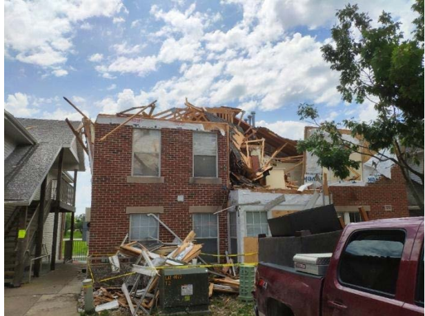
Fig. A10 Entire roof was severely damaged; wall fell off.
