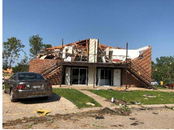
Fig. 17 Partial roof was blown away; wall collapsed; brick veneer fell off.
