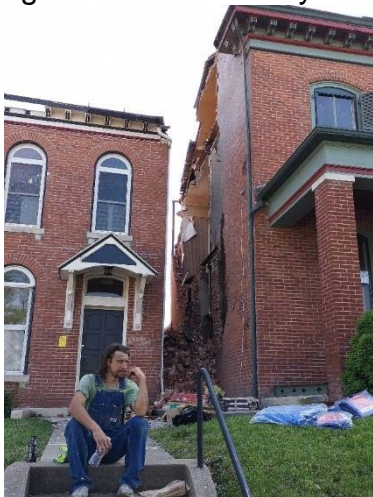
Fig. A7 Side wall collapsed.
