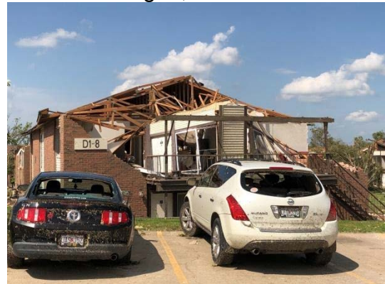
Fig. A12 Partial roof was blown away; wall collapsed; brick veneer fell off.
