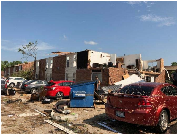
Fig. A1 Entire roof was blown away; wall collapsed; brick veneer fell off.
