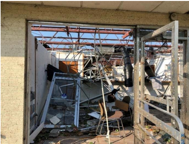
Fig. A5 Entire roof was severely damage; glass door is destroyed.
