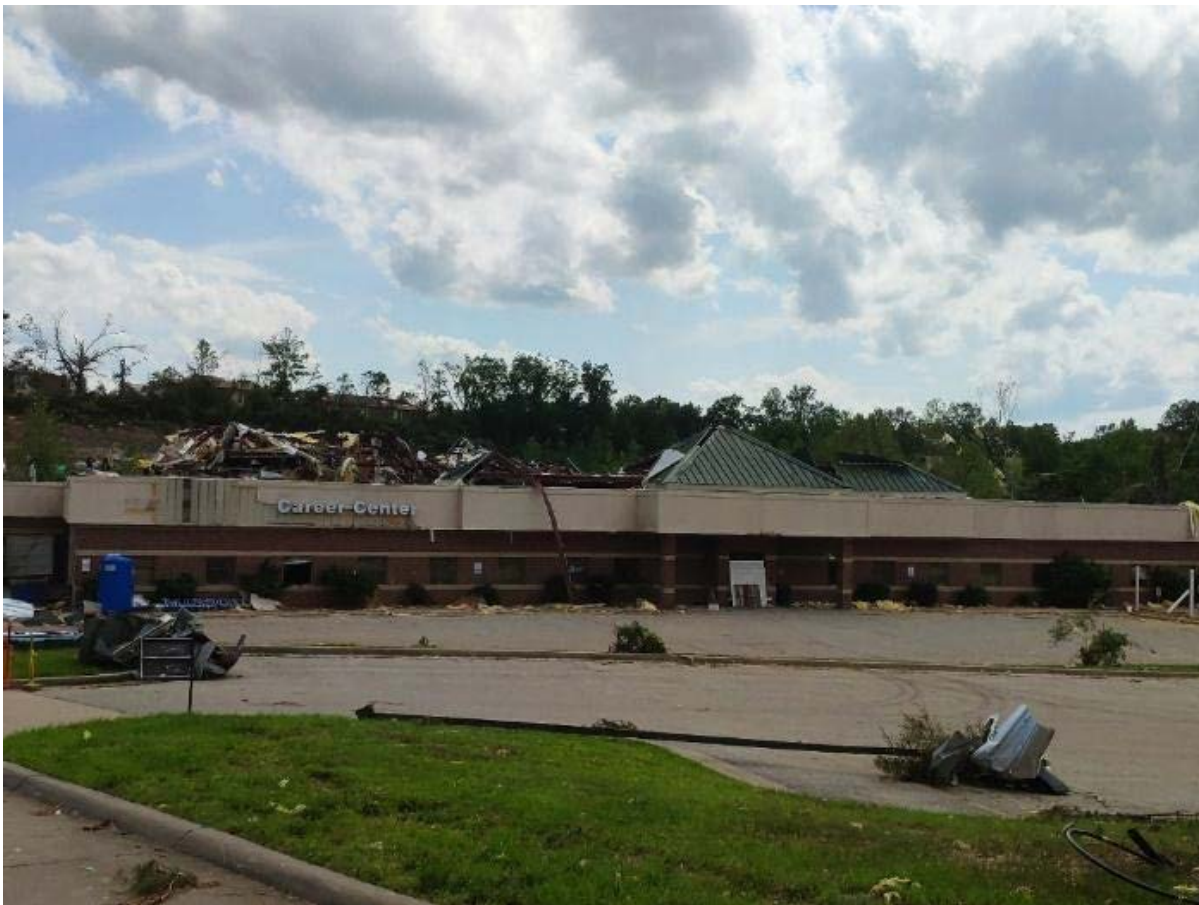
Fig. A13 Steel roof was severely damaged.
