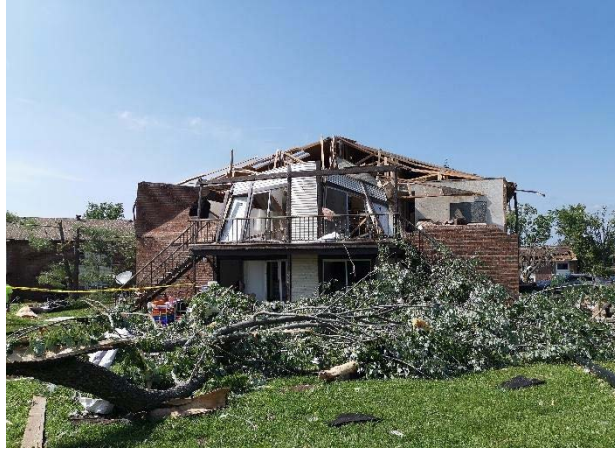
Fig. A4 Partial roof truss was severely; wall collapsed.
