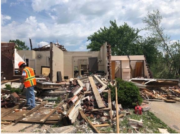
Fig. 16 Entire roof was blown away; wall collapsed; brick veneer fell off.
