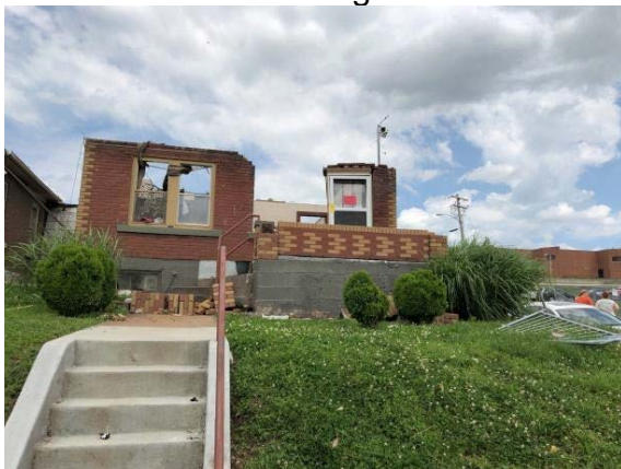
Fig. A14 Entire roof was blown away; wall collapsed; brick veneer fell off.
