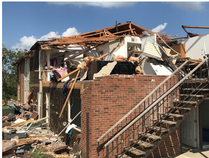
Fig. 8: Multi-family residence with total destruction of the second floor apartment.
