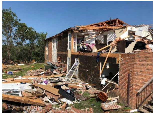
Fig. A2 Partial roof was blown away; wall collapsed; brick veneer fell off.
