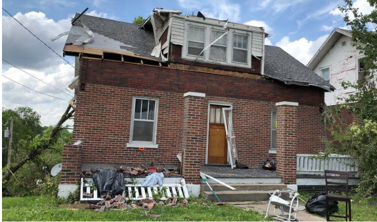
Fig. 7: Typical single-family residence with damage to windows and the roof.
