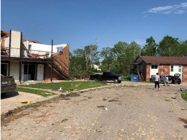
Fig. A3 Partial roof was blown away; wall fell off.
