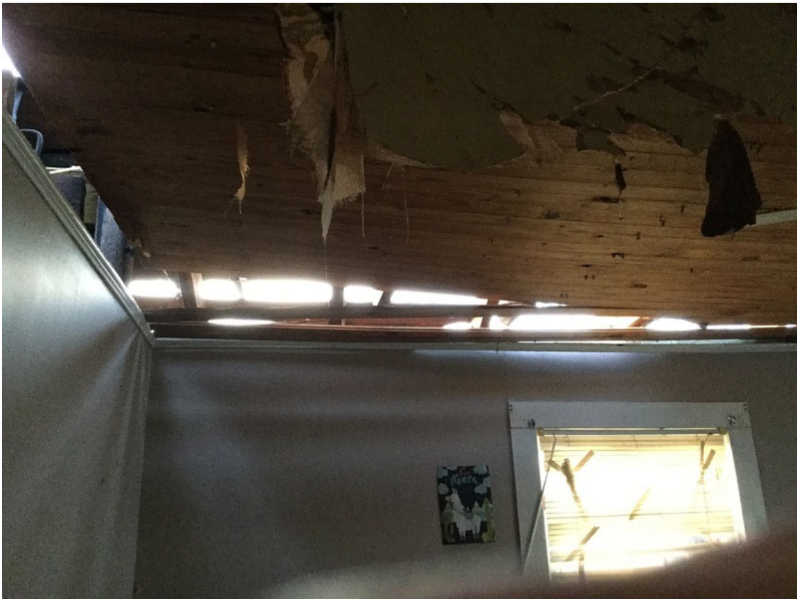
Figure 15. Multi-family residential structure with failure of the roof structure on the west-facing slope of the exterior hip roof, and partial uplift of the ceiling joists as viewed from inside the structure. The additional dead weight of the roof from the wood plank ceilings and wood plank roof diaphragm may have prevented complete lift-off of the roof structure.
