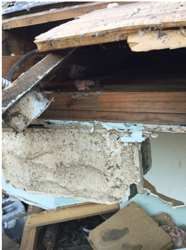
Figure 13. Roof-to-wall connection at the Wetumpka Senior Center, showing wood top plate anchored to grouted CMU block with \frac{1}{2} -inch anchor bolt. Lack of reinforcement in the CMU block wall allowed the grouted cell to easily separate from the rest of the wall structure.
