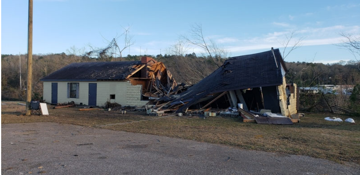
Figure 16. Tree damage (removed before photo was taken) to a facility nearby the Wetumpka Senior Center.
