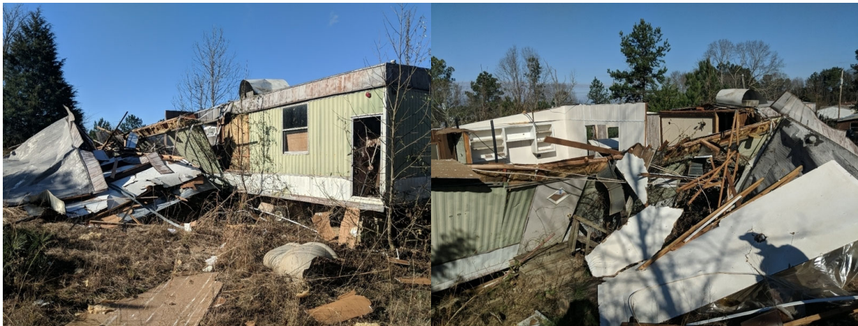
Figure 23. Single-wide mobile home that lost the majority of its roof.
