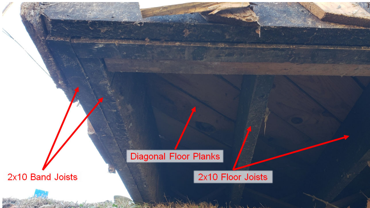
Figure 9. Looking upward at the floor structure of the First Presbyterian Church east wing after it had been shifted off the masonry stem wall on which it originally rested.
