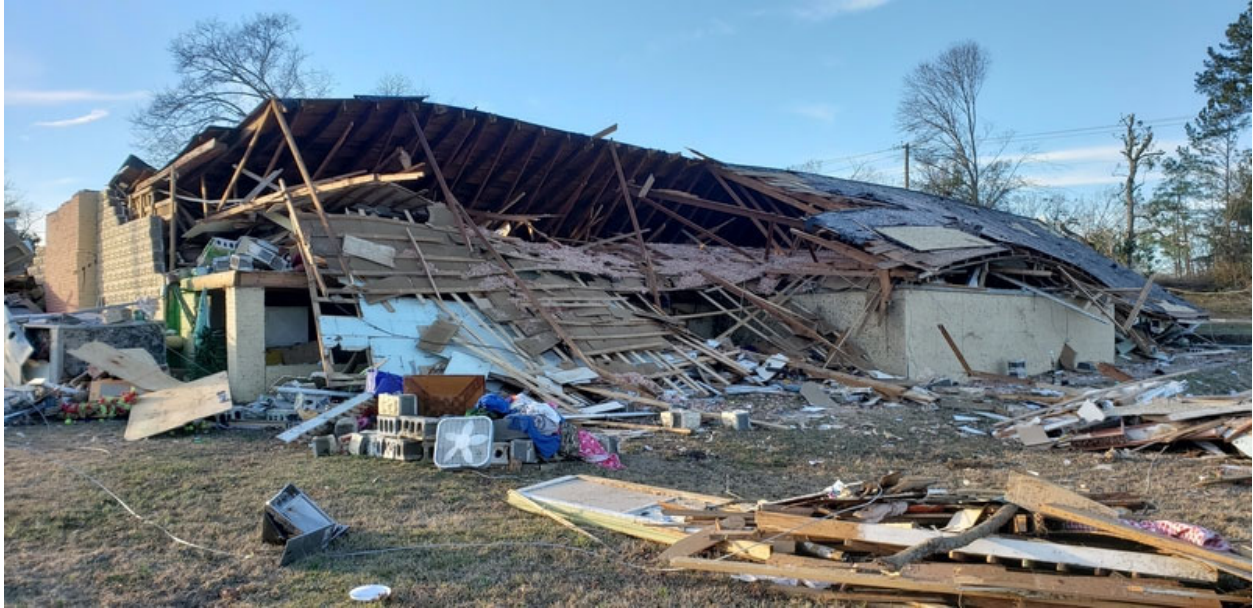
Figure 12. View from the back of the building looking northwest showing the collapsed, unreinforced CMU block walls and damage to roof structure.
