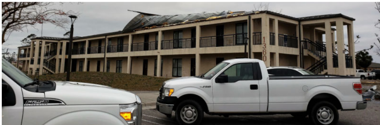
Figure 27. New roof of a barracks peeled back due to tornado winds on the Tyndall AFB (Source: National Weather Service, Tallahassee, FL WFO)
