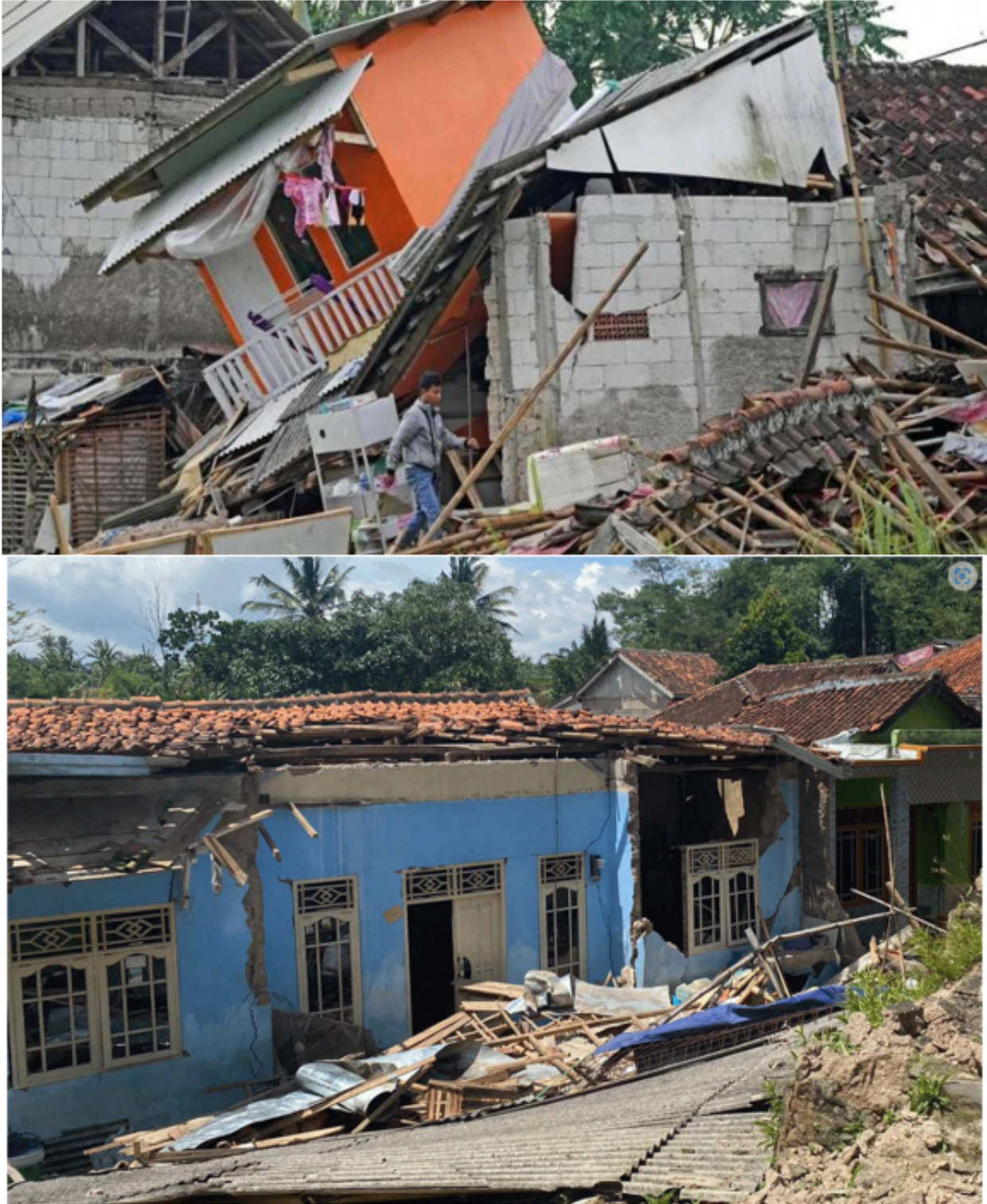
Figure 4.3 – Damage to masonry and concrete brick infills (Project Hope, 2022; Nugraha and Firdaus, 2022).
