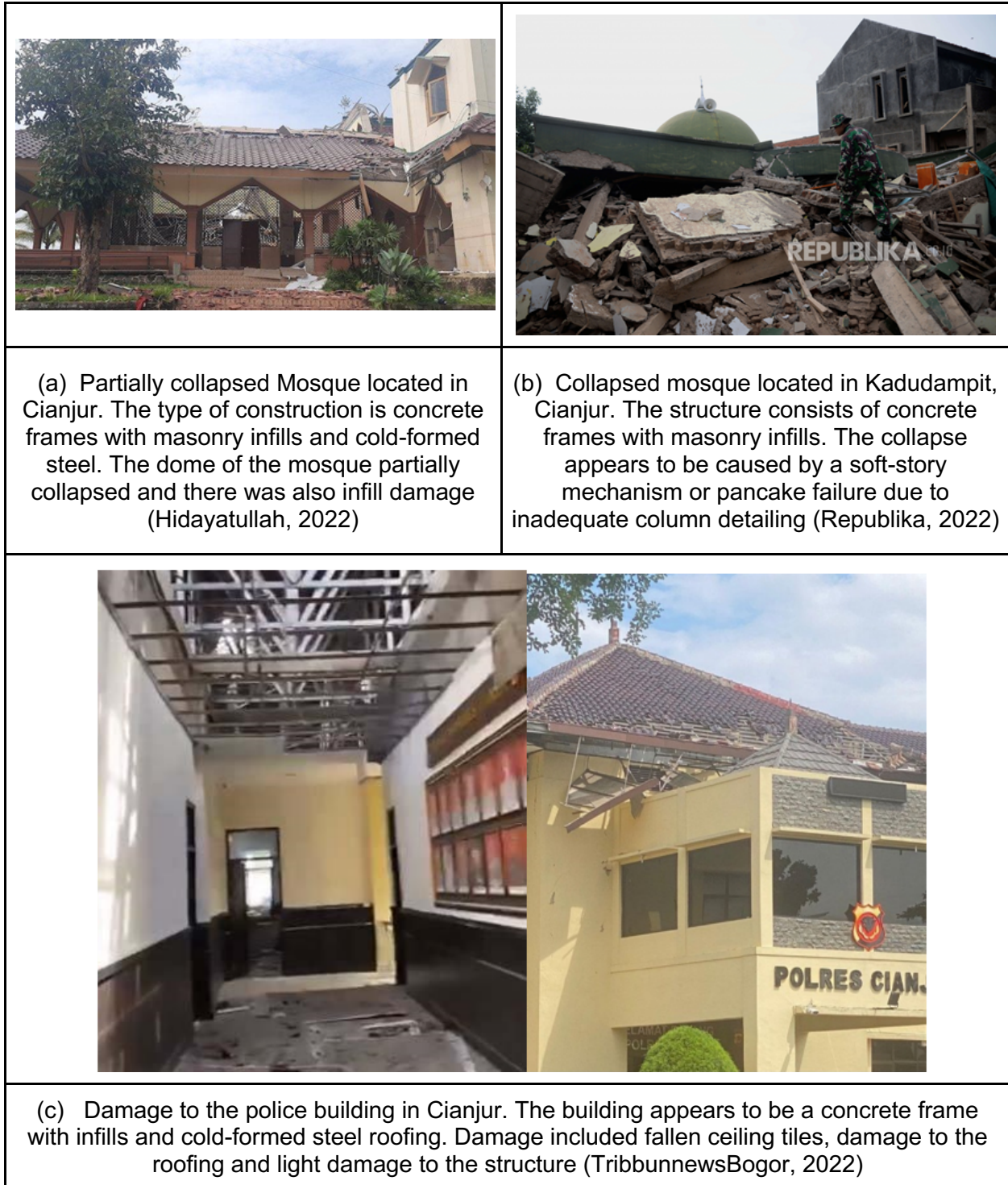
Figure 4.7 – Damage to religious and government buildings.
