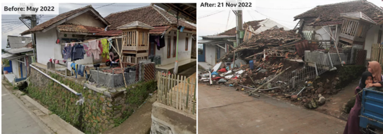
Figure 4.5 – Before and After Picture of Damaged House in Nyalindung Village, Cianjur Region, West Java Province (BBC, 2022a).
