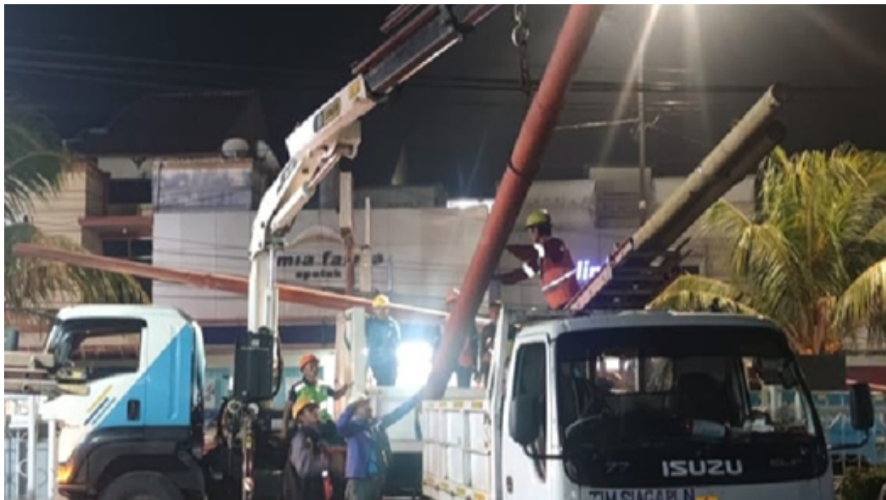
Figure 5.1 Perusahaan Listrik Negara (PLN) officials are working to restore the power grid at the Cianjur earthquake disaster site (Budianto 2022).
