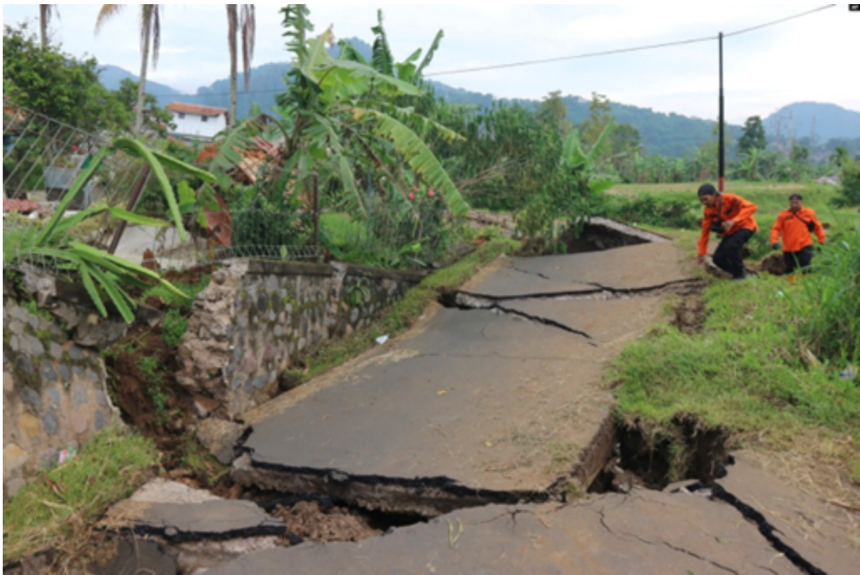
Figure 5.2 Severe road damage caused by the West Java earthquake (VOA News, 2022).
