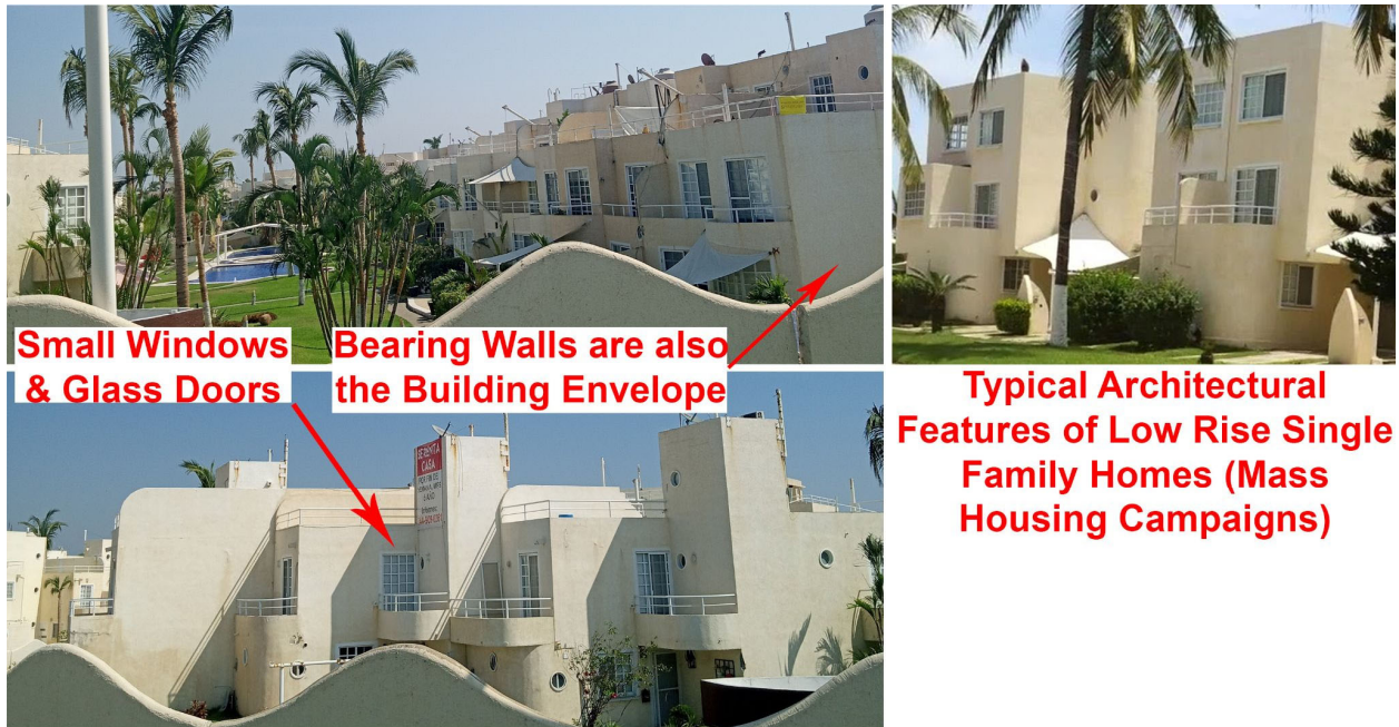
Figure 4.2.2. Minimum damage to building envelope and components and cladding of single-family homes in the Barra Vieja area; (left) after Hurricane Otis (Source: FAST); (right) before Hurricane Otis showing typical architectural features (Source: Google Street View).
