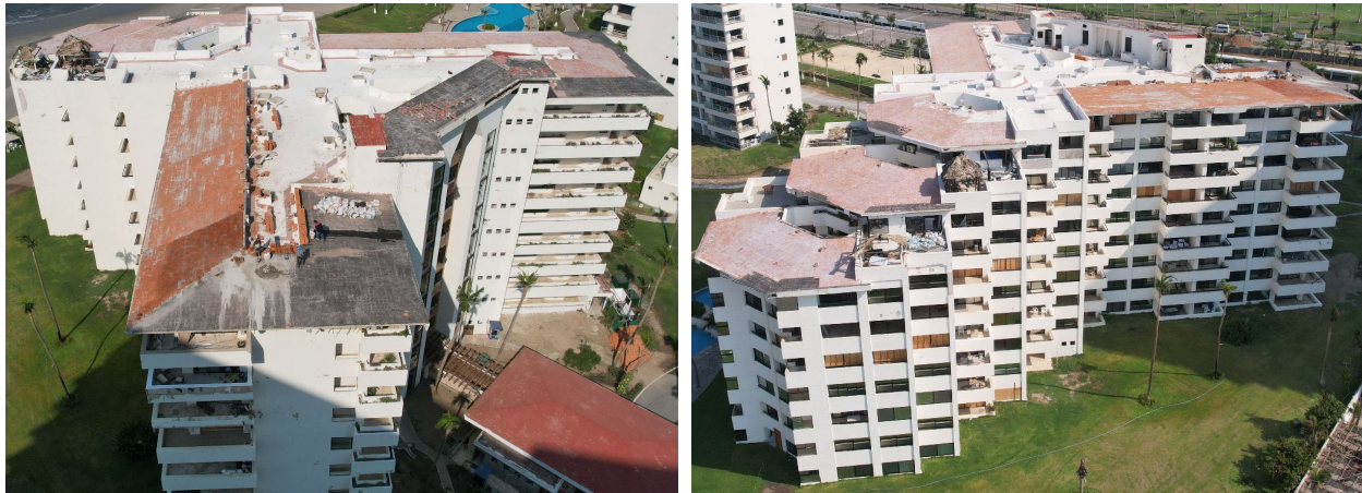
Figure 4.1.9. Roof cover (Flat Clay Roofing Tile) damage at Torre Uno Condominio in Cluster 12 (Source: FAST).
