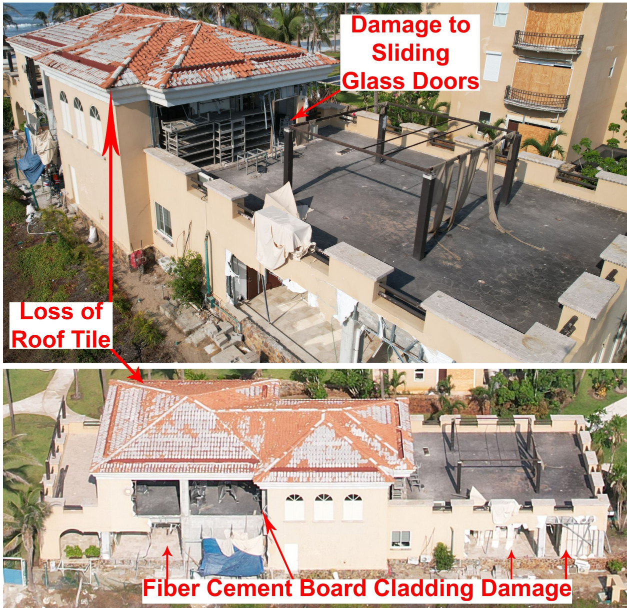
Figure 4.2.1. Damage to building envelope and components and cladding of accessory building (Source: FAST).
