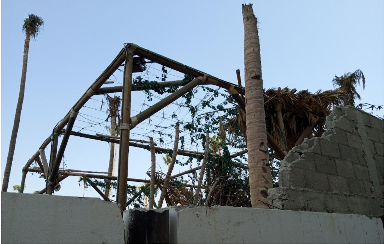
Figure 4.4.3. Out-of-plane damage to masonry wall (tie element on top of black column sheared off completely) and damage to a palapas, a non-engineered wood structure with palm thatched roof (Source: FAST).
