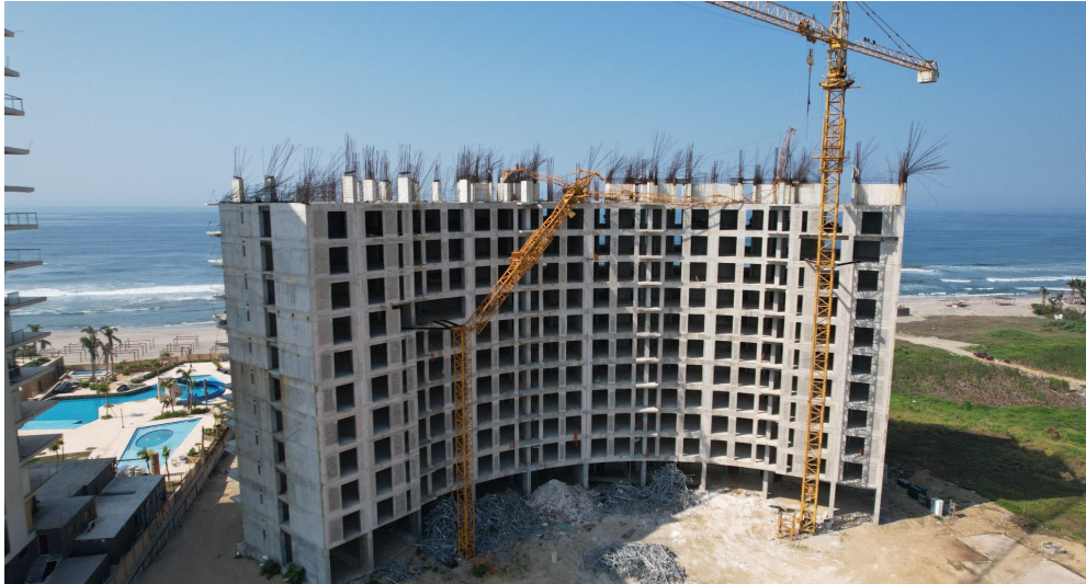
Figure 4.4.1. A tower crane collapsed onto a building under construction (Source: FAST).
