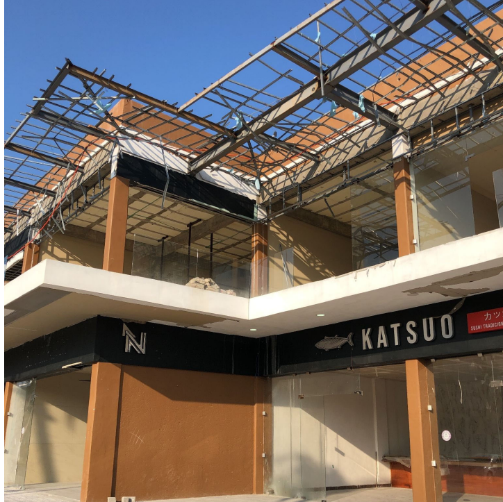
Figure 4.3.3. Damage to Centro Commercial Harbour (Source: FAST)
