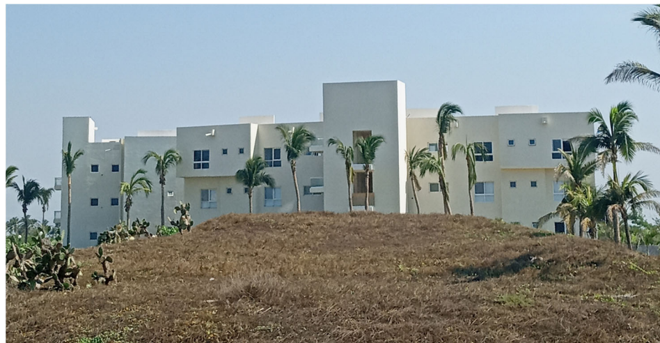
Figure 4.2.3. Examples of INFONAVIT-style construction utilizing reinforced concrete bearing walls as both the LFRS and the building envelope. Both the top and bottom images are representative of multi-family complexes just south of the airport (Source: FAST).
