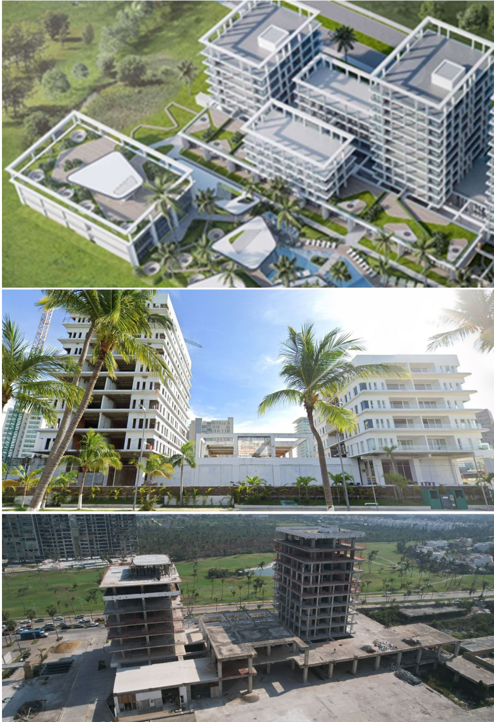
Figure 4.1.10. Maroa (Cluster 11) loss of wall cladding and building envelope; (top) rendering (Source: https://maroadiamante.mx/ ); (middle) before Hurricane Otis on August 2021 view of the NE elevation (Source: Google Street View); (bottom) after hurricane Otis view of the SW elevation, after removal of damaged elements (Source: FAST).
