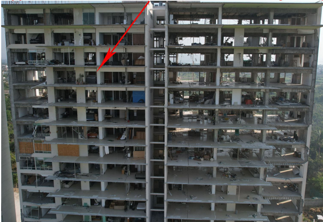
Figure 4.1.12. Damage to Building Contents at Condominio Laguna in Cluster 11, fairway view (Source: FAST).
