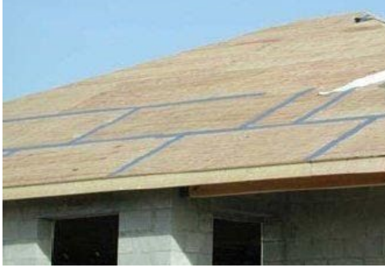
Figure 2.1.1. Peel and stick membrane over joints in the roof sheathing. (Source: IBHS )
